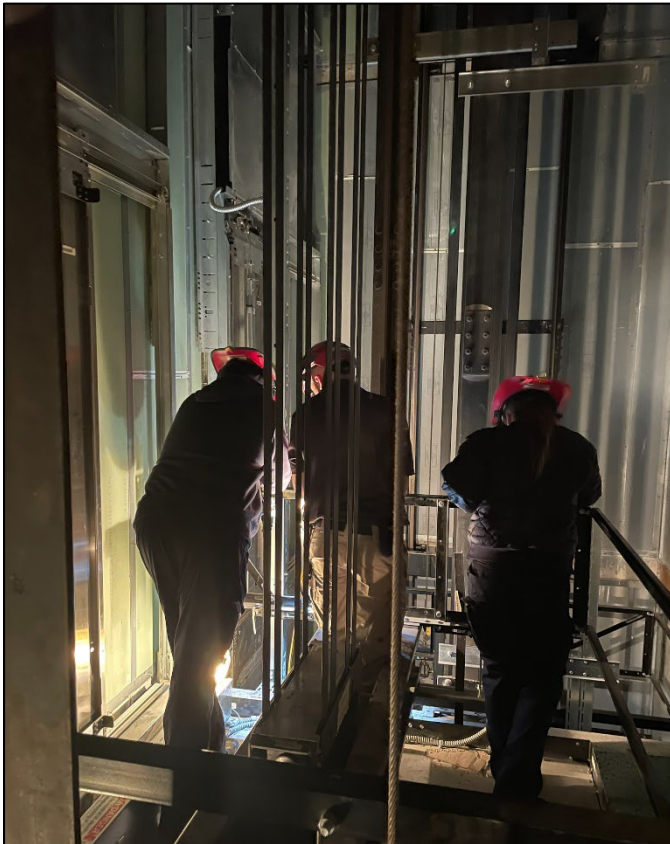
(above) January 2023 - Elevator training.
