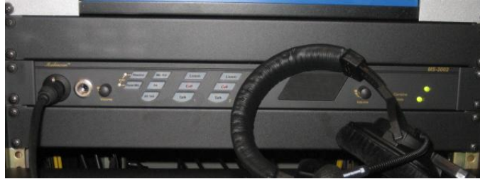
• Intercom Main Station
