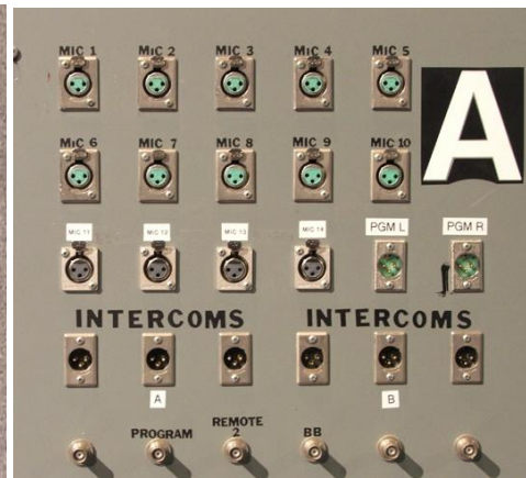
Junction Box (A)
