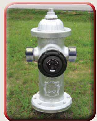
Hydrant Secured with (2) Knox SecureCaps and (1) Knox StorzGuard
