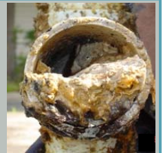
Sewer pipe clogged with grease
