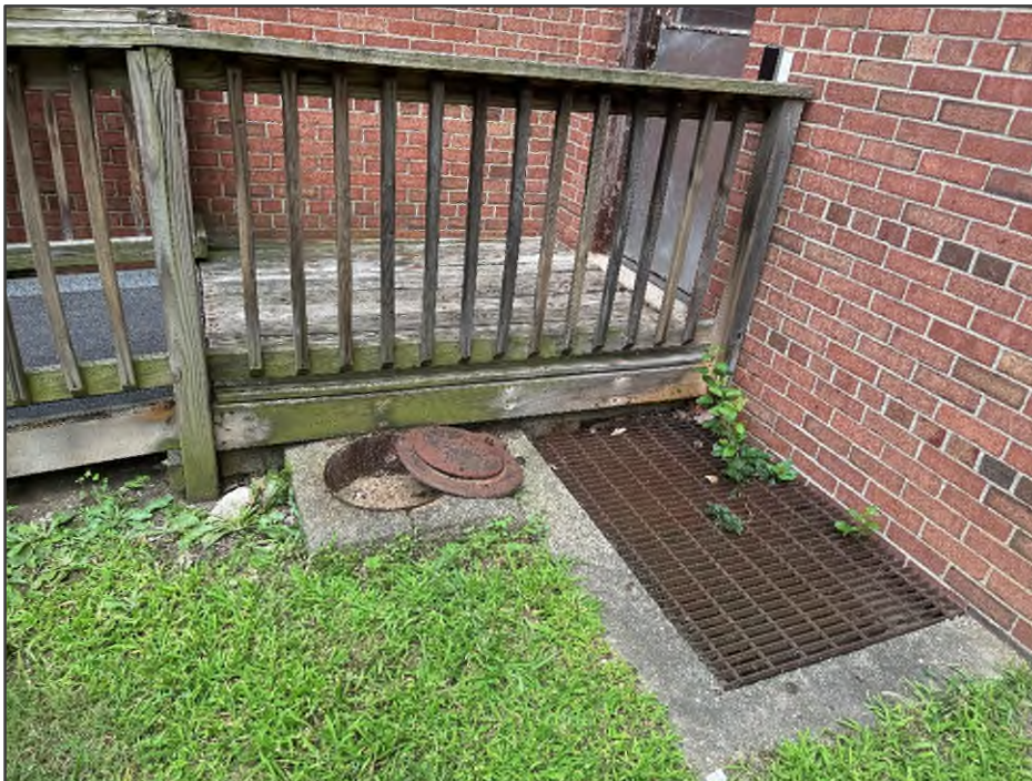
PHOTO NO. 12: View of an access cover and pit filled with debris on the southeastern portion of the former fire station building.
