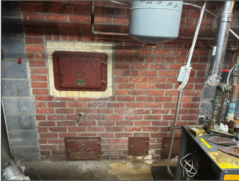
PHOTO NO. 23: View of the incinerator doors and a boiler unit observed in the central portion of the basement.
