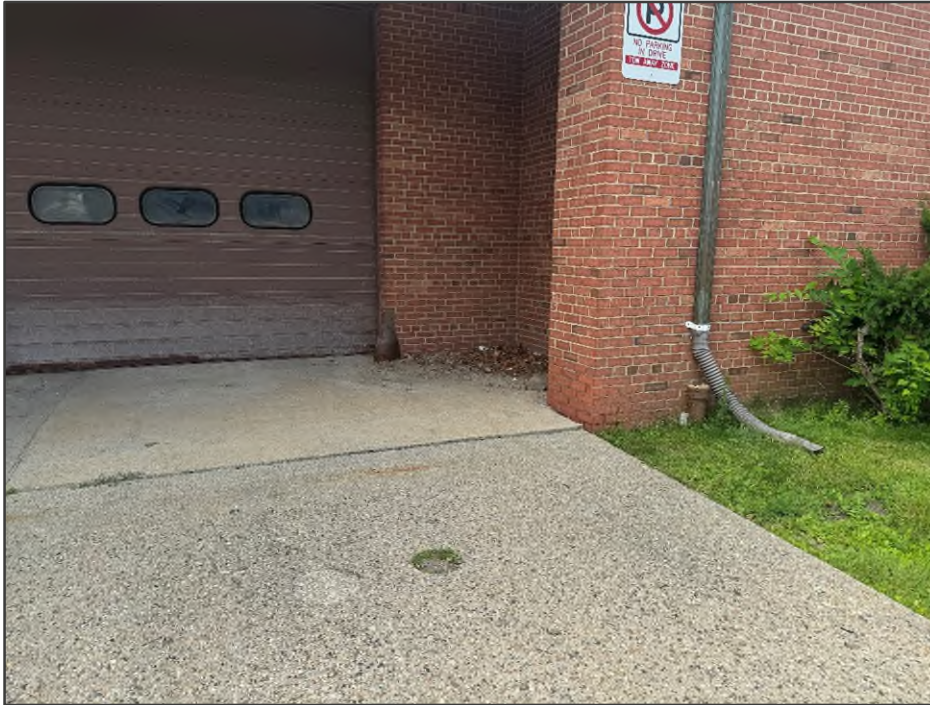
PHOTO NO. 9: View of circular cuts in the concrete, an area of patched concrete, and unidentified pipe next to a roof drain conduit.
