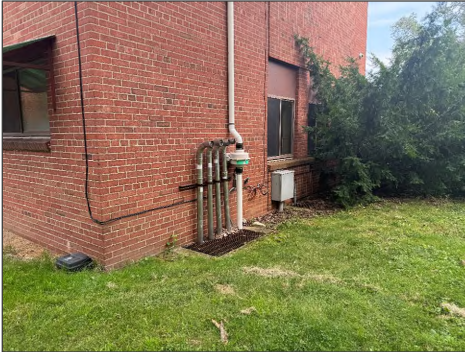
PHOTO NO. 11: View of the radon mitigation system piping observed at the southeast corner of the former fire station building.
