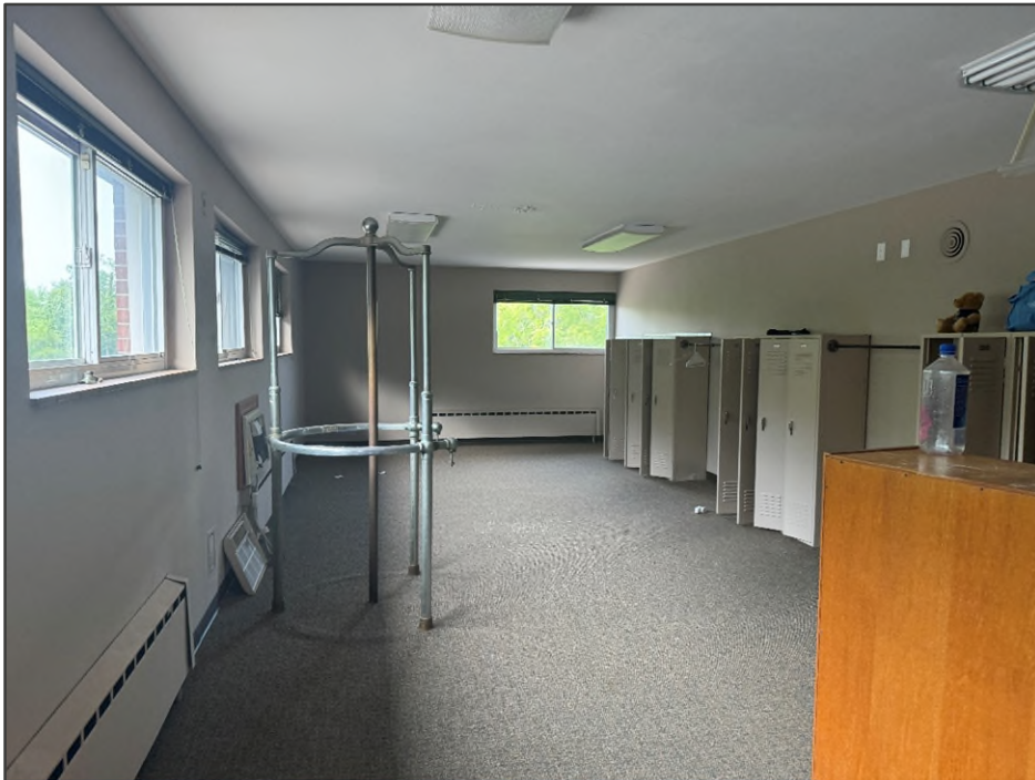
PHOTO NO. 22: View of a second floor locker-room area and sealed-off fire pole.
