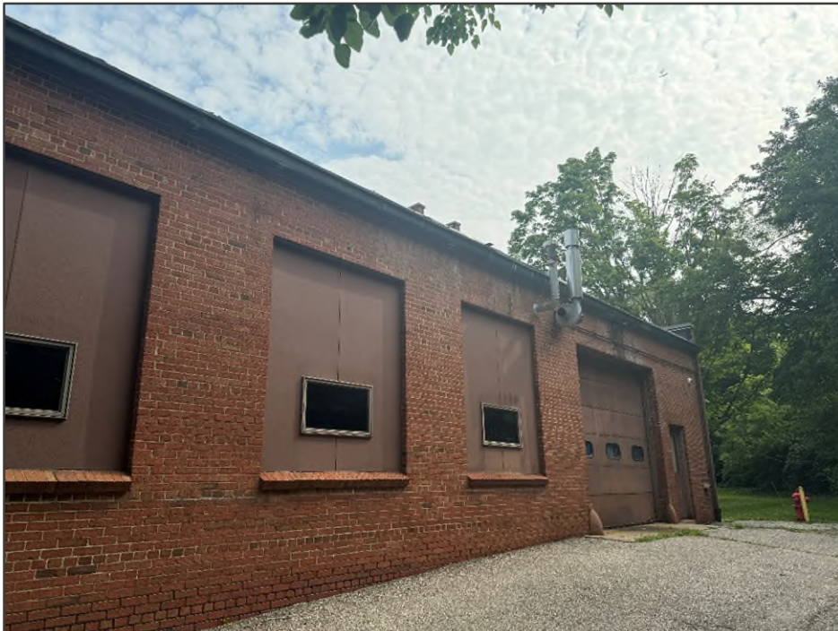
PHOTO NO. 14: View of the former fire truck exhaust ventilation from the garage area.
