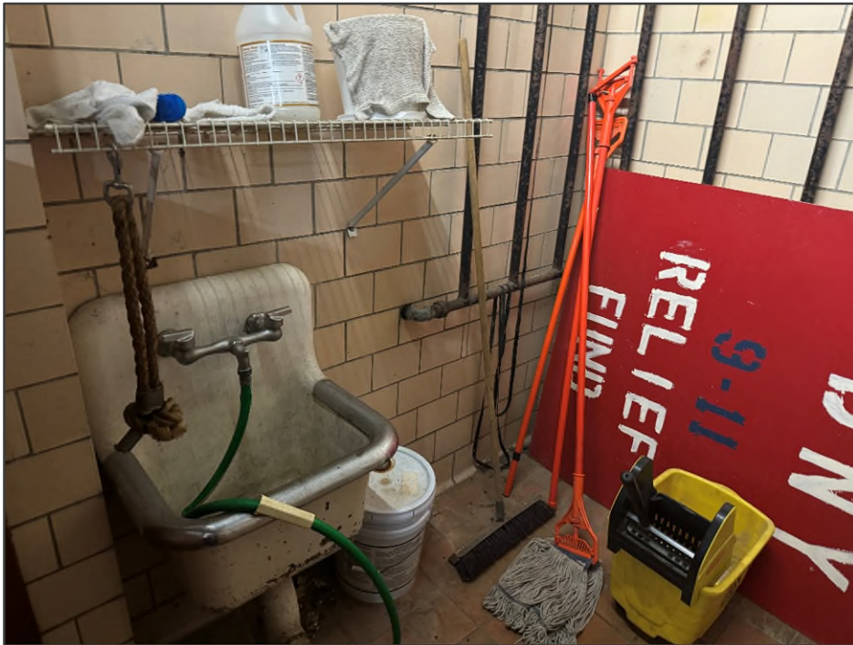
PHOTO NO. 26: View of a janitorial closet in the garage portion of the building.
