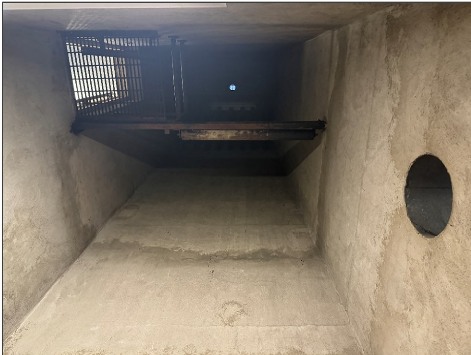
PHOTO NO. 28: View of the former fire hose drying tower (looking up).
