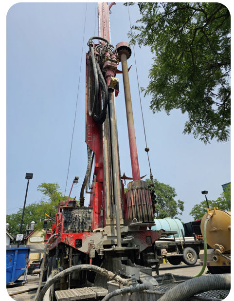
Test boring at 121 Catherine Street. This is a test drill to ensure that the area is viable and there aren't any issues in the subsurface. The actual drilling process is essentially the same.
