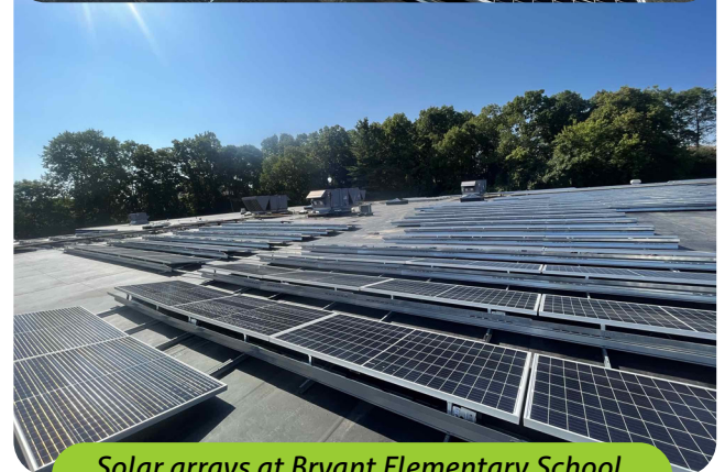
Solar arrays at Bryant Elementary School.
