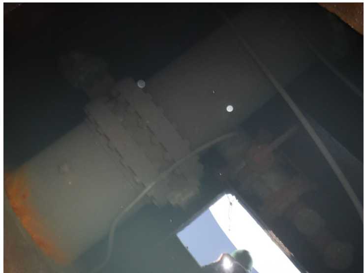
17) The pit is full of water and the coating on the piping appears to be in poor condition.
