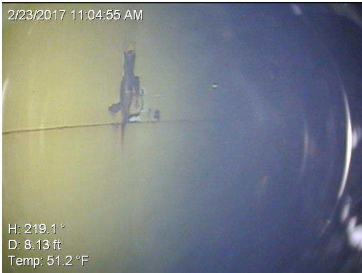
43) Delaminated coating to the steel substrate on the sidewall.
