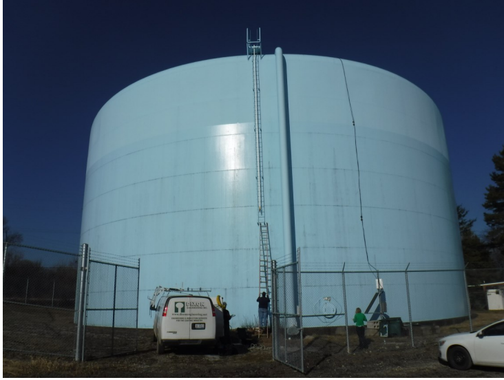
1) 4,000,000 gallon Industrial Drive reservoir located in Ann Arbor, Michigan.
