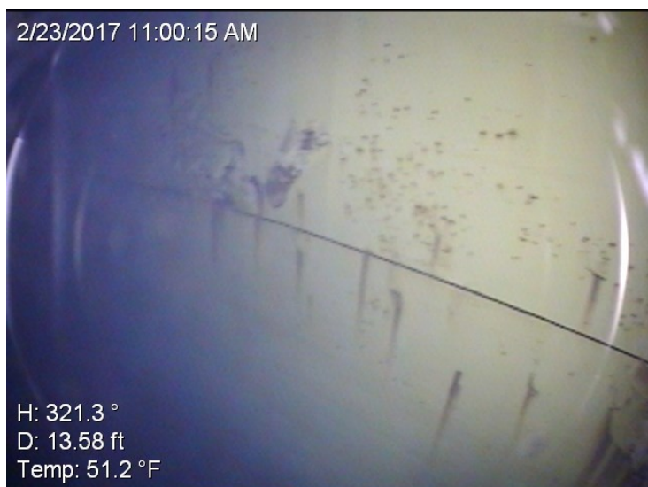
48) Rust bleedthrough and spot coating failures on the sidewall.
