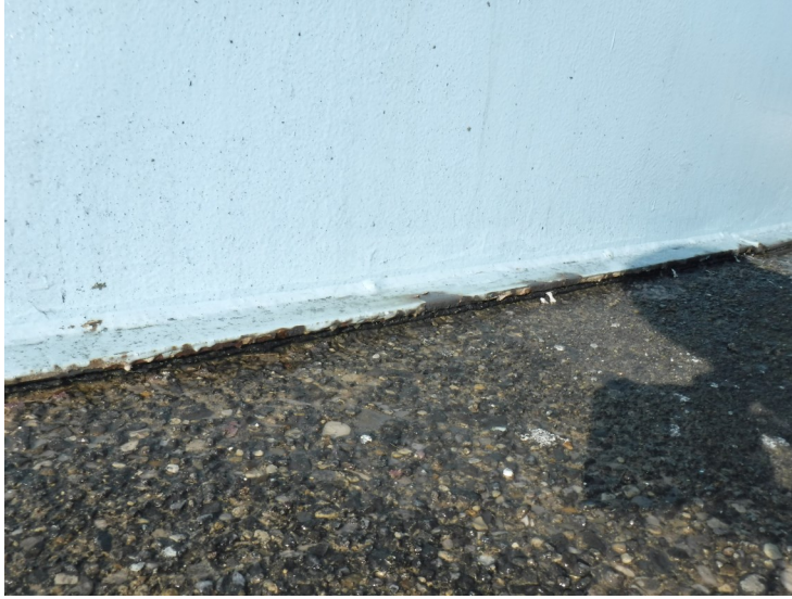
4) There is a gap between the baseplate and foundation with missing caulk on \frac{3}{4} of the circumference.
