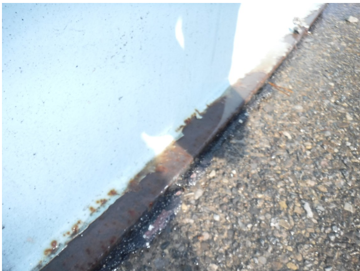
3) Coating deterioration on the top of the baseplate.
