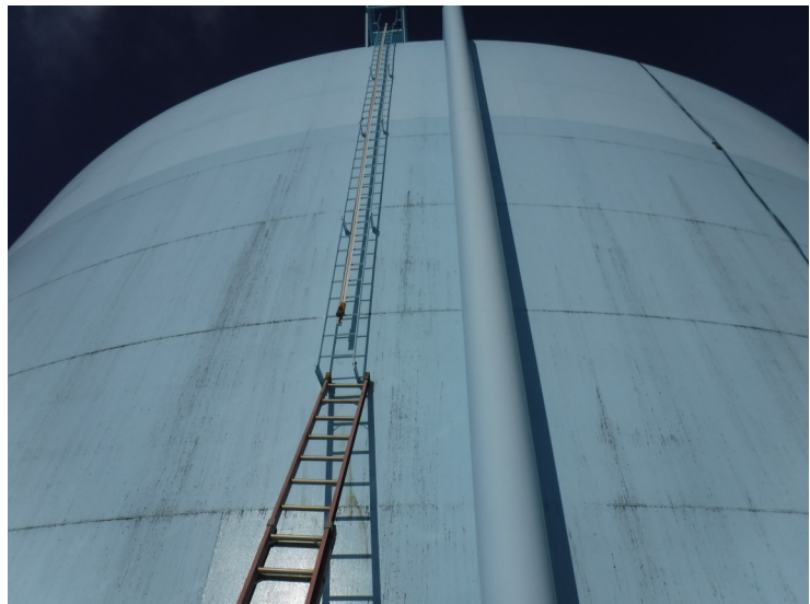
14) Overflow pipe routing and roof access ladder on the sidewall.
