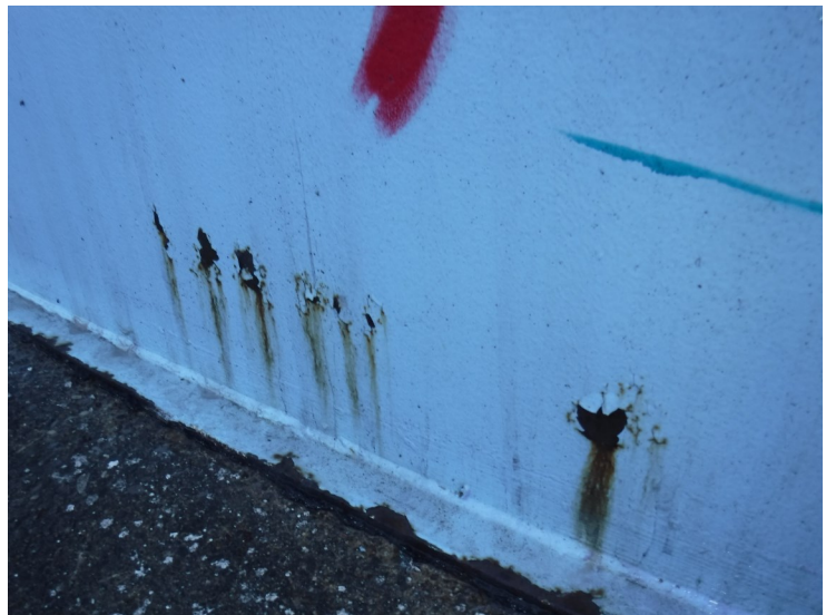
8) Spot failures with rust undercutting on the lower sidewall.
