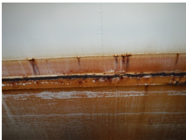
39) Sidewall stiffener with coating failure to the steel.
