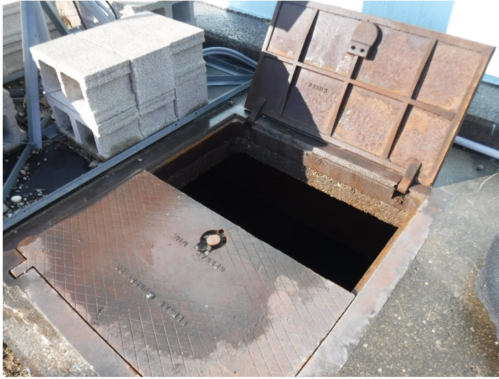
16) Pit piping cover with no handles.
