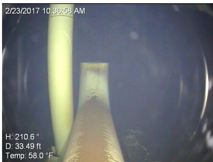
53) The pipe discharges near the center of the tank.
