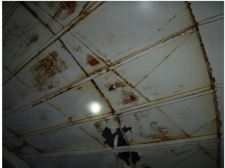
35) Rust bleedthrough and delamination on the roof.
