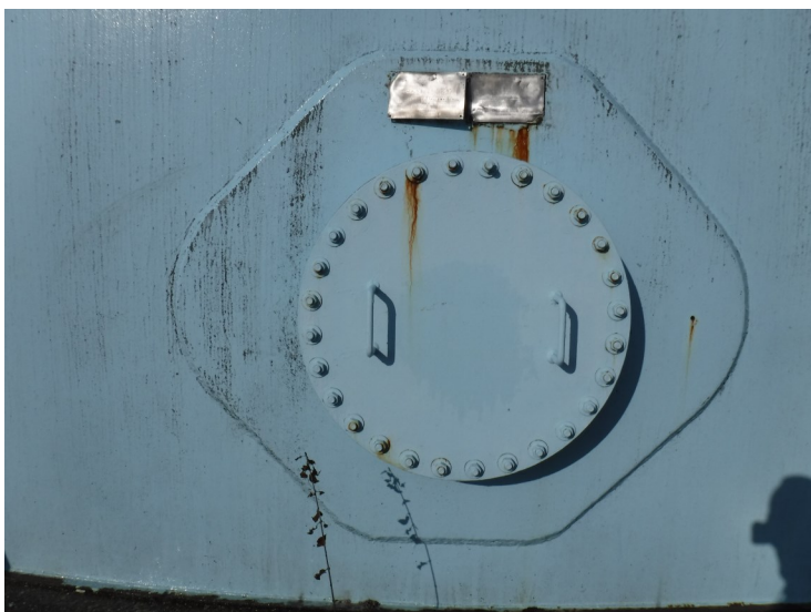
12) Sidewall manway nameplates that are not completely secure.
