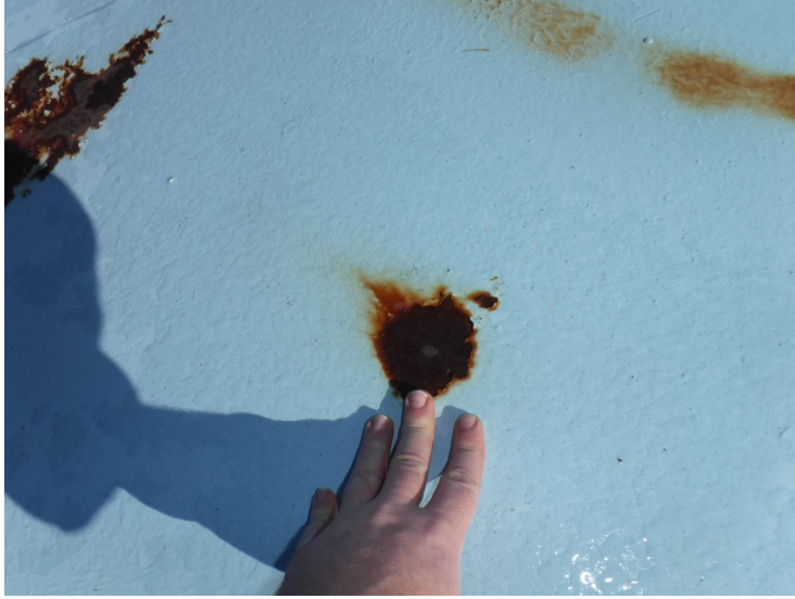
22) Spot coating failure on the roof.
