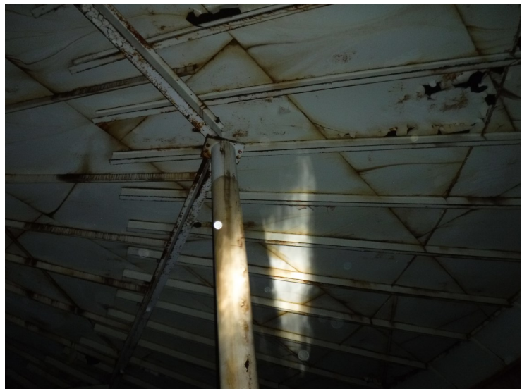
38) Coating failures on a column support.
