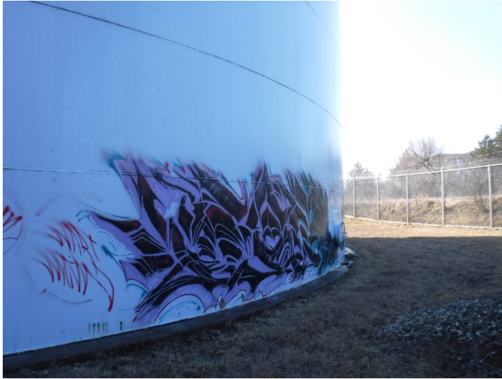
7) Graffiti on the sidewall facing the railroad tracks.
