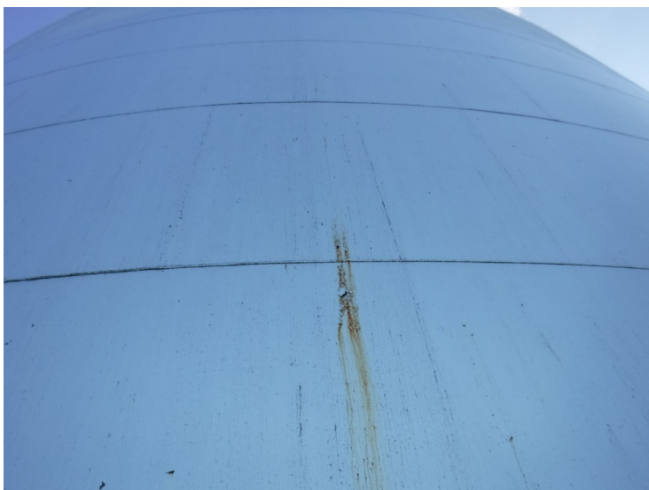
9) Rust bleedthrough and spot failures on the sidewall.
