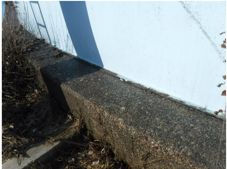
2) The foundation is in good condition overall with some aggregate exposed from weathering.
