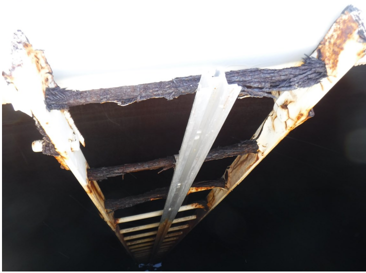
31) Extensive corrosion on the upper four ladder rungs.
