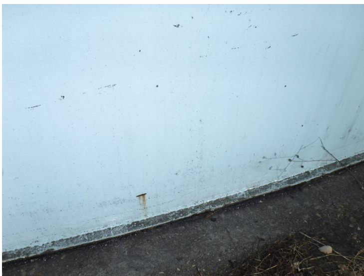
6) Coating failures to the steel substrate on the lower sidewall.
