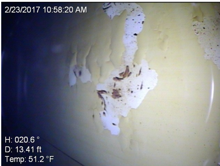
46) Coating delamination to the previous coat with areas to the steel substrate.
