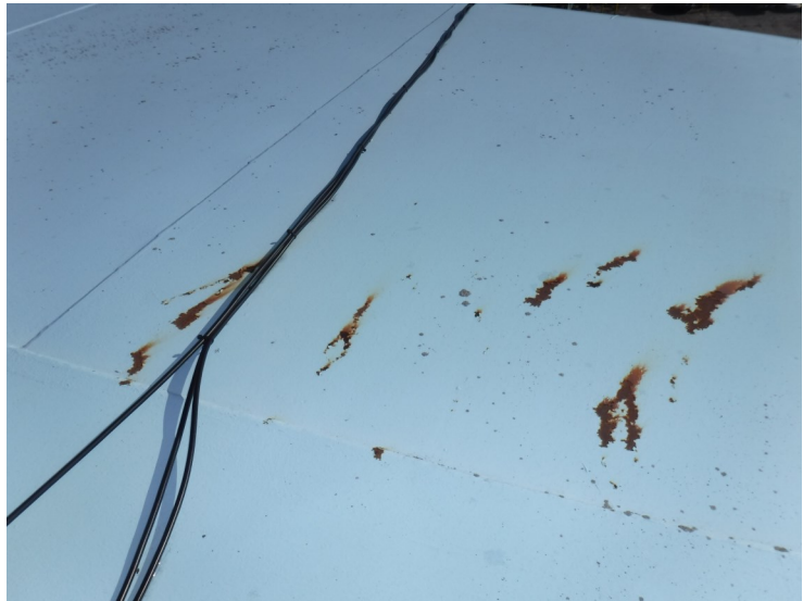
20) Coating failures to the steel substrate on the roof.
