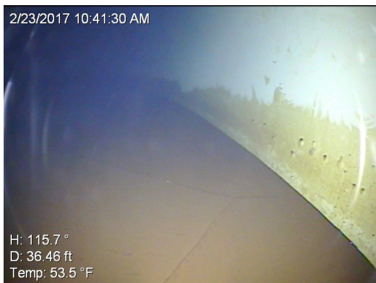
51) Coating failures on the bottom of the sidewall.
