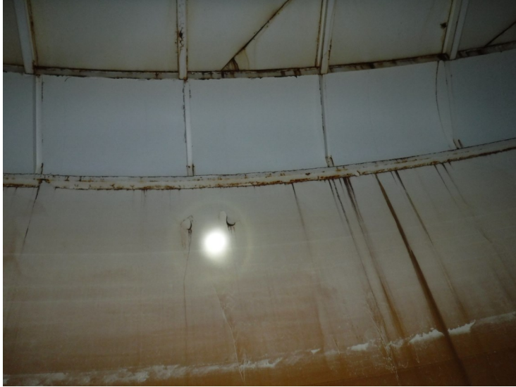
40) Delaminated coating to the steel substrate on the upper sidewall.
