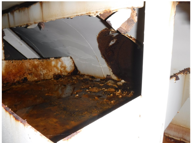
32) Extensive coating failure on the interior of the overflow weir box.
