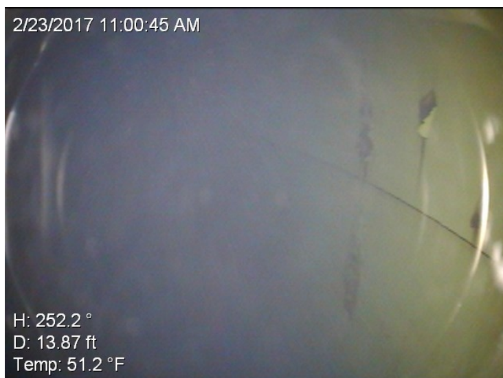
45) Area of delamination to the steel substrate.
