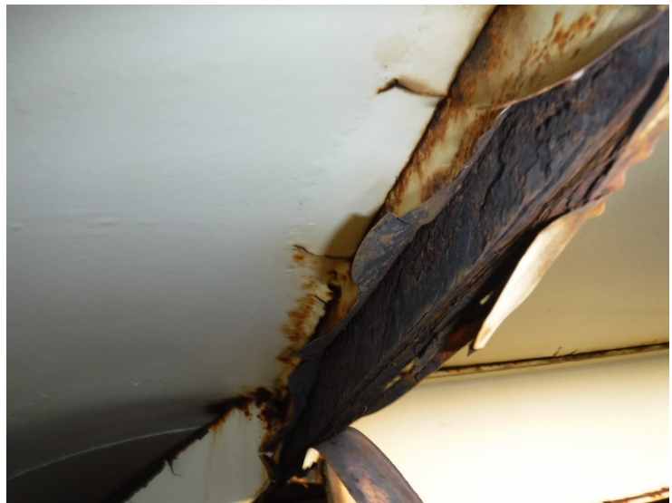
29) Section of the wind girder with extensive steel loss.
