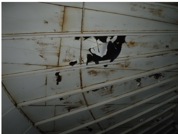
33) Coating delaminated to the steel substrate on the roof panels in numerous areas.
