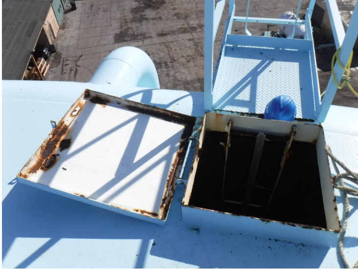
19) The coating on the interior of the hatch is in poor condition.
