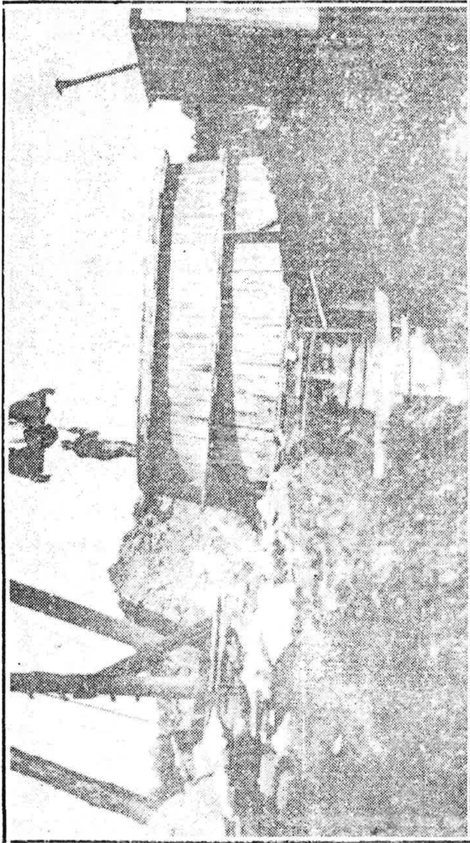
Sixteen foot well under construction. Excavating clay from inside of well casing. Concrete in place but forms not yet removed.
