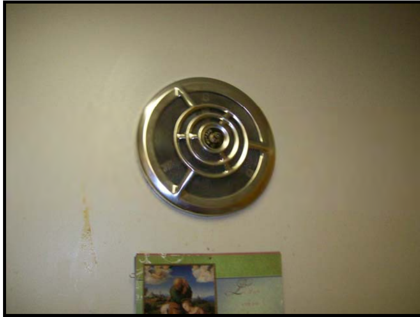
PHOTOGRAPH NO. 15: SUBJECT BUILDING: TYPICAL VIEW OF TENANT UNIT EXHAUST FAN (KITCHEN)
