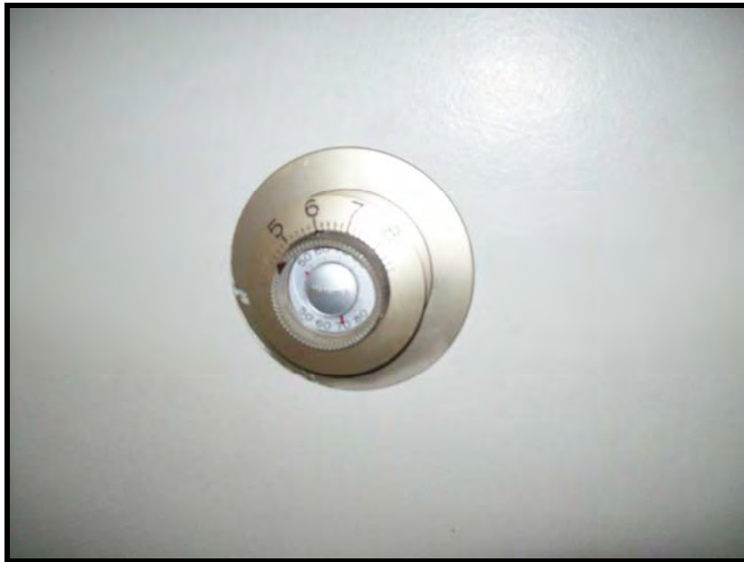
PHOTOGRAPH NO. 18: SUBJECT BUILDING: TYPICAL VIEW OF TENANT UNIT THERMOSTAT
