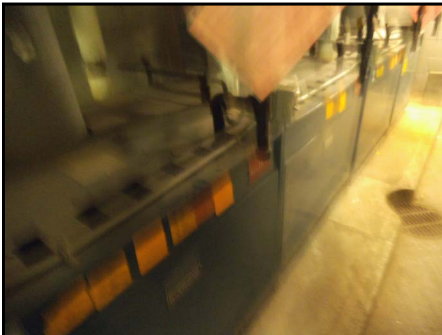
PHOTOGRAPH NO. 6: SUBJECT BUILDING: VIEW OF GAS-FIRED BURNHAM BOILERS
