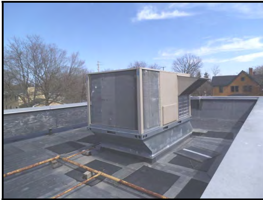
PHOTOGRAPH NO. 3: SUBJECT BUILDING: VIEW OF OFFICE WING PACKAGE RTU
