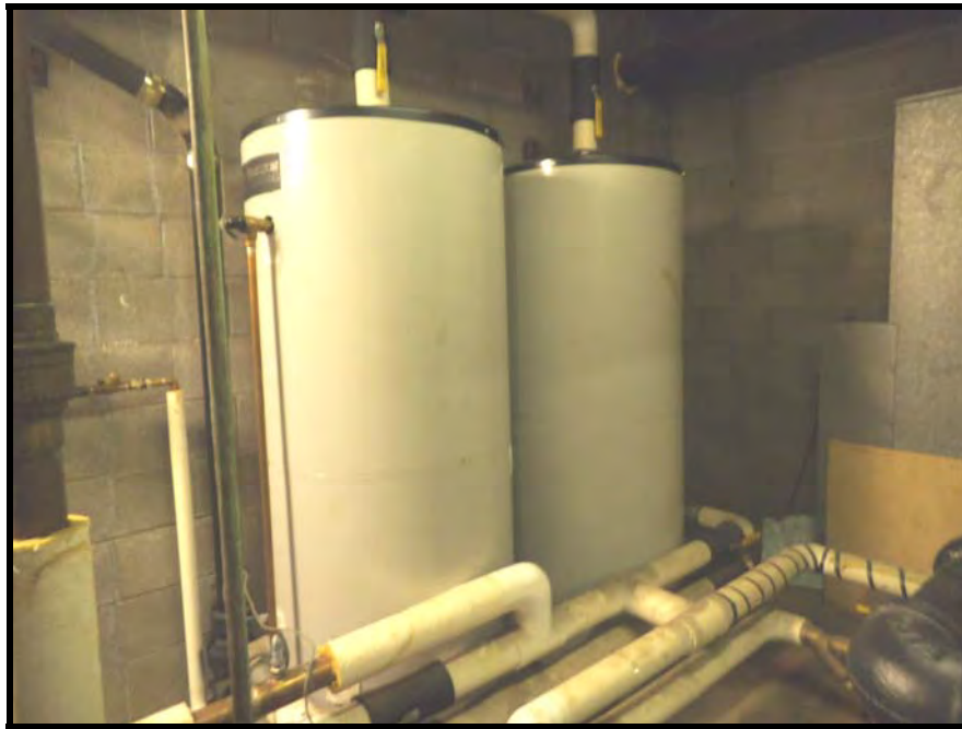
PHOTOGRAPH NO. 5: SUBJECT BUILDING: VIEW OF HOT WATER TANKS
