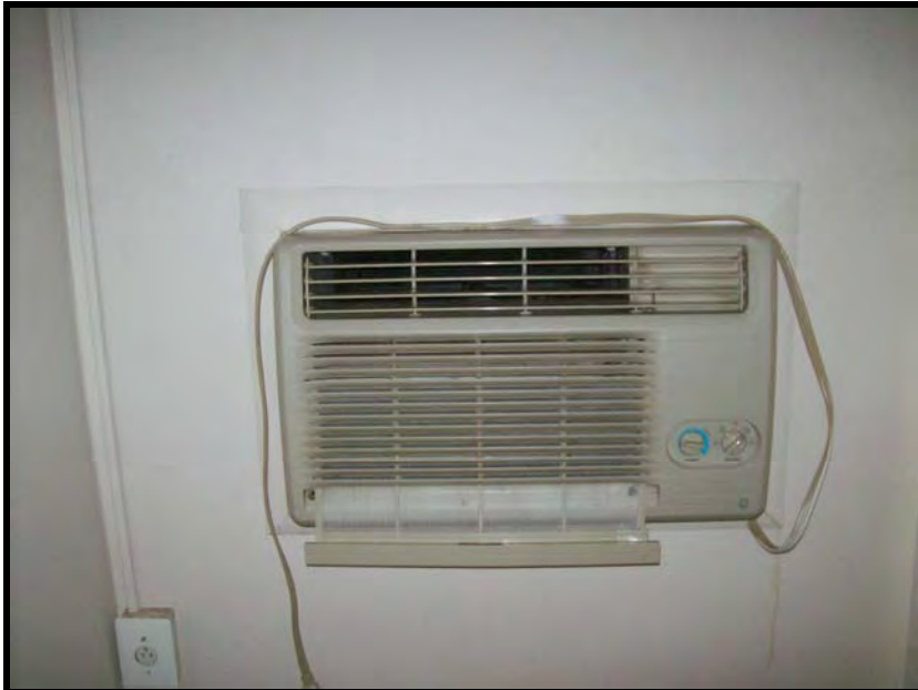
PHOTOGRAPH NO. 8: SUBJECT BUILDING: TYPICAL VIEW OF TENANT UNIT AIR CONDITIONER
