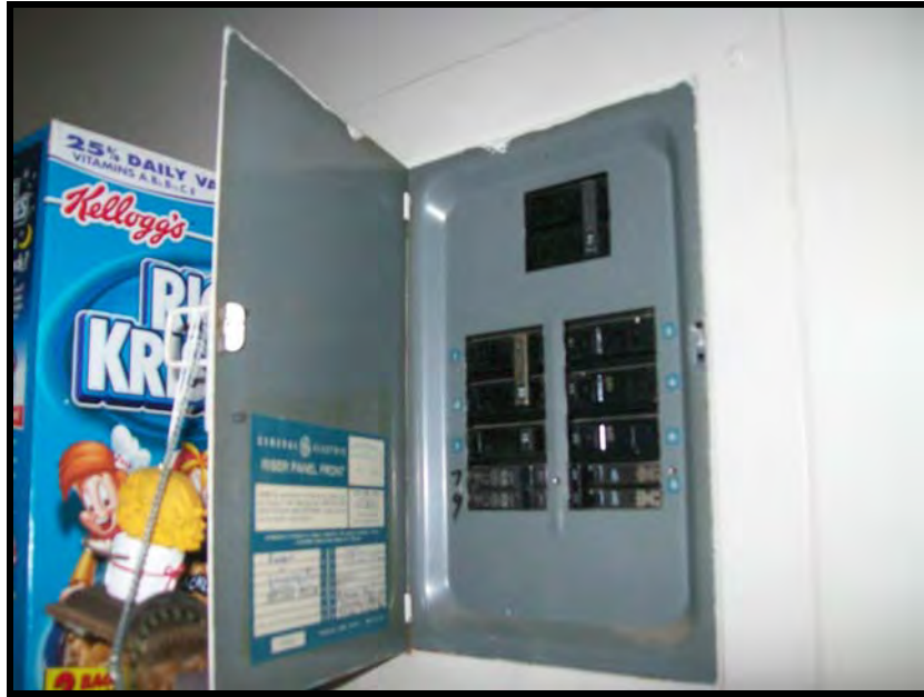
PHOTOGRAPH NO. 9: SUBJECT BUILDING: TYPICAL VIEW OF TENANT UNIT ELECTRICAL PANEL
