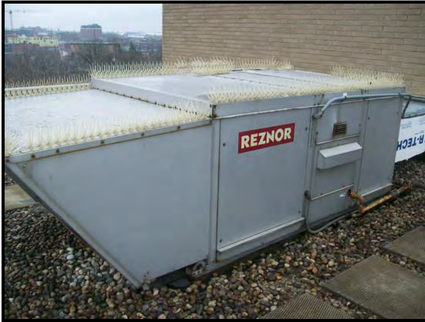
PHOTOGRAPH NO. 7: SUBJECT BUILDING: TYPICAL VIEW OF REZNOR MUA UNIT
