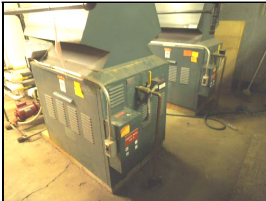
PHOTOGRAPH NO. 4: SUBJECT BUILDING: TYPICAL VIEW OF GAS-FIRED HOT WATER BOILERS
