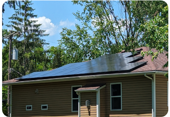
Solar panels installed through the Solarize Ann Arbor program this past year.
