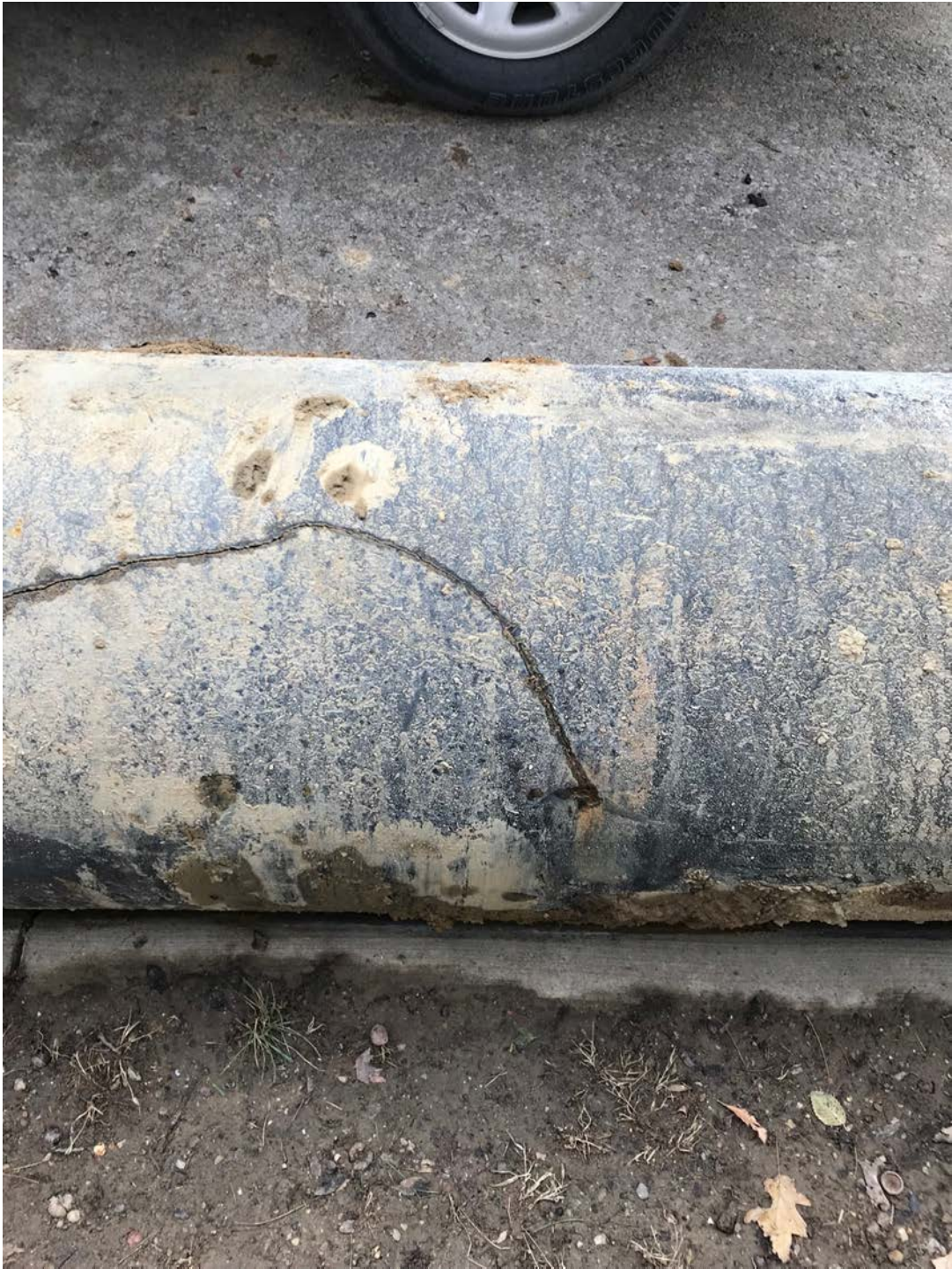
Figure 6 - 24" 1949 CI Main from Break along Sunset Road, Deep Pitting at Start of 14' Crack that Extended Through to a Joint
