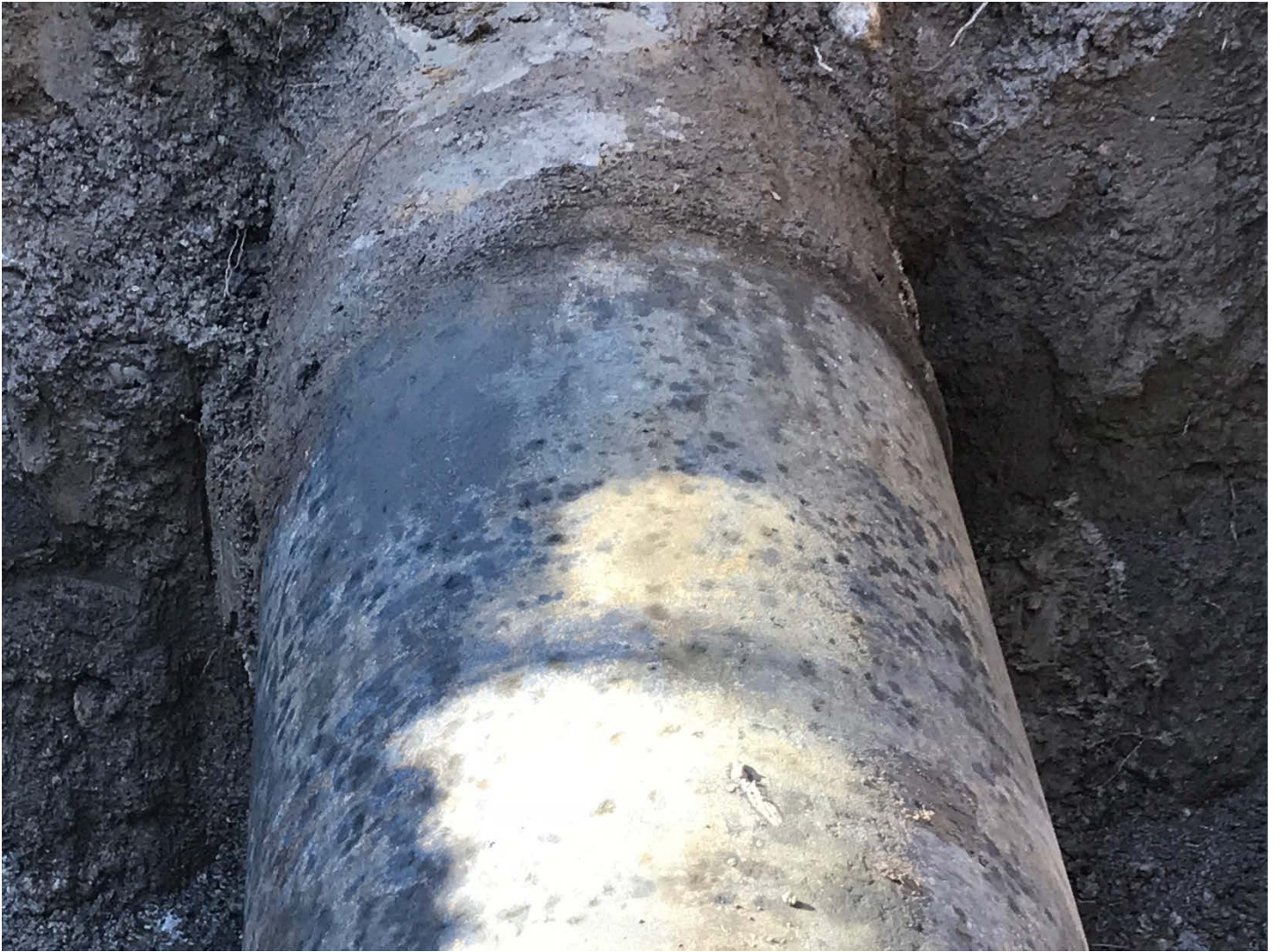
Figure 3 - 24" 1965 DI Main at Barton PS, Pitting where Tapping Sleeve was Installed
