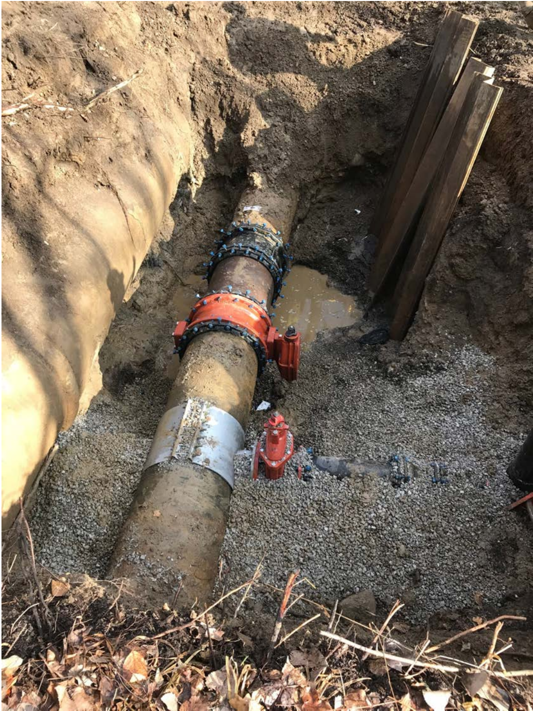
Figure 1 - 24" 1965 DI Main at Barton PS, 42" PCCP Main Seen to the West
