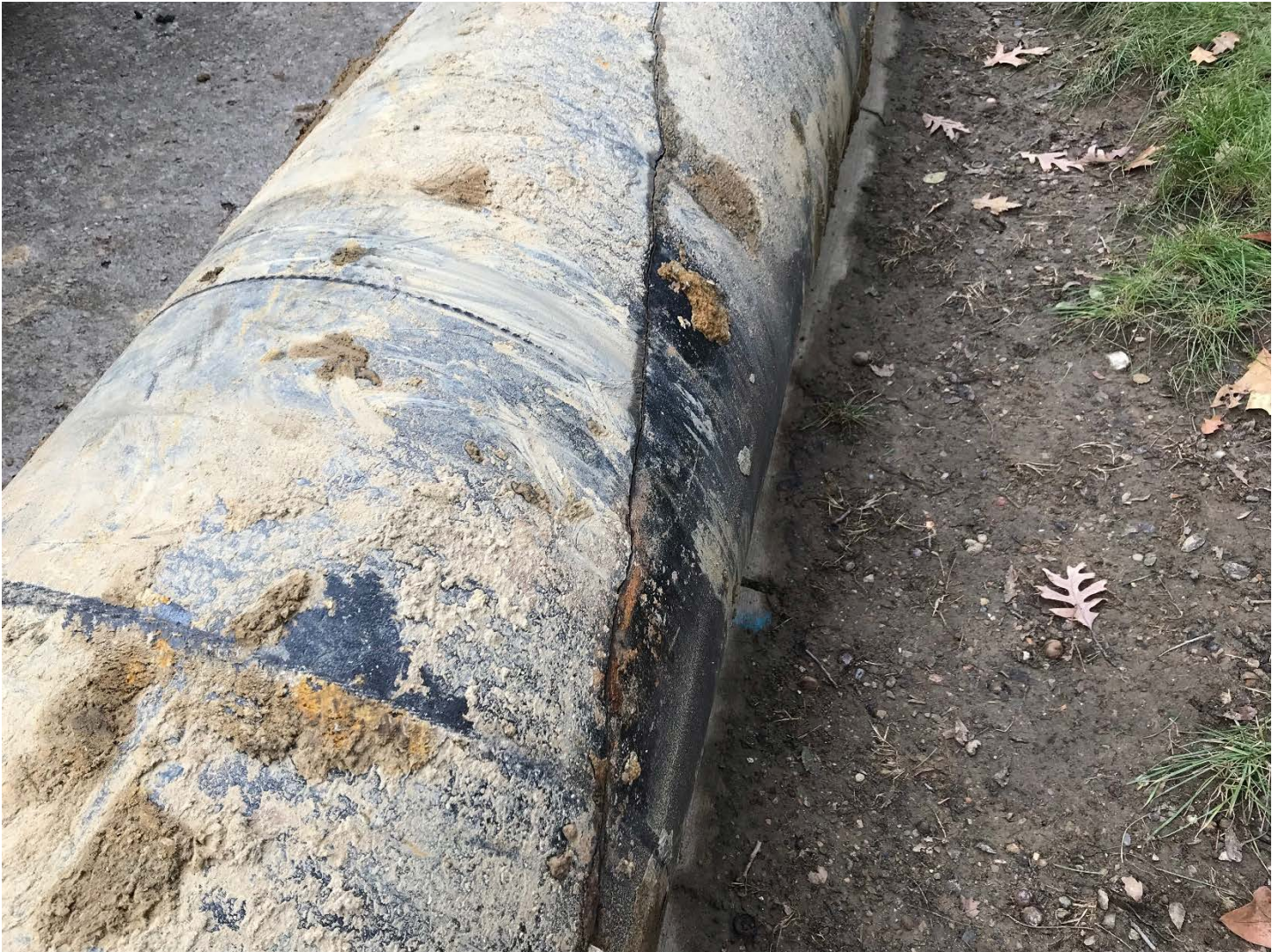
Figure 4 - 24" 1949 CI Main from Break along Sunset Road, 14' Long Crack
