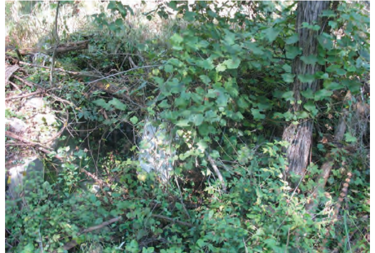
Viewing the remnants of a building foundation and a washing machine located in the southeast corner of the Subject Property, adjacent to the aforementioned potential vent pipe.
