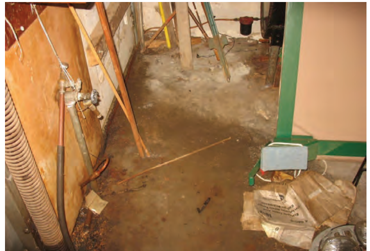
Viewing stained concrete located adjacent to the previously mentioned 275-gallon AST.
