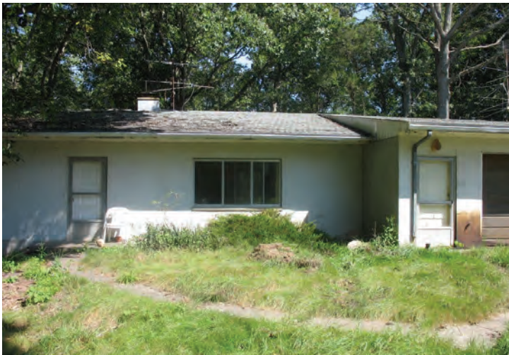
Facing east viewing a house located in the west-central portion of the Subject Property.
