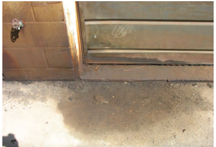
Viewing stained concrete located adjacent to the house garage door.
