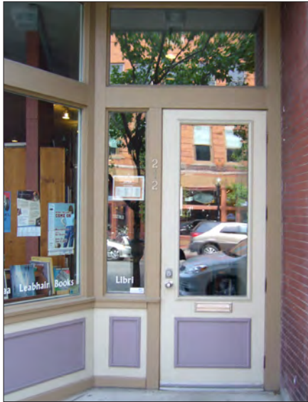
Retain, repair and maintain original doors and trim including surrounds and transoms.
