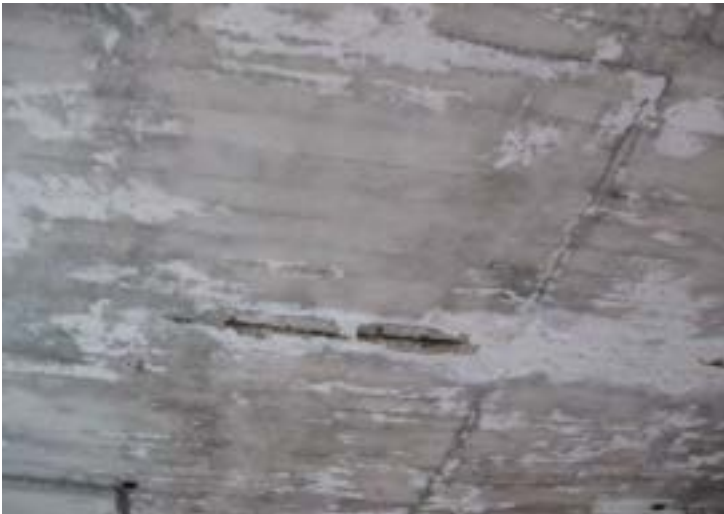
[5] Rebars in the reinforced concrete ceiling have rusted, causing the concrete to spall. The rebars must be cleaned of rust before the concrete can be patched.
