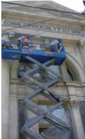
[1] An alkaline-based product is appropriate to use to clean historic marble because it will not damage the marble, which is acid sensitive.
