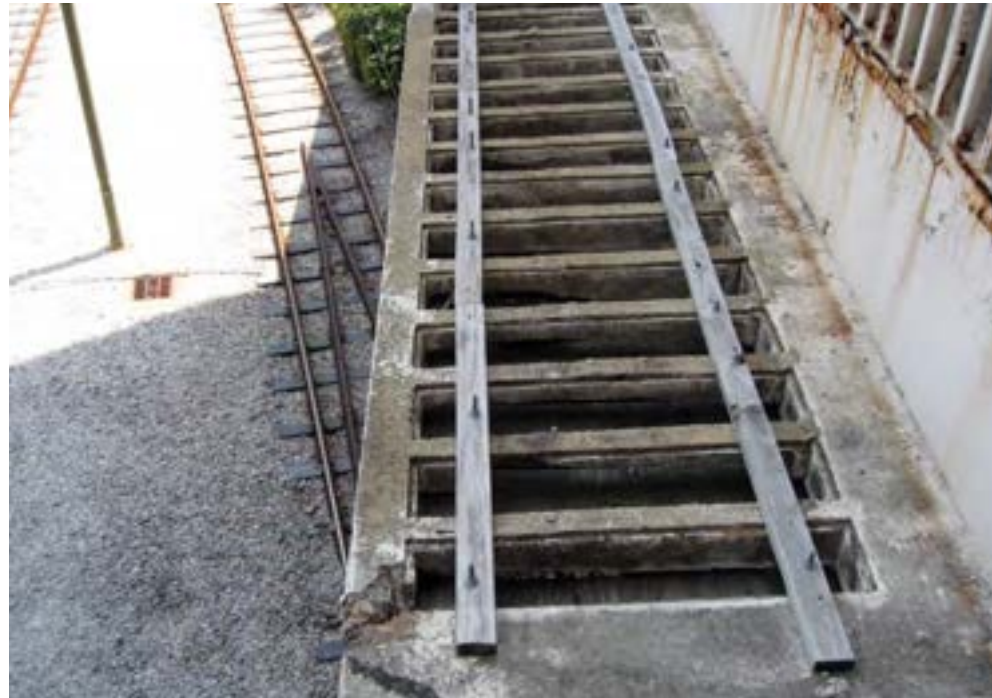
[6] Some areas of the concrete brise soleil screen on this building constructed in 1967 are badly deteriorated. If the screen cannot be repaired, it may be replaced in kind or with a composite substitute material with the same appearance as the concrete.
