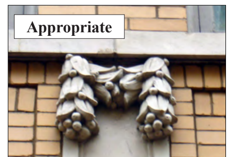
Protect, maintain and preserve masonry features and surfaces that contribute to the overall character of a historic building.
