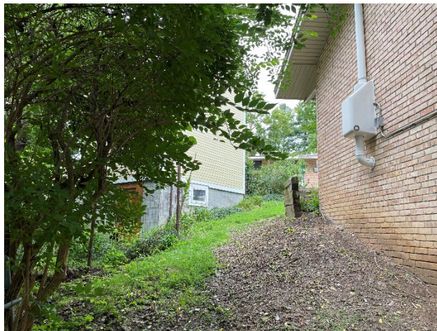
Photograph 15: View of the west elevation of building 1508, and adjoining residential dwelling to the west.
