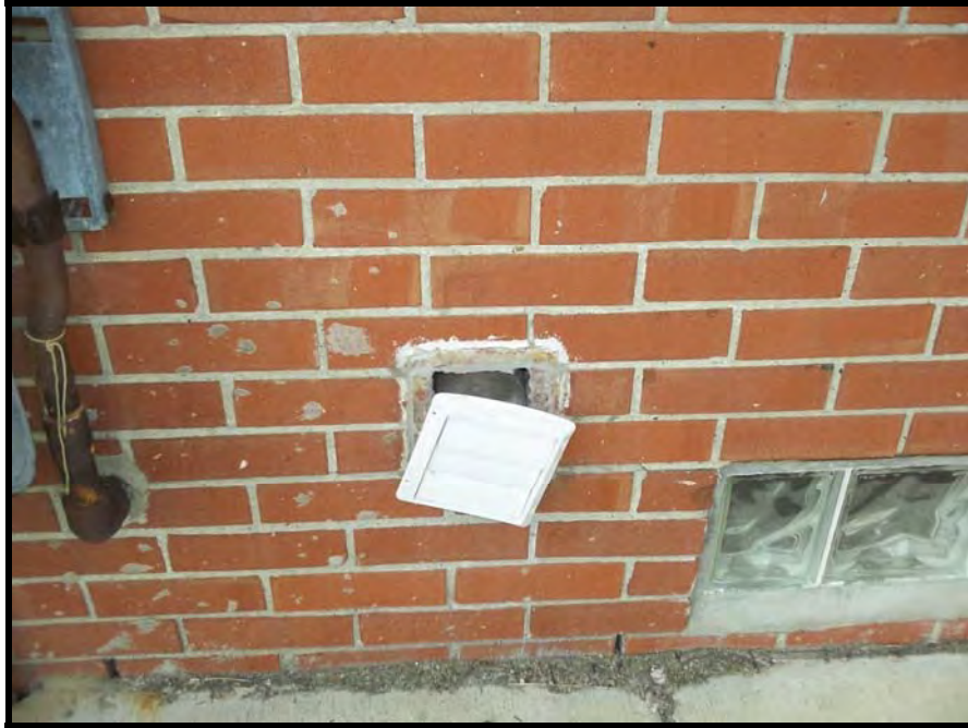
PHOTOGRAPH NO. 21: VIEW OF DAMAGED VENT PLATE ON EXTERIOR OF BUILDING
