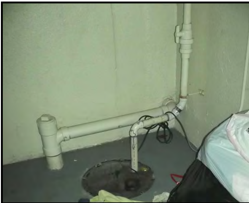
PHOTOGRAPH NO. 18: TYPICAL VIEW OF SUMP PUMP IN BASEMENT
