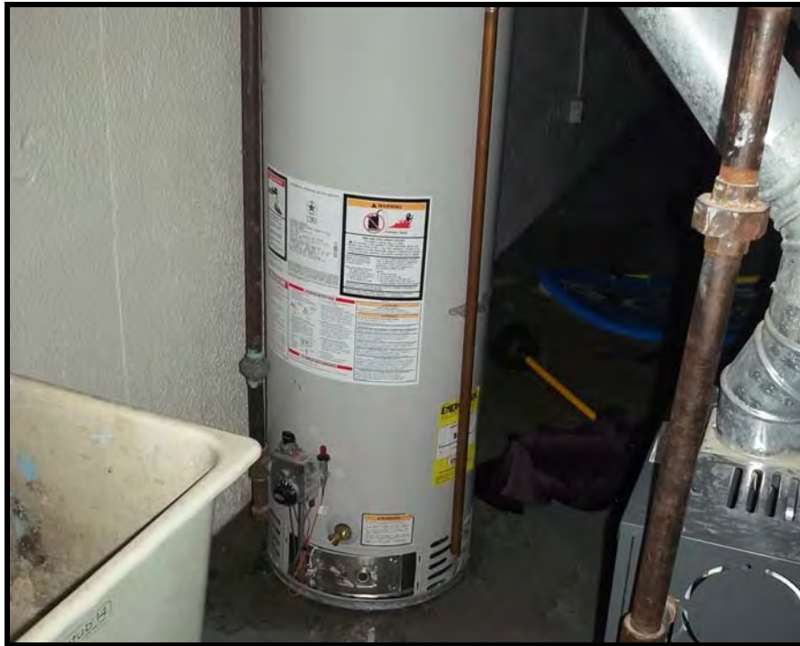
PHOTOGRAPH NO. 11: TYPICAL VIEW OF HOT WATER HEATERS IN TENANT UNITS
