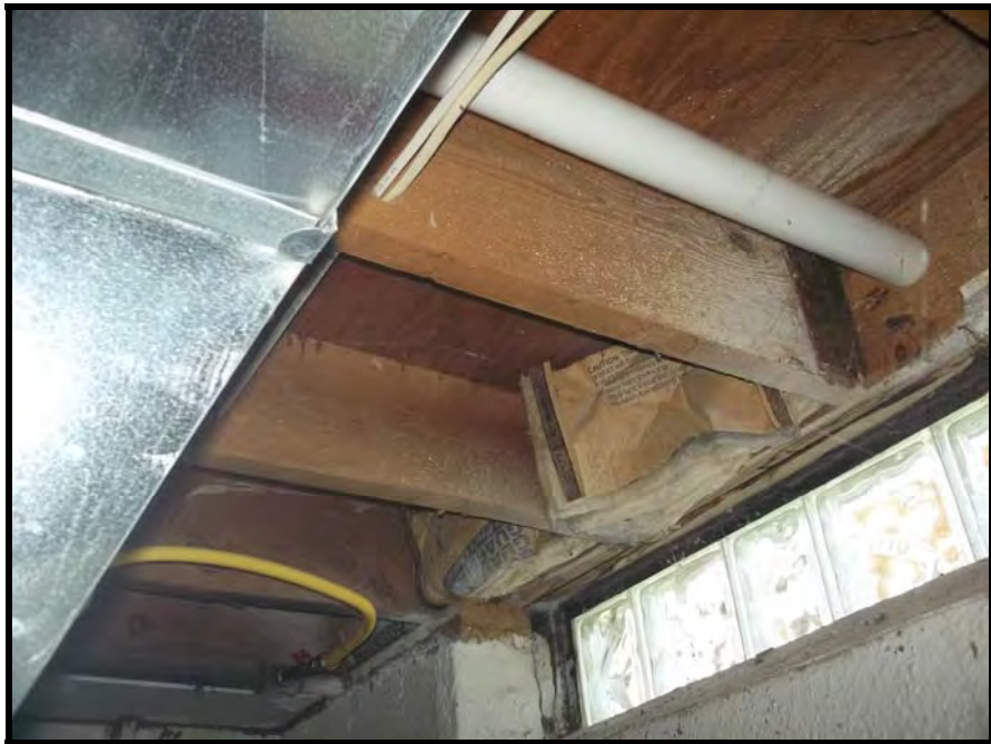
PHOTOGRAPH NO. 10: TYPICAL VIEW OF DUCTWORK AND JOIST BRACING IN TENANT UNIT BASEMENT
