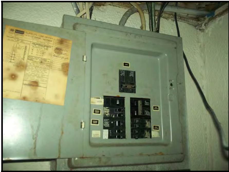
PHOTOGRAPH NO. 9: TYPICAL VIEW OF ELECTRICAL PANELS IN TENANT UNITS
