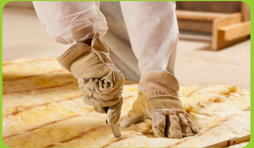
Home insulation is an important component of any energy waste reduction strategy and is the second most impactful step for increasing the energy efficiency of any building.
