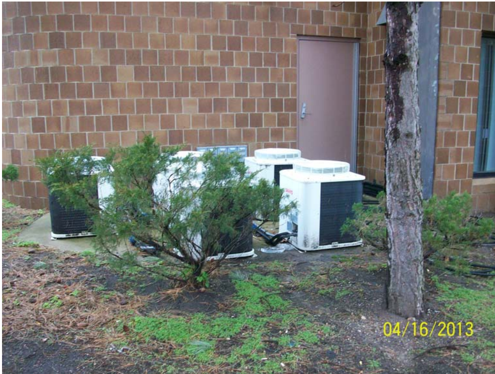
Photograph 7: Air conditioning units observed on the north side of the building.
