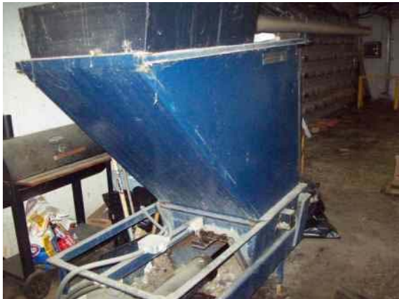
Photo #75: Trash compactor
