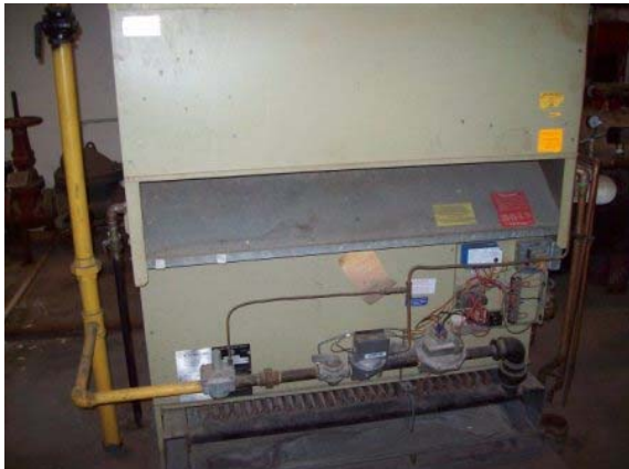
Photo #51: Domestic water boiler
