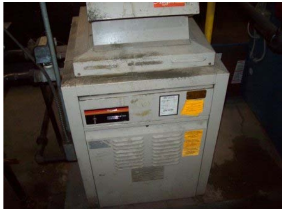
Photo #36: Raypack boiler
