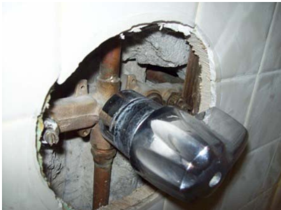
Photo #53: Typical shower mixing valve
