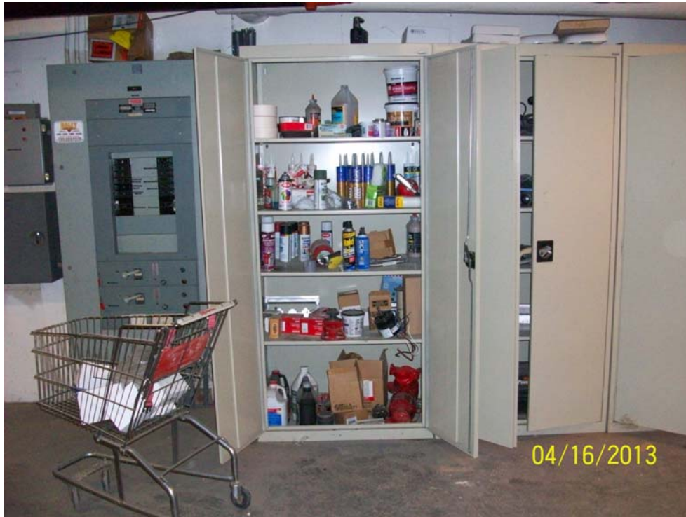
Photograph 19: Maintenance material storage observed in the basement of the building.
