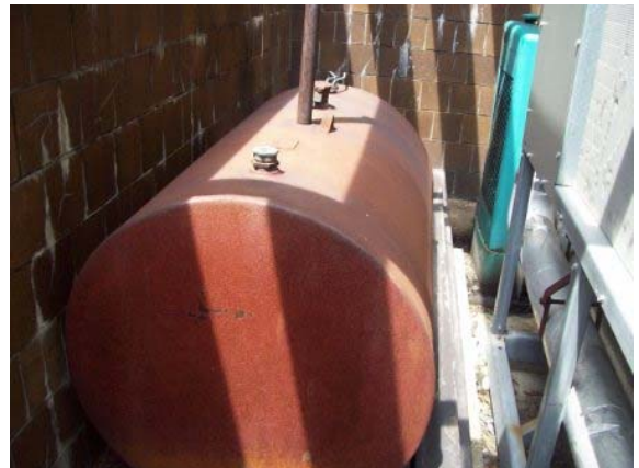
Photo #60: Above-ground diesel storage tank
