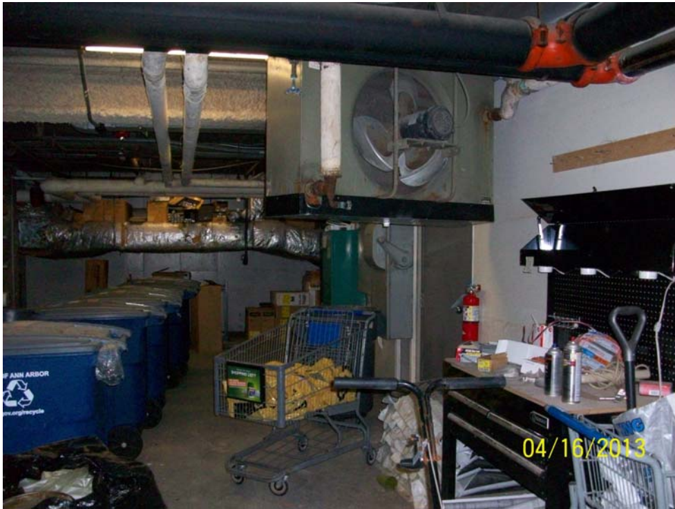
Photograph 17: Storage observed in the basement of the building.
