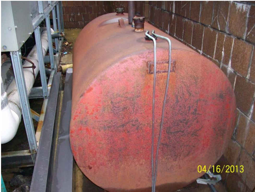
Photograph 23: Above ground storage tank observed within a brick storage area (holding chillers and the emergency generator, and above ground storage tank) on the west side of the building.
