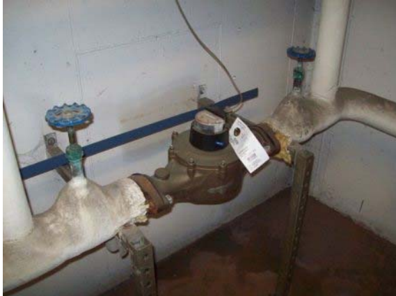
Photo #49: Domestic water meter
