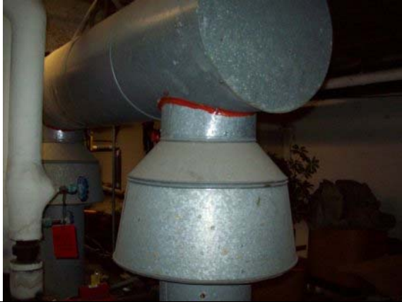
Photo #37: Boiler exhaust stack
