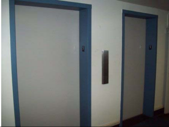
Photo #61: Elevator cab doors
