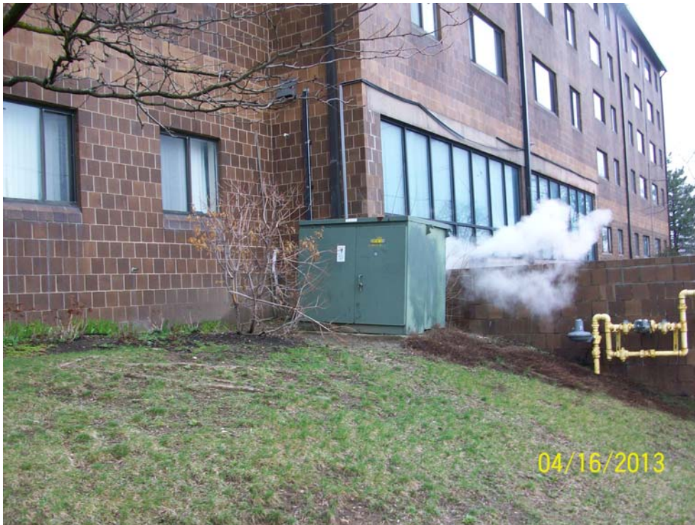
Photograph 8: Pad mounted transformer and natural gas connection on the west side of the building.
