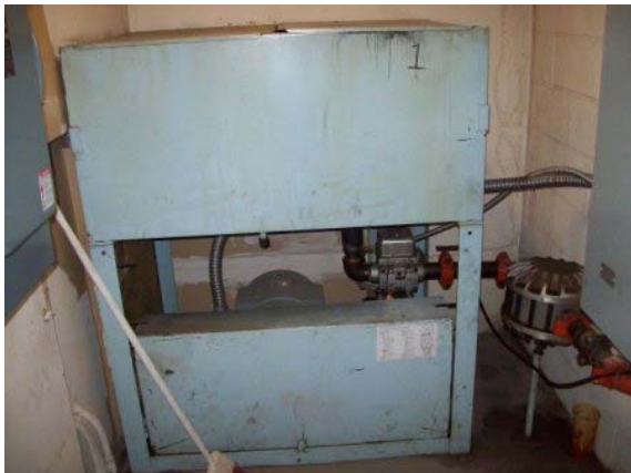
Photo #65: Hydraulic elevator equipment
