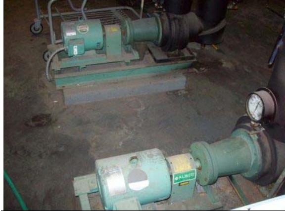
Photo #38: Circulating pumps
