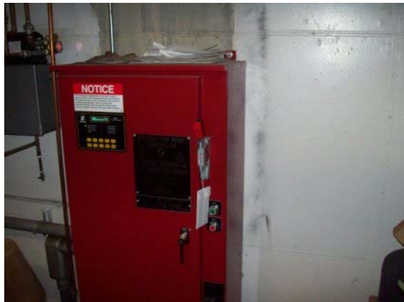
Photo #71: Fire pump controller
