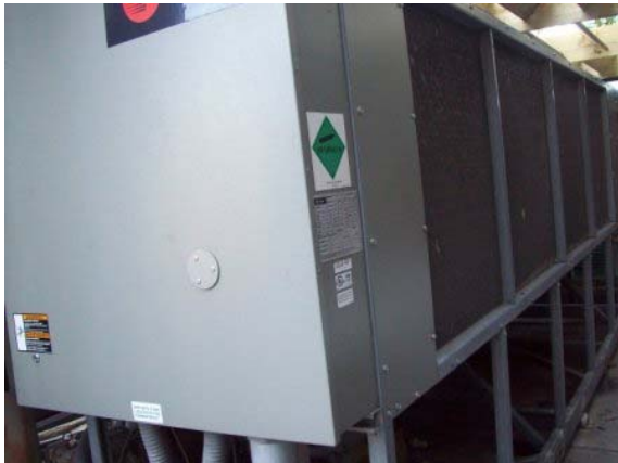
Photo #39: Air cooled chiller
