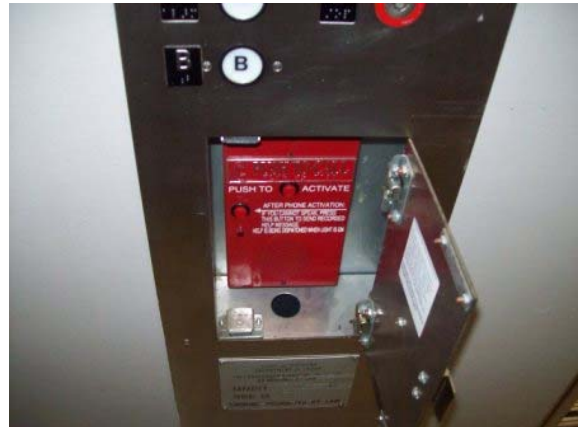
Photo #64: Emergency communication equipment
