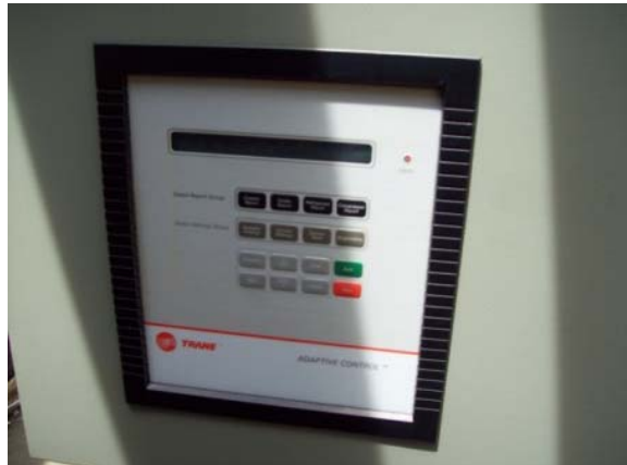
Photo #40: Chiller control module
