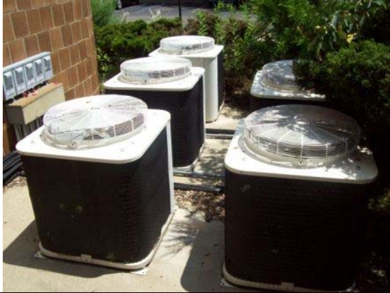
Photo #43: Split system heat pumps
