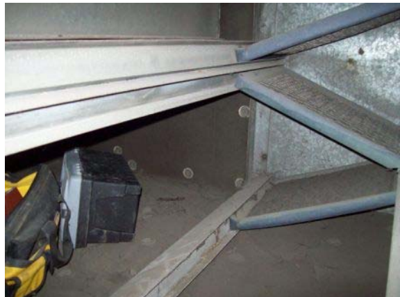
Photo #42: Interior of make-up air unit - appears not to be functioning.
