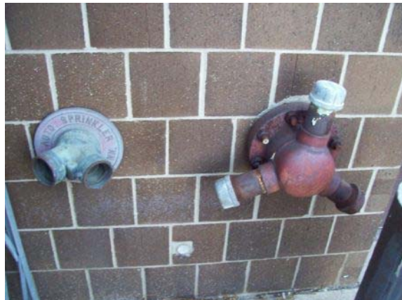
Photo #72: Exterior hose connections
