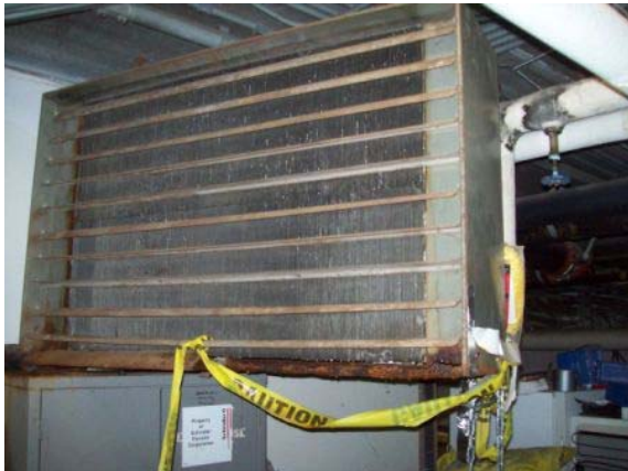
Photo #45: Supplemental heating unit for basement
