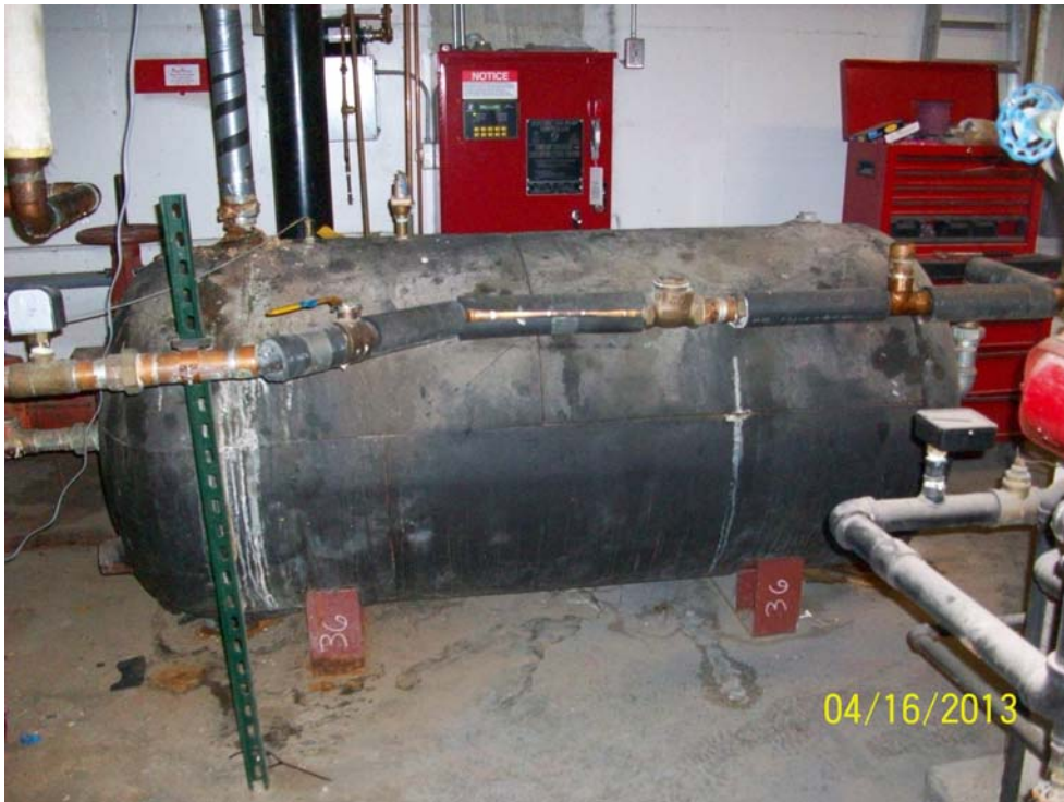
Photograph 18: Mechanical equipment observed in the basement of the building.
