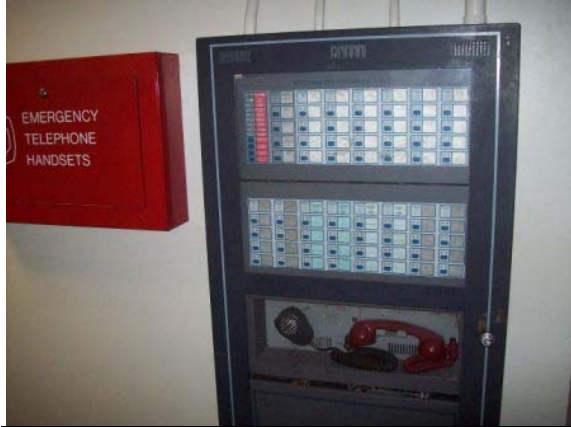
Photo #67: Fire alarm panel - to be replaced
