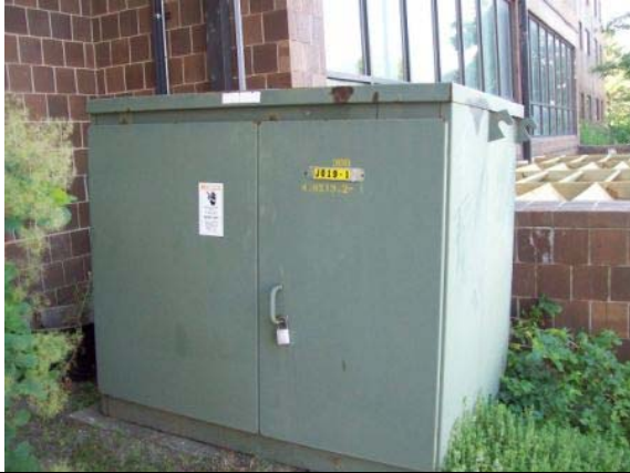
Photo #55: Electrical transformer
