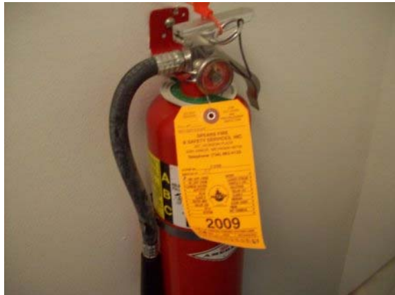
Photo #69: Fire extinguisher
