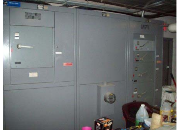
Photo #56: Main switchgear and common electric meter
