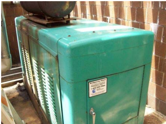
Photo #59: Emergency generator
