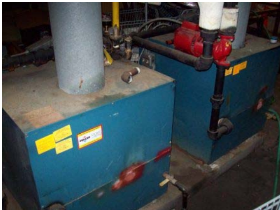
Photo #35: Burnham boilers
