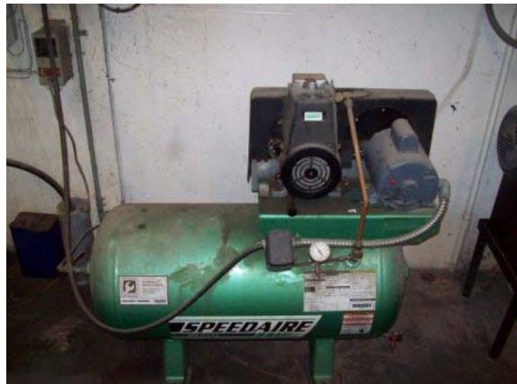
Photo #48: Air compressor for pneumatic controls
