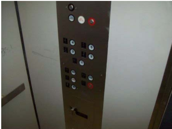
Photo #63: Elevator control panel
