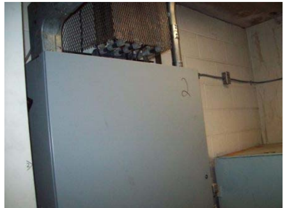
Photo #66: Elevator control unit
