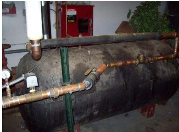
Photo #52: Hot water storage tank
