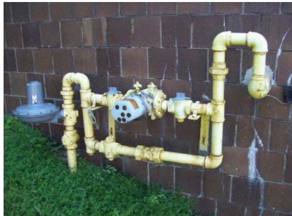
Photo #54: Gas meter and regulator
