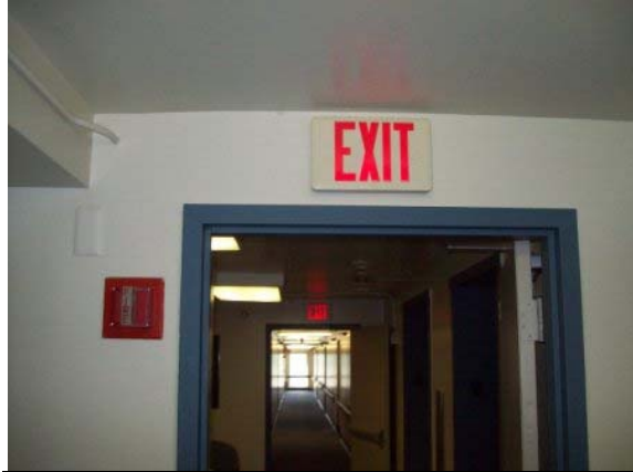
Photo #68: Exit sign and fire alarm horn with strobe light
