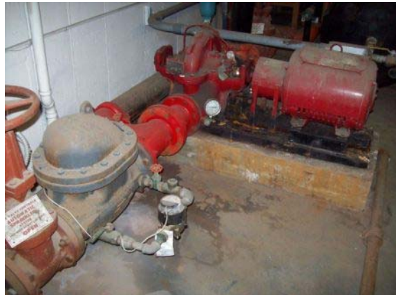
Photo #70: Fire pump
