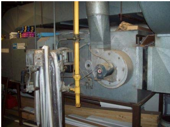
Photo #41: Make-up air unit for corridors
