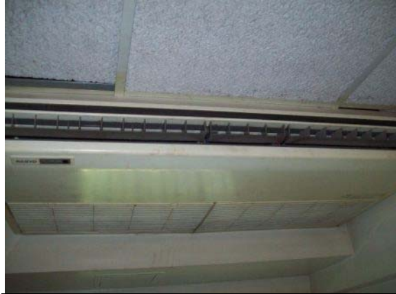
Photo #44: Split system fan coil unit
