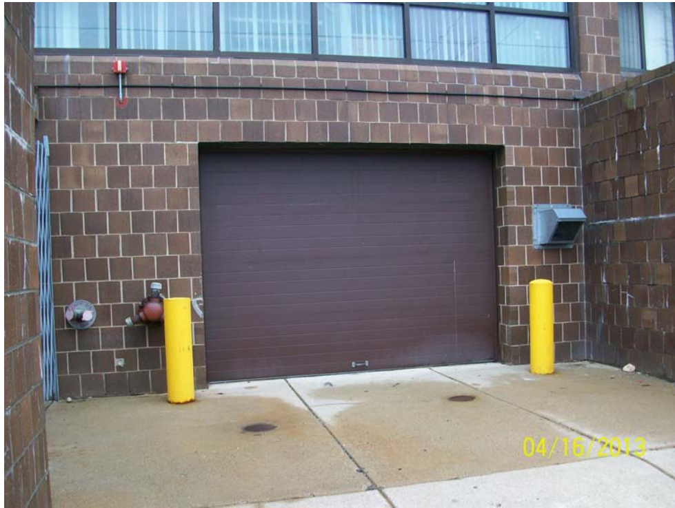
Photograph 9: Overhead door from the basement on the west side of the building.
