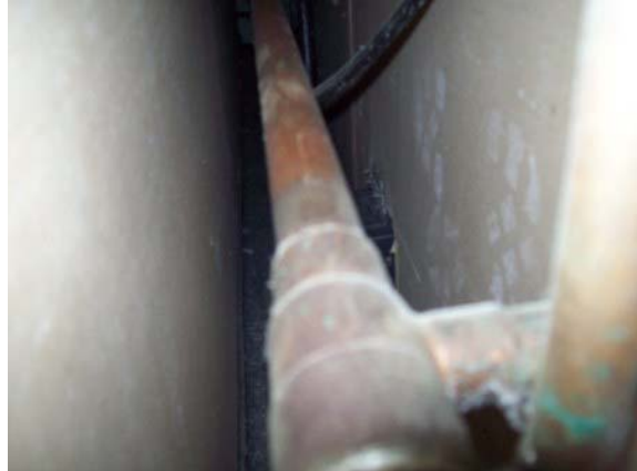
Photo #50: Domestic water piping
