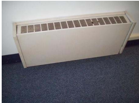
Photo #46: Supplemental heating unit for corridor
