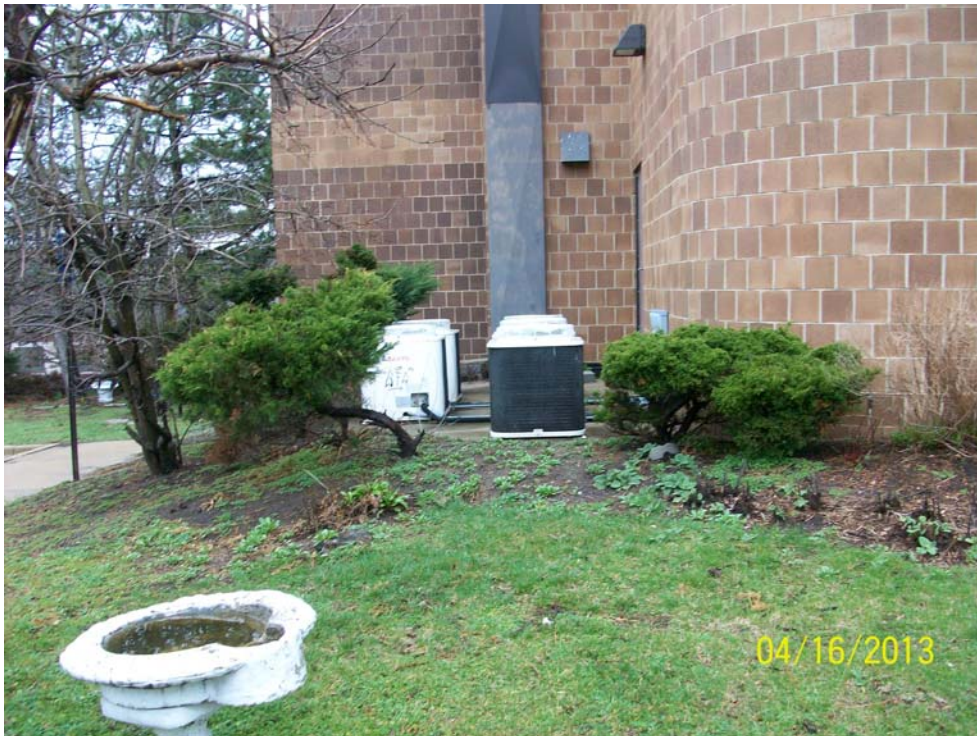
Photograph 6: Air conditioning units observed on the north side of the building.
