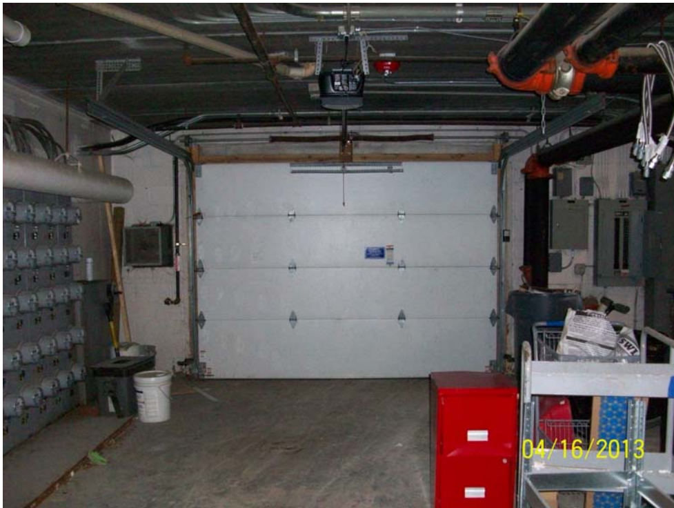
Photograph 16: Electrical panels and overhead door observed on the west side of the basement of the building.
