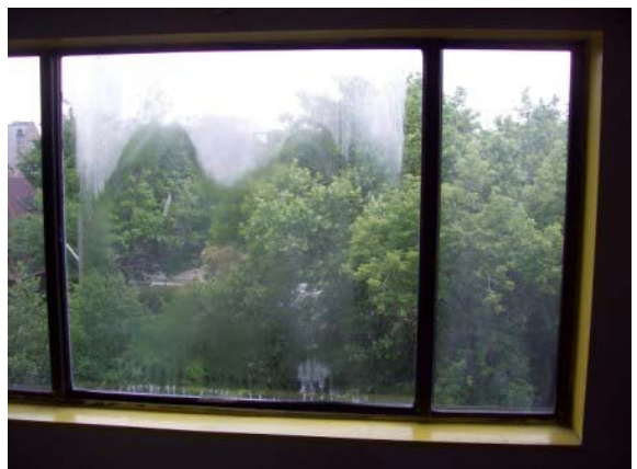
Photo #12: Failed thermal seal in unit window
