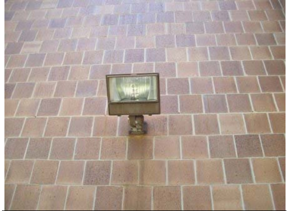
Photo #74: Exterior building-mounted lighting
