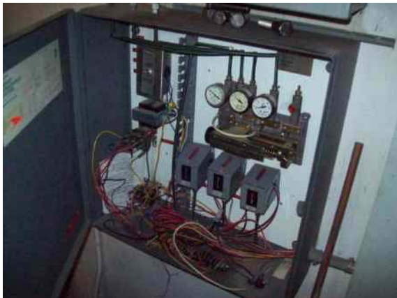
Photo #47: Pneumatic control unit
