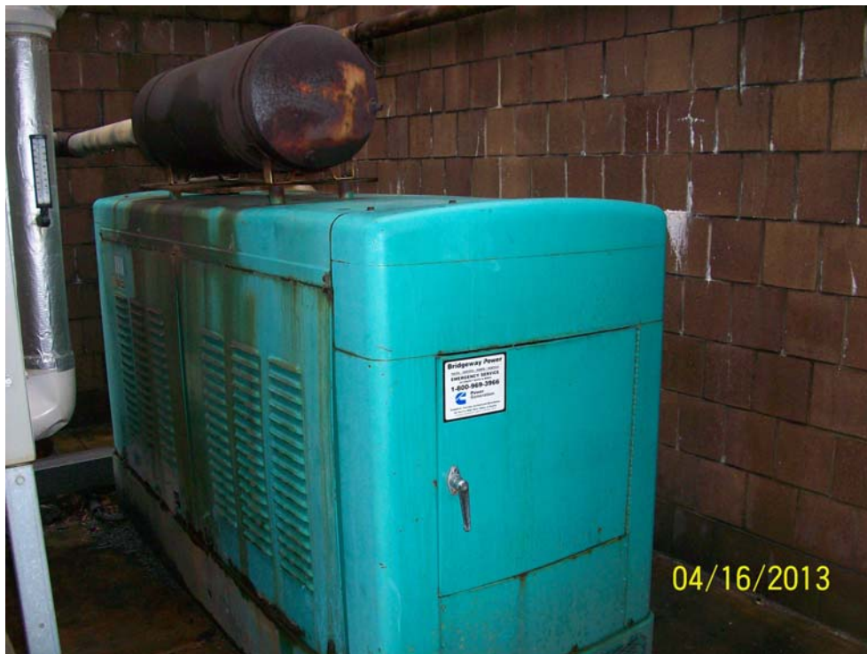
Photograph 22: Emergency generator observed within a brick storage area (holding chillers and the emergency generator, and above ground storage tank) on the west side of the building.
