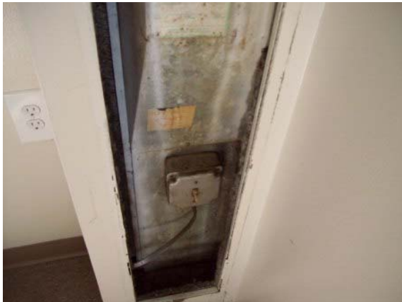
Photo #33: Fan coil unit for apartment
