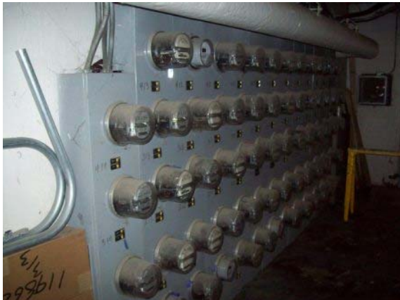
Photo #57: Tenant electric meters
