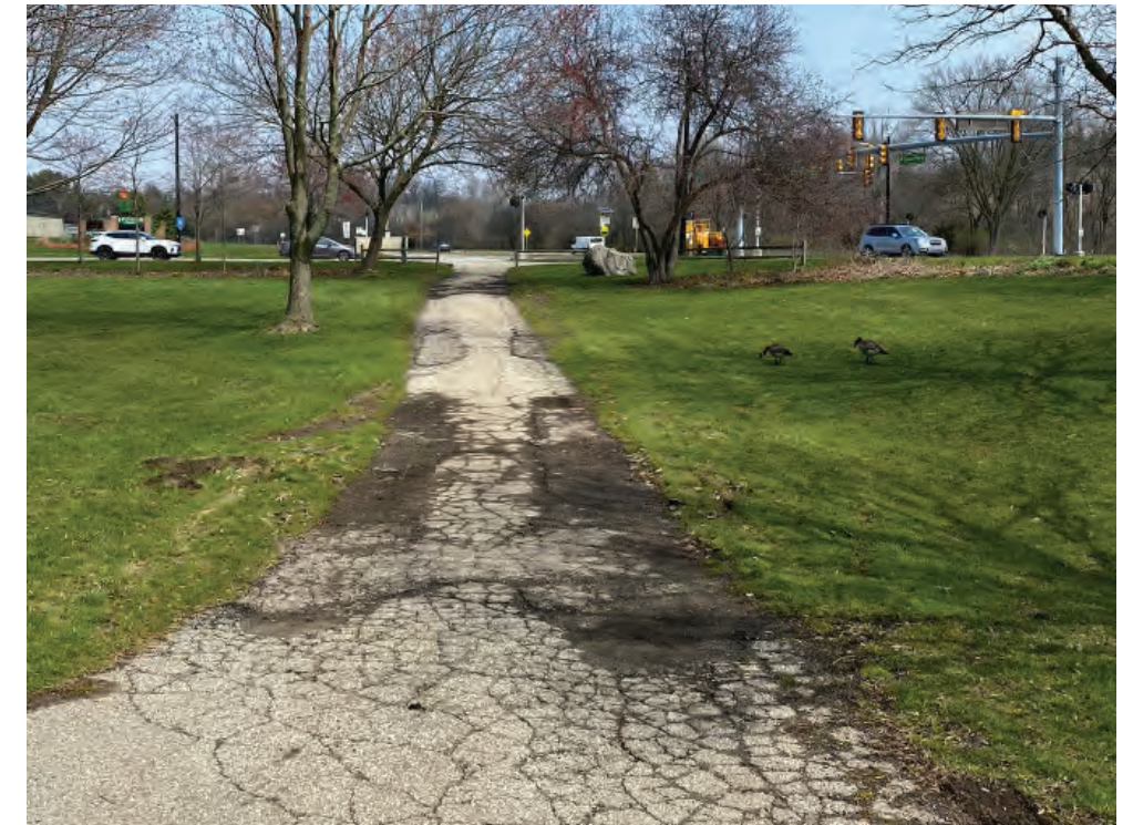
EXISTING 6' WIDE ASPHALT PATH CONNECTING TO HURON PARKWAY AND FULLER ROAD (WEST OF BRIDGE).
