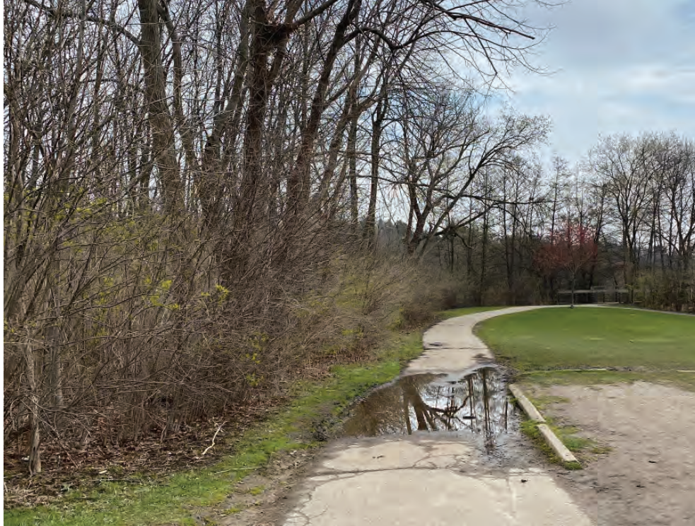
FLOODING BY BOAT LAUNCH - ELEVATION NEEDS TO BE RAISED HERE TO PROMOTE POSITIVE DRAINAGE.
