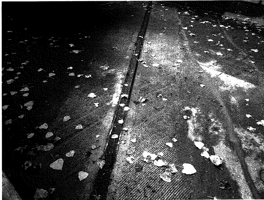
Photograph No. 13 Dirt and Debris in Deck Joint
