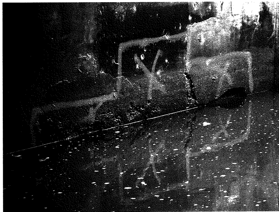
Photograph No. 42 Spalling and Delaminations Water line on Southwest Side of Pier
