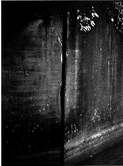
Photograph No. 35 Spalling at East Abutment and South Wingwall
