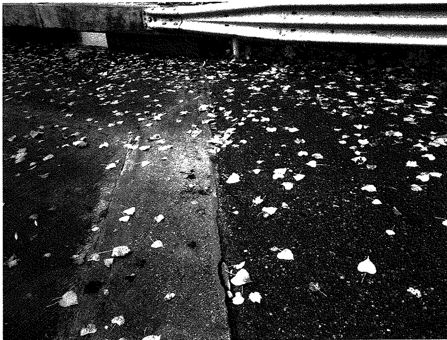
Photograph No. 15 Concrete Delaminations along West Reference Line
