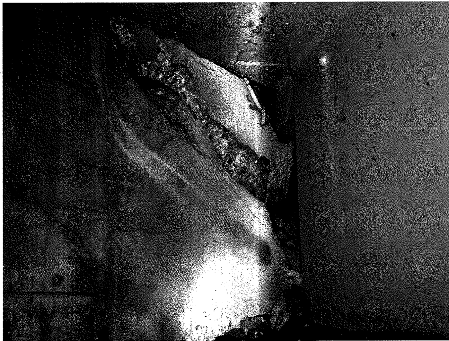
Photograph No. 36 Spalling and Cracking at Southeast Corner of East Backwall
