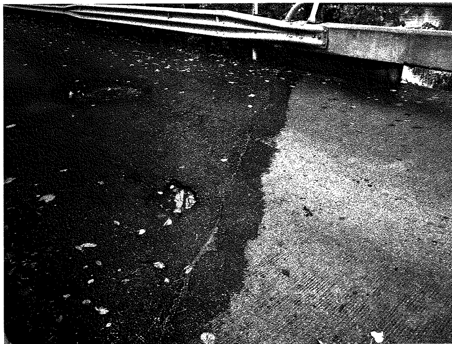
Photograph No. 16 Cracking and Pothole in Approach Pavement near East Reference Line
