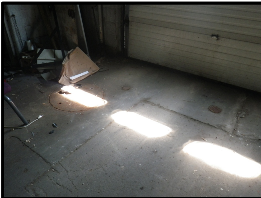
Sump/skimmer for oil UST inside the maintenance garage
