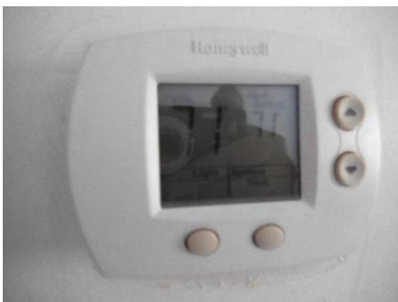
Photo 5: Digital Honeywell Thermostat
