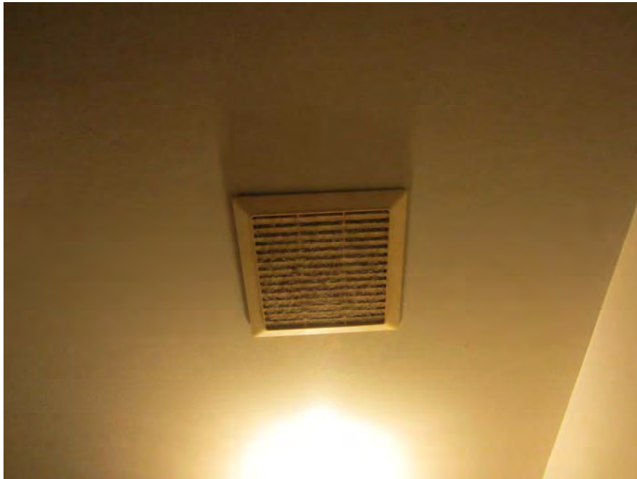
PHOTOGRAPH NO. 12: EXHAUST FAN IN TENANT UNIT 749 BATHROOM
