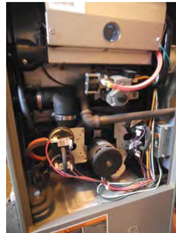
Photo 14: Interior of gas-fired furnace
