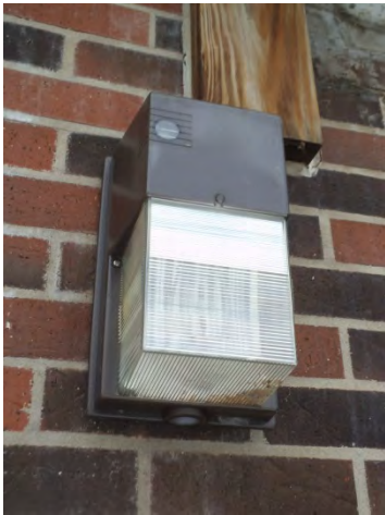
Photo 3: Wall-Mounted Exterior Lighting
