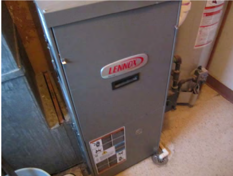
PHOTOGRAPH NO. 9: TYPICAL VIEW OF FURNACES IN TENANT UNITS (749)
