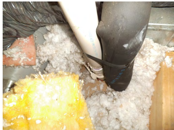
Photo 12: Insulation on piping
