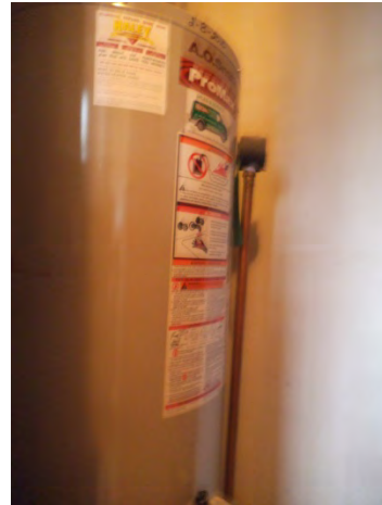
Photo 12: Domestic Hot Water Heater per Unit
