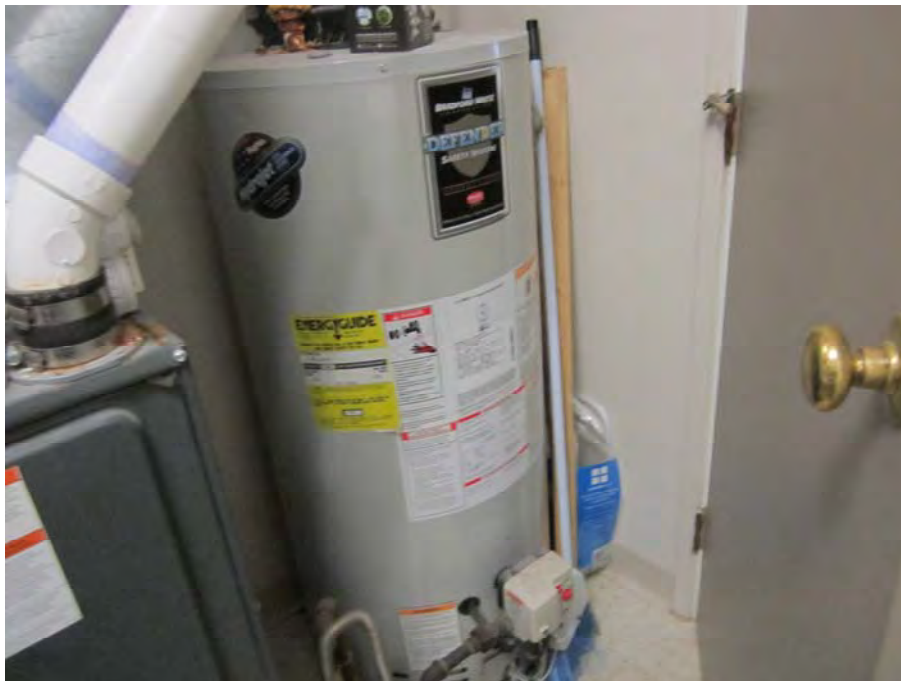
PHOTOGRAPH NO. 8 VIEW OF HOT WATER HEATER IN UNIT 743
