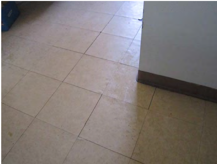
PHOTOGRAPH NO. 14: TENANT UNIT 749 WATER DAMAGED HALLWAY FLOORING
