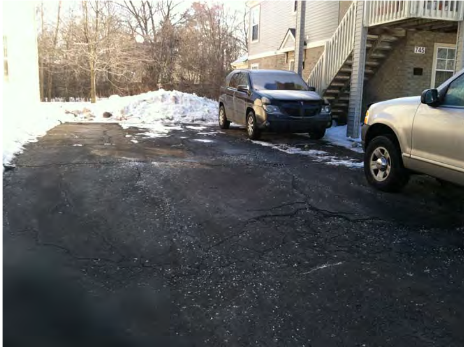
PHOTOGRAPH NO. 5: CLOSE UP OF DETERIORATED AREA IN PARKING LOT
