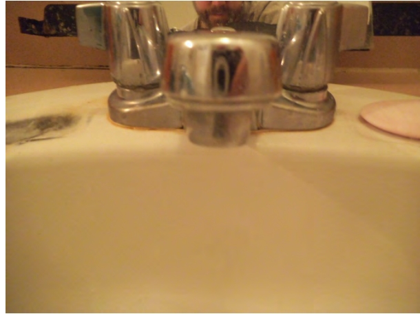
Photo 8: Typical Bathroom Sink Faucet
