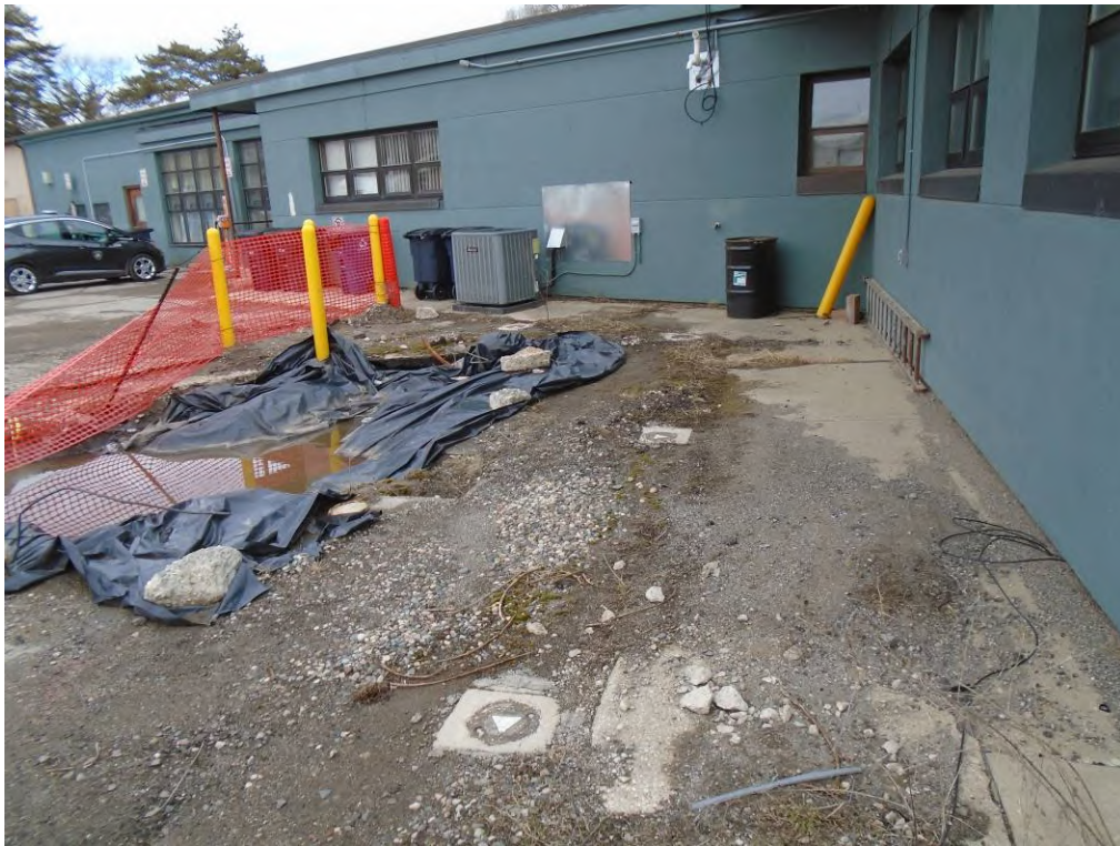
Photo 4: View of the former heating oil UST excavation, groundwater monitoring wells, and 55-gallon drum located within the northeastern parking lot portion of the 2000 South Industrial Highway subject property, facing north.
