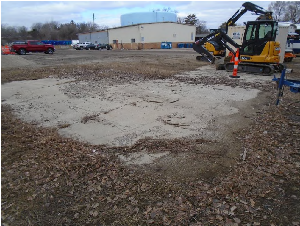
Photo 38: View of the southeastern portion of the subject property, former glass refuse bins concrete pad, facing northwest.
