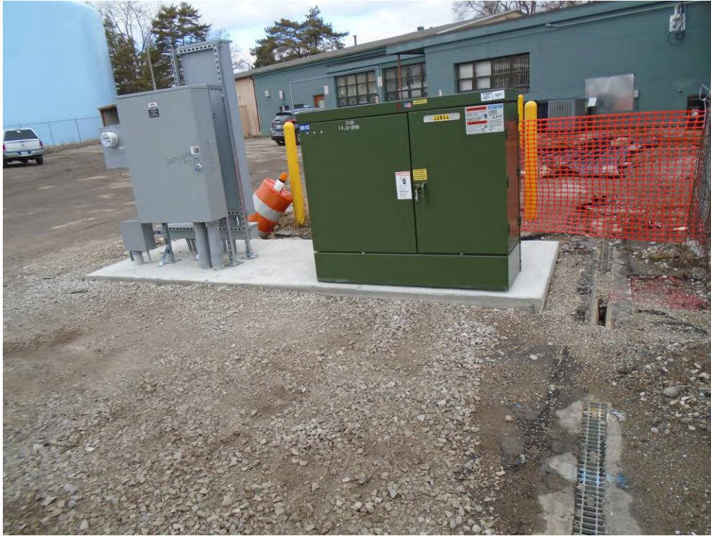
Photo 3: View of a pad-mounted electrical transformer and trench drain located within the northeastern parking lot portion of the 2000 South Industrial Highway subject property, facing north.
