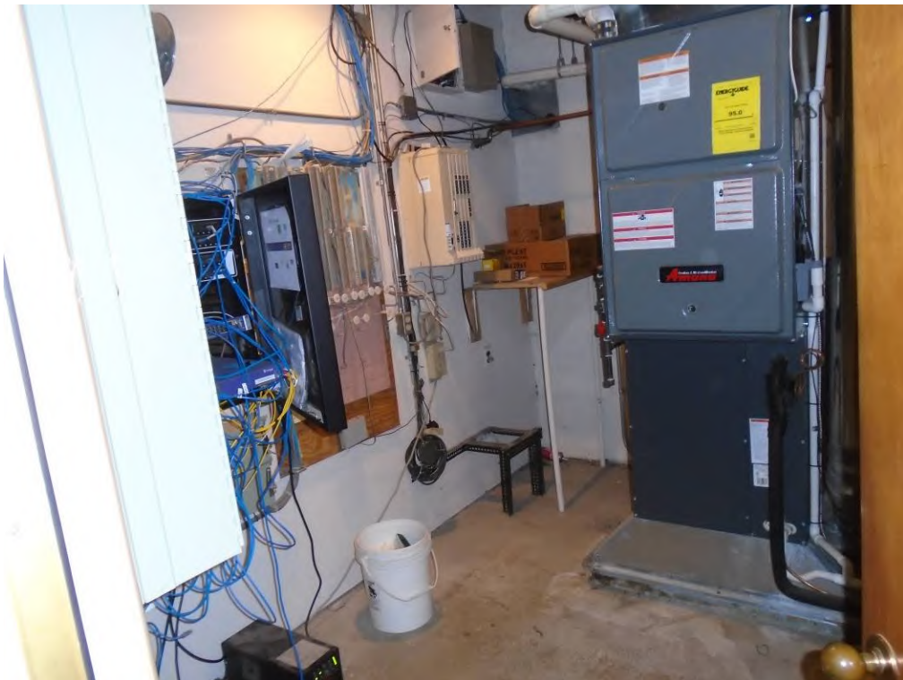
Photo 10: View of the 2000 South Industrial Highway subject property building mechanical room with potential floor access point of the former heating oil UST.
