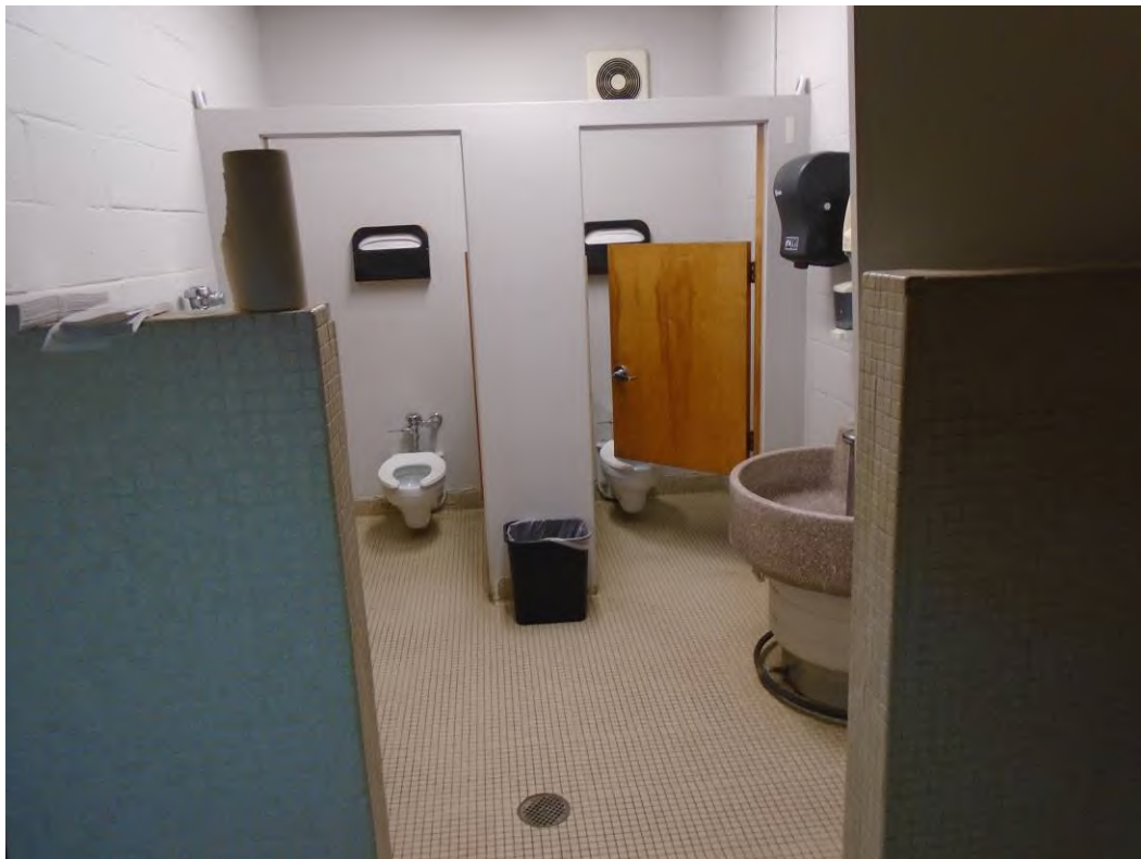
Photo 8: View of the 2000 South Industrial Highway subject property building restroom with floor drain.
