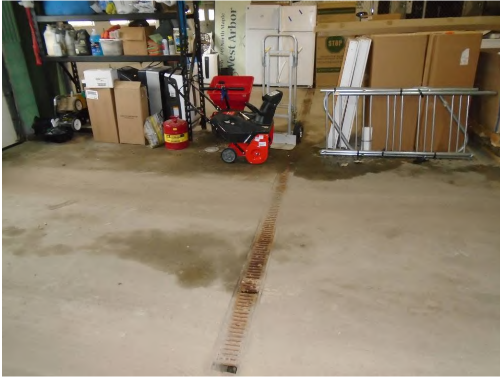
Photo 23: View of trench drain within the drain commission warehouse space within the 2050 South Industrial Highway subject property building.
