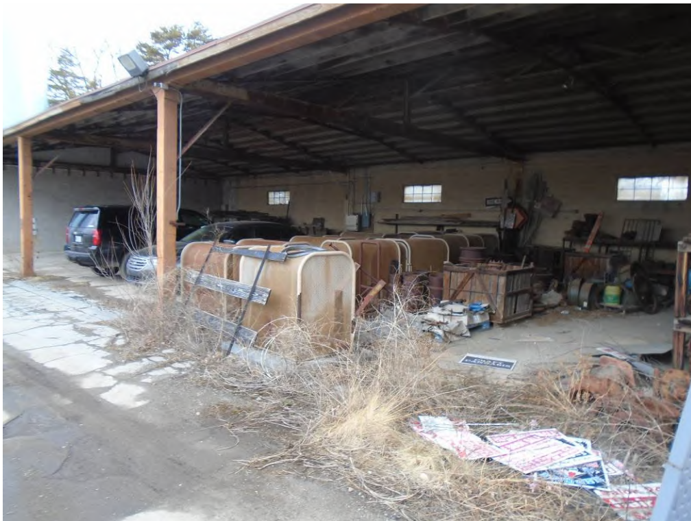
Photo 6: View of the western portion of the 2000 South Industrial Highway subject property building, facing northwest.
