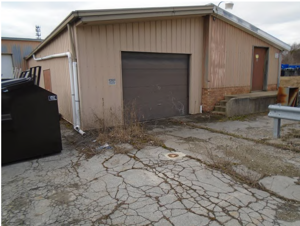
Photo 32: View of the secure unassessed Fire Department evidence room warehouse space within the 2050 South Industrial Highway subject property building at left.
