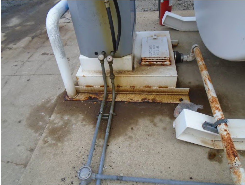
Photo 17: View of dispenser staining associated with the 15,000-gallon diesel AST.
