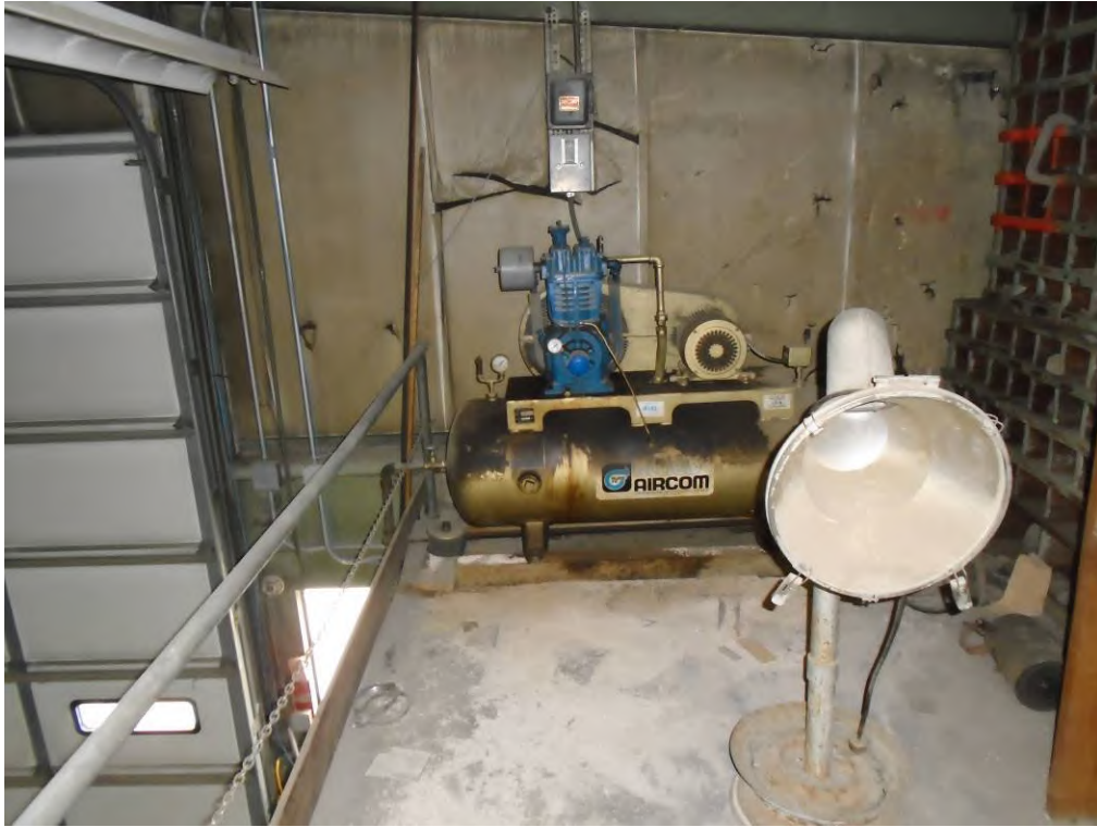
Photo 29: View of air compressor within the CTN TV mezzanine warehouse space within the 2050 South Industrial Highway subject property building.
