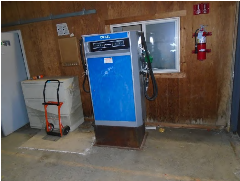
Photo 28: View of diesel fuel dispenser within the CTN TV warehouse space within the 2050 South Industrial Highway subject property building.
