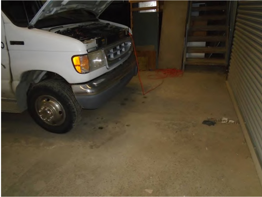
Photo 27: View of trench drain and floor patching within the CTN TV warehouse space within the 2050 South Industrial Highway subject property building.
