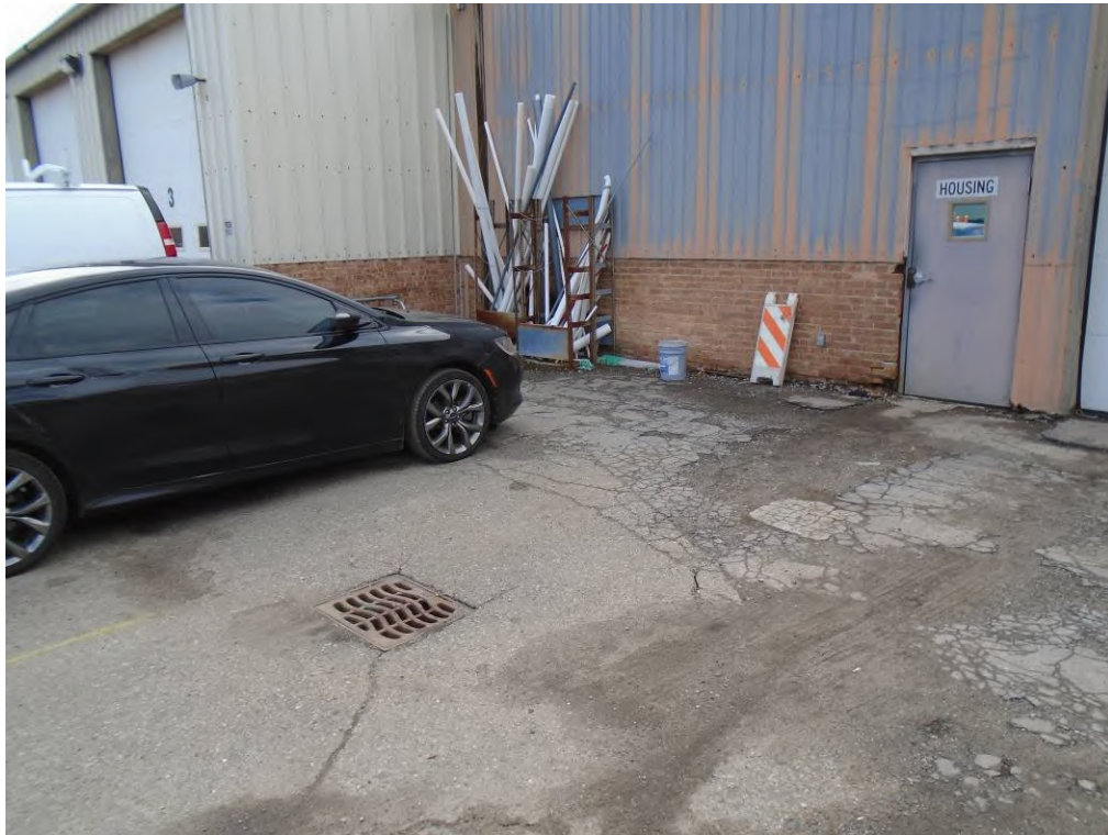
Photo 13: View of the northern entrance of the 2050 South Industrial Highway subject property building, facing southeast. Note the stormwater catch basin and area of petroleum odor at entry door.
