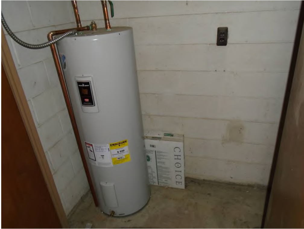
Photo 9: View of the 2000 South Industrial Highway subject property building hot water heater closet with floor drain.
