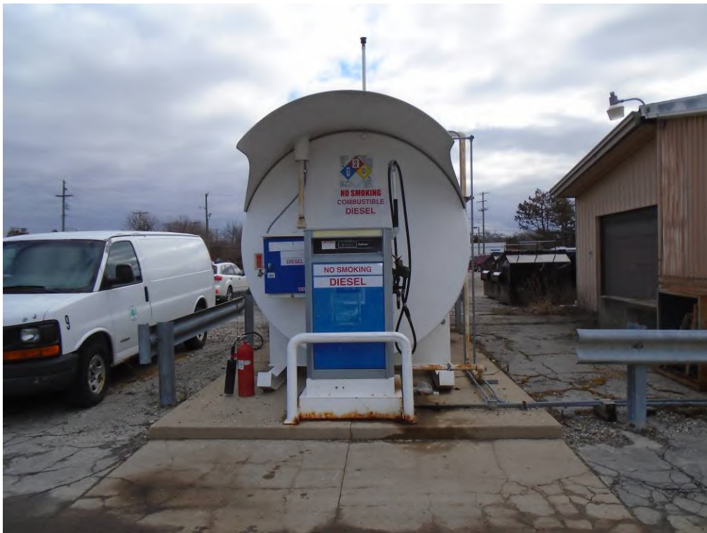
Photo 16: View of 15,000-gallon diesel fuel AST, facing east. Note the staining present at the dispenser.
