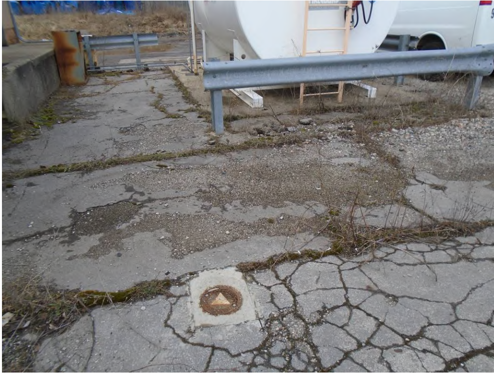
Photo 15: View of the monitoring well associated with the 15,000-gallon diesel fuel AST.
