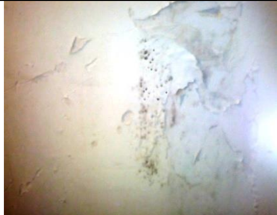
Photo #24: Unit 3681 water damage in basement
