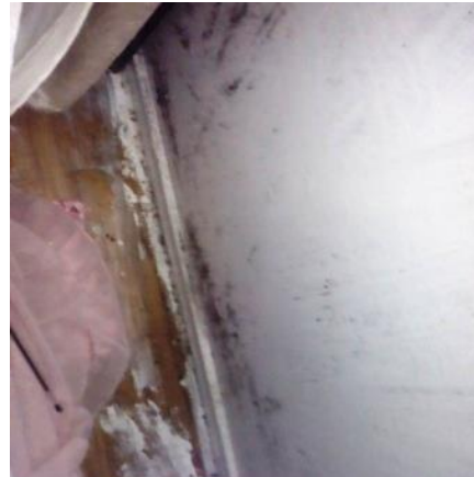
Photo #26: Unit 3681 Moisture damage in bedroom 1
