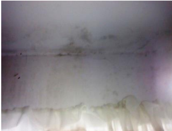
Photo #25: Unit 3681 Water damage in bathroom
