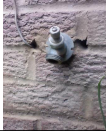
Photo #32: Potential entry point for pests.
