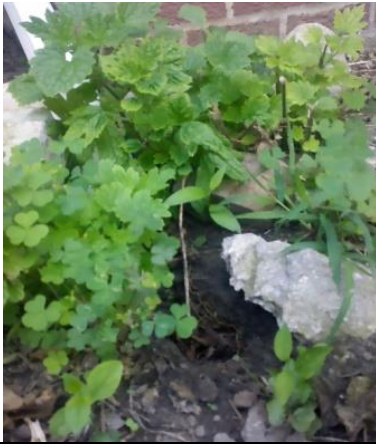
Photo #31: Bottom of downspout missing. Water pools against foundation here.
