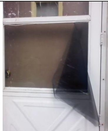
Photo #34: Damaged screen should be replaced to prevent pest entry.
