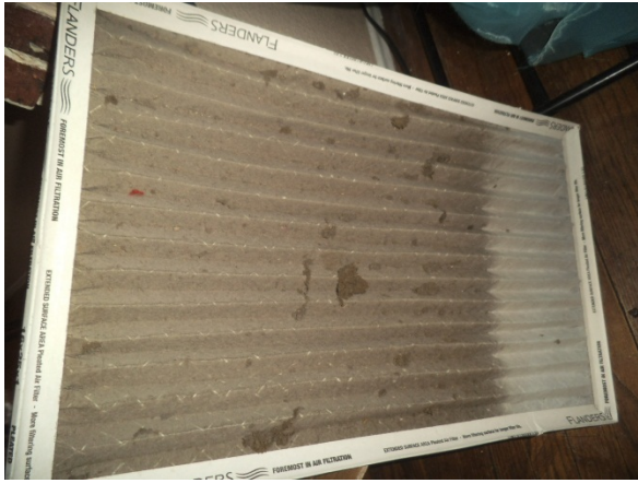
Photo 13: Old furnace filter
