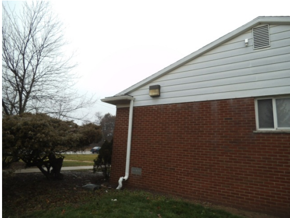
Photo 3: Exterior wallpack on side of complex
