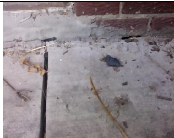
Photo #36: Expansion joints between concrete slabs and building should be sealed to prevent pest issues.
