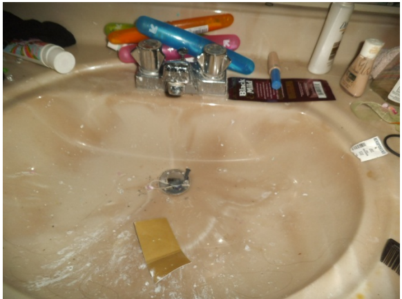
Photo 14: Bathroom faucet with aerator
