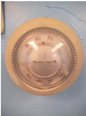
Photo 15: Manual thermostat in community center
