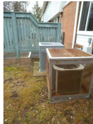
Photo 16: Community center condensing unit
