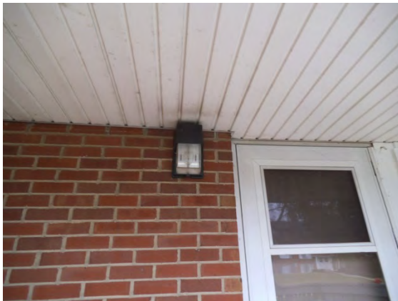
Photo 5: Exterior wall-pack near each entrance
