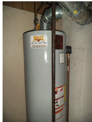
Photo 28: DHW tank in Community Center
