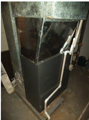
Photo 28: Furnace in community center basement
