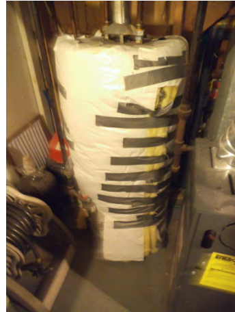
Photo 14: Insulated DHW storage tank
