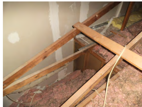
Photo 18: Minimal insulation in some areas
