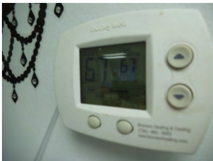
Photo 23: Digital thermostat in community center
