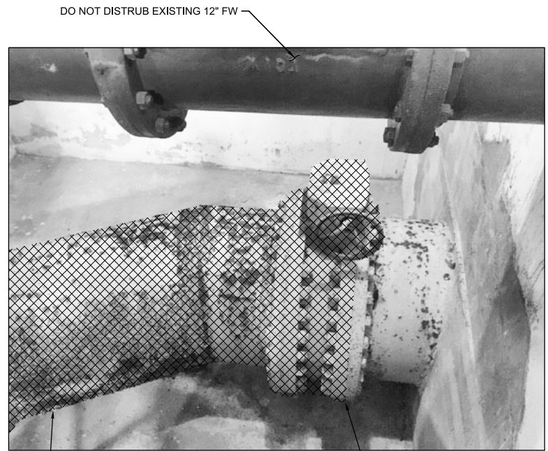
8 PHOTO NTS 020-X-121 2 DEMOLISH EXISTING 30" CLEARWELL INTERCONNECT PIPE 2 DEMOLISH VALVE AT FLANGE
