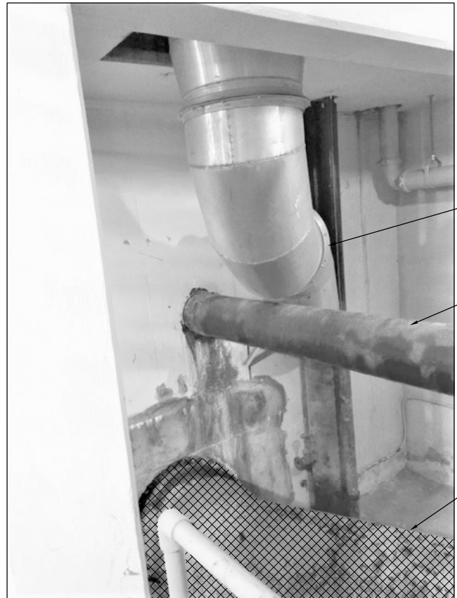
9 PHOTO NTS 020-X-121 2 DEMOLISH EXISTING 30" CLEARWELL INTERCONNECT PIPE DO NOT DISTURB EXISTING 12" FW CONTRACTOR TO REMOVE FAN PRIOR TO DEMOLITION OF EXISTING 30" CLEARWELL INTERCONNECT PIPE. REINSTALL FAN AND REALIGN AS NECESSARY FOLLOWING CONSTRUCTION OF NEW 30" CLEARWELL INTERCONNECT PIPE
