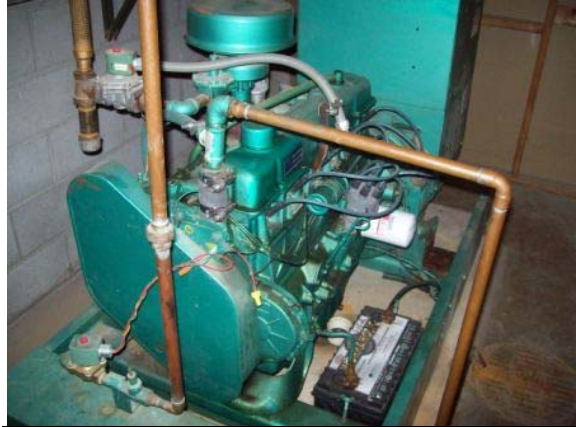
Photo #44: Emergency generator
