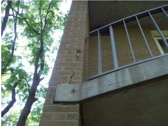
Photo #69: Cracking at southwest corner of building
