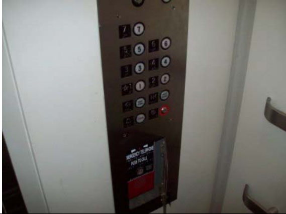
Photo #49: Elevator control panel
