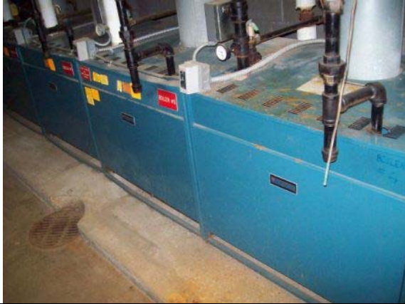
Photo #25: Set of four modular boilers
