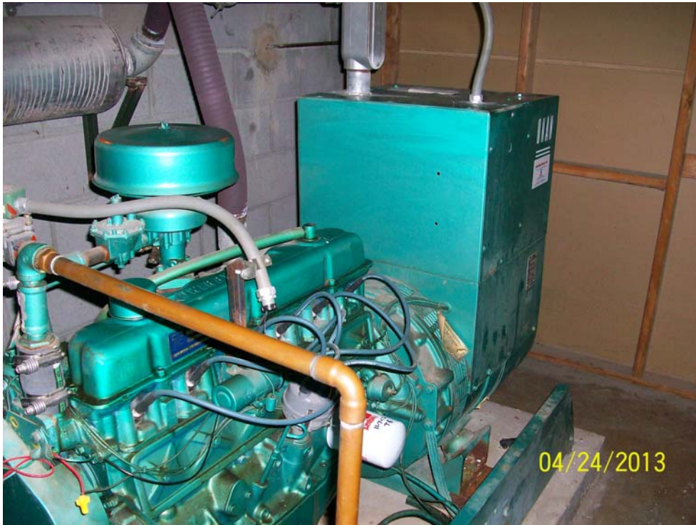
Photograph 13: Natural gas fired emergency generator observed in the southeast corner of the first floor of the apartment building.
