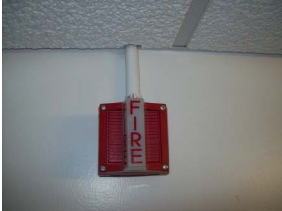
Photo #55: Fire alarm horn with strobe light
