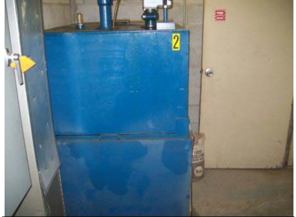
Photo #50: Hydraulic elevator equipment
