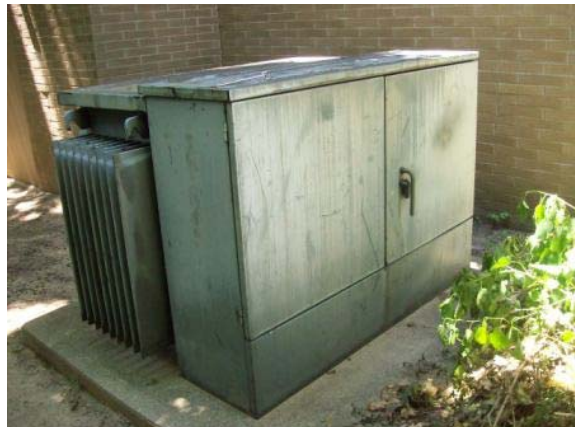
Photo #42: Electrical transformer
