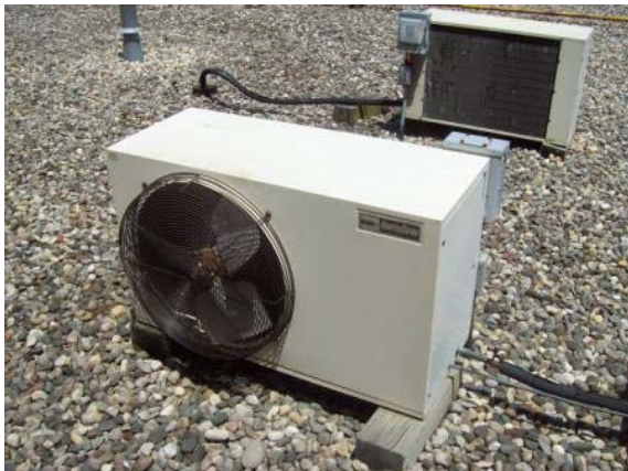
Photo #35: Split system condensing units for lobby
