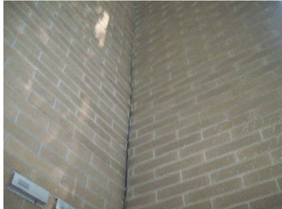
Photo #70: Cracking at stairwell near west end of building
