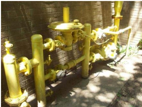
Photo #41: Gas meter and regulator
