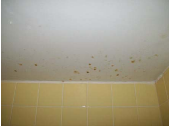
Photo #67: Water staining on ceiling near office area
