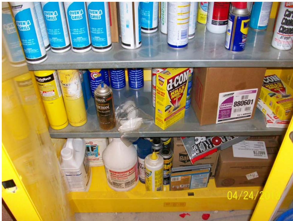
Photograph 24: Maintenance chemical storage in the north side addition to the building.
