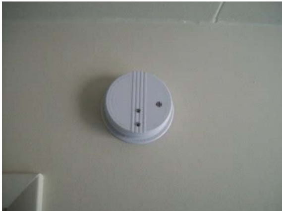
Photo #57: Smoke detector in resident unit
