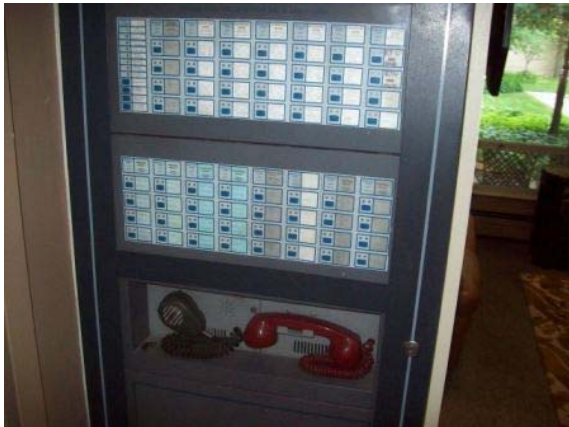
Photo #51: Fire alarm panel
