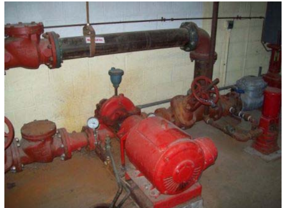
Photo #52: Fire pump
