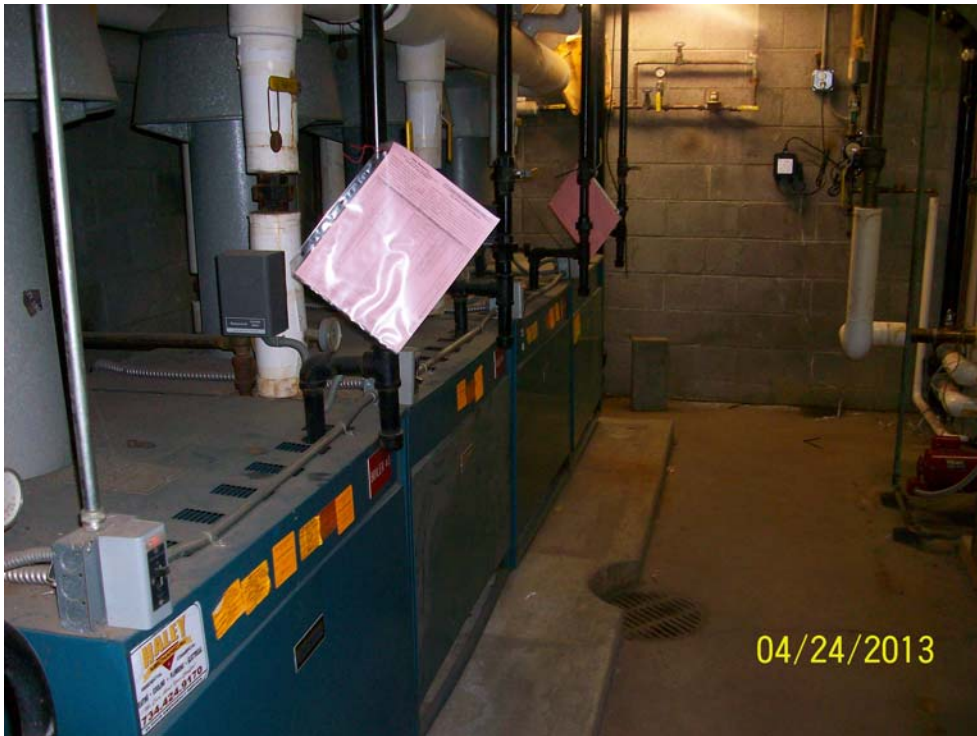
Photograph 14: Furnaces observed in the first floor of the apartment building.
