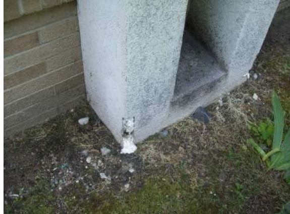
Photo #68: Damage to EIFS finish at office area
