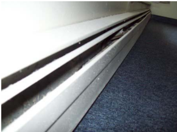
Photo #29: Typical baseboard finned-tube heating unit
