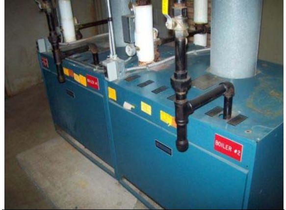
Photo #26: Set of two modular boilers
