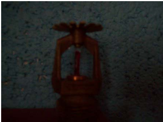
Photo #53: Sprinkler head
