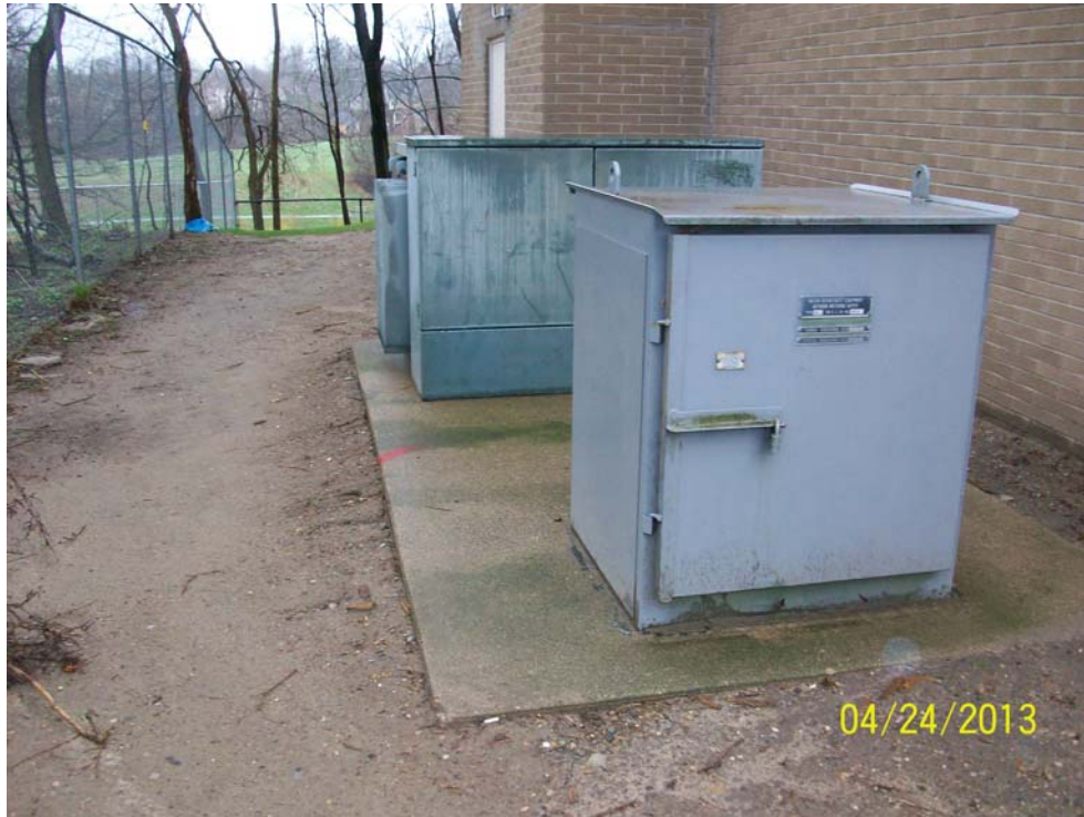
Photograph 5: Pad-mounted transformer and switch gear box observed on the east side of the apartment building.
