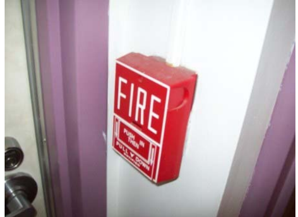
Photo #56: Fire alarm pull station
