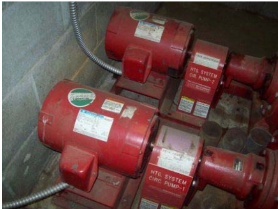
Photo #27: Heating water circulating pumps
