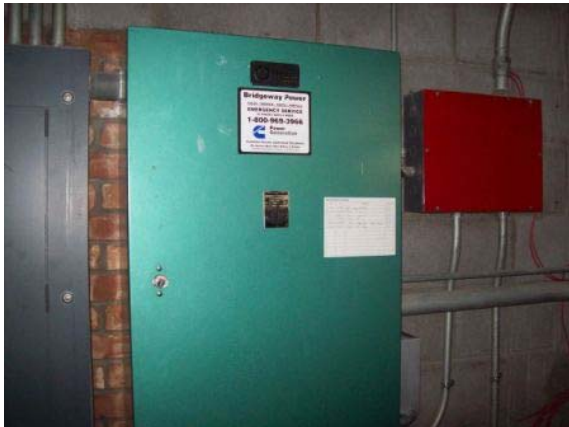
Photo #45: Emergency power transfer switch
