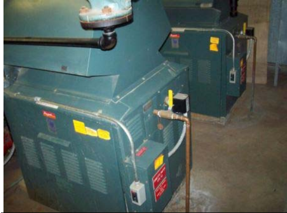
Photo #38: Domestic water boilers
