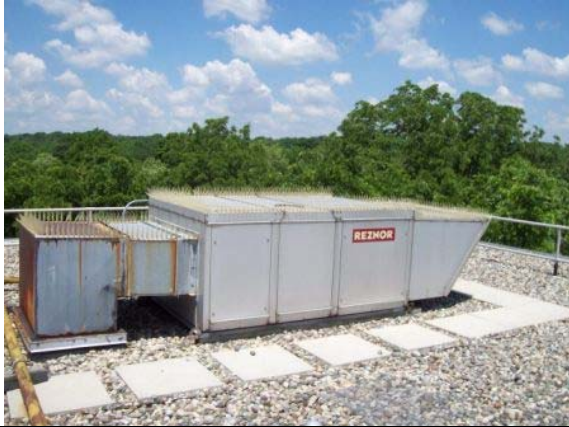
Photo #31: Make-up air unit for corridors
