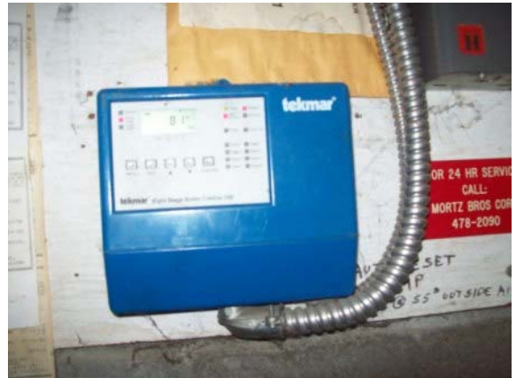
Photo #28: Boiler control module
