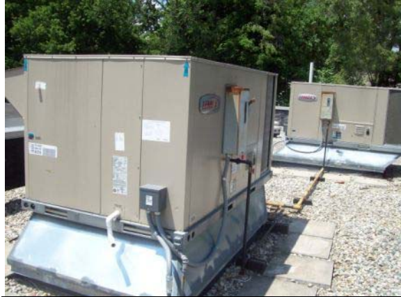
Photo #32: Rooftop units for office spaces
