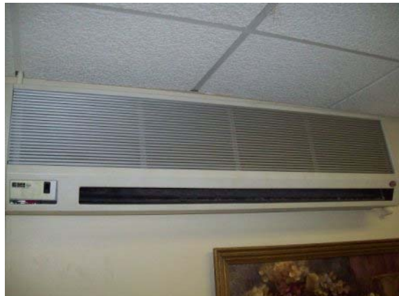
Photo #36: Wall-mounted fan coil units for lobby
