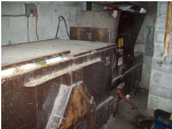
Photo #65: Trash compactor
