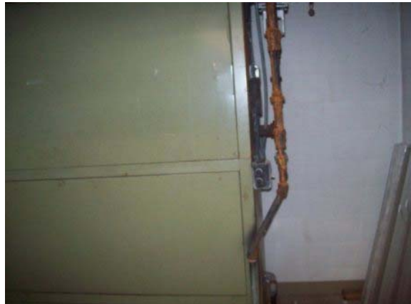
Photo #34: Split system fan coil unit and furnace for community room
