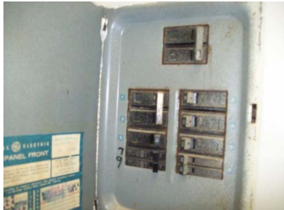
Photo #46: Resident unit breaker panel
