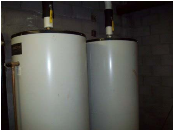
Photo #39: Domestic hot water storage tanks
