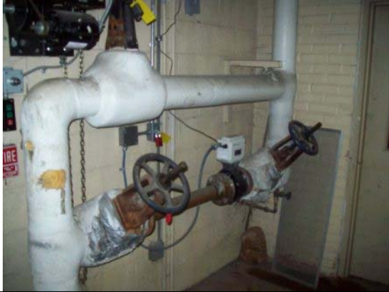
Photo #37: Domestic water meter
