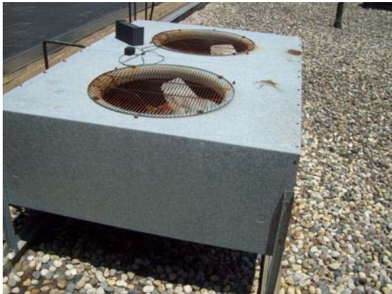
Photo #33: Split system condensing unit for community room
