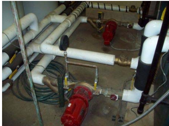
Photo #40: Domestic hot water circulating pumps
