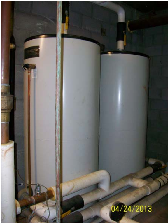
Photograph 15: Water heaters observed in the first floor of the apartment building.
