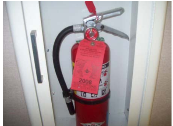
Photo #54: Fire extinguisher
