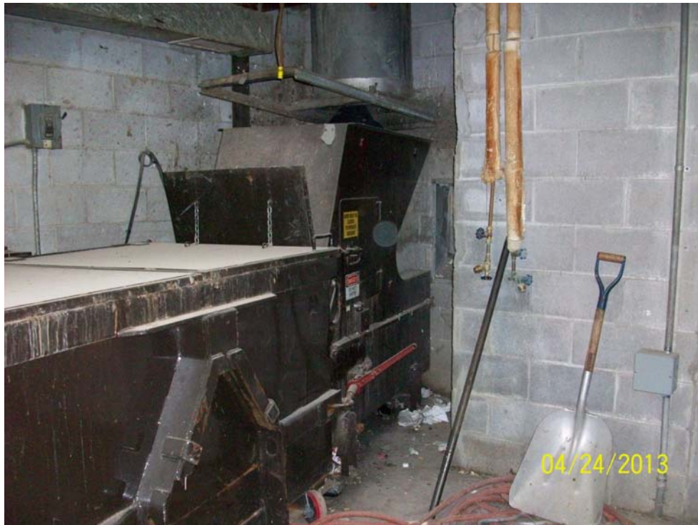
Photograph 12: Trash compactor in the first floor of the apartment building.
