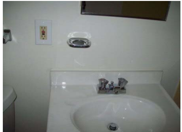
Photo #58: GFCI in resident unit
