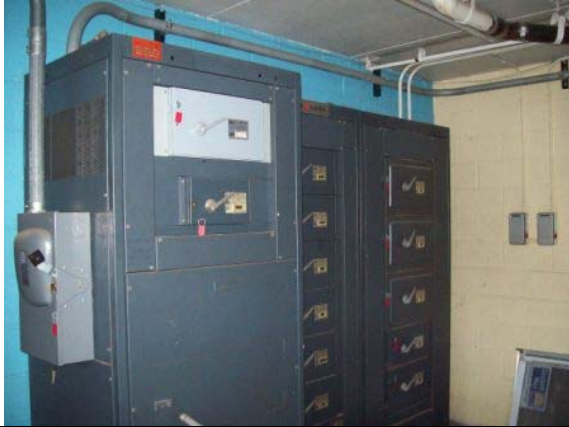
Photo #43: Main electrical switchgear
