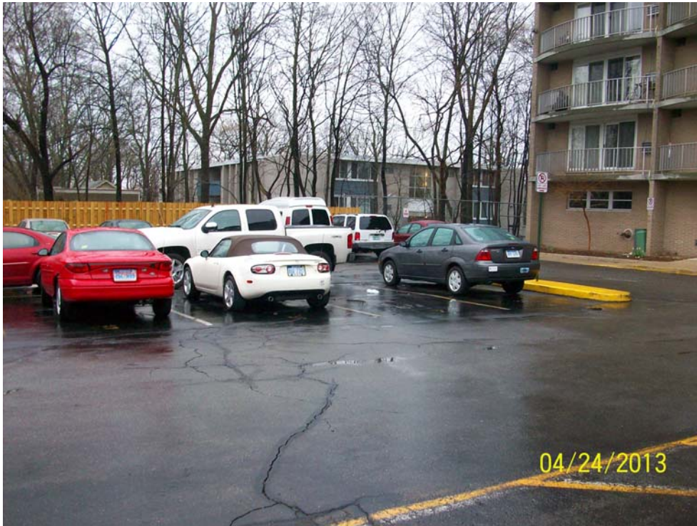
Photograph 3: Asphalt parking lot observed on the northeast portion of the Subject Property.
