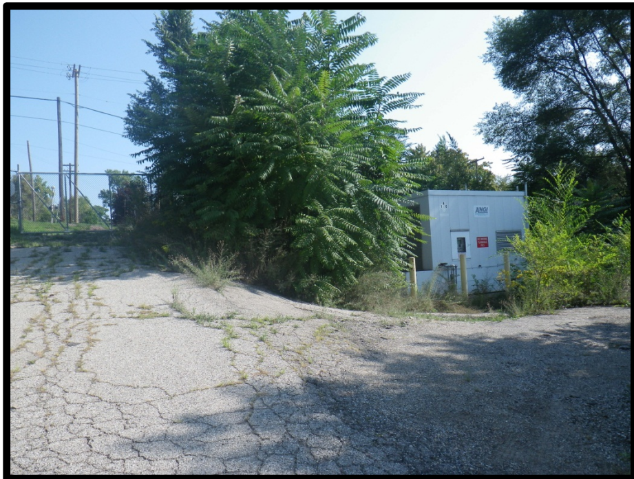
Looking north at the compressed natural gas compressor
