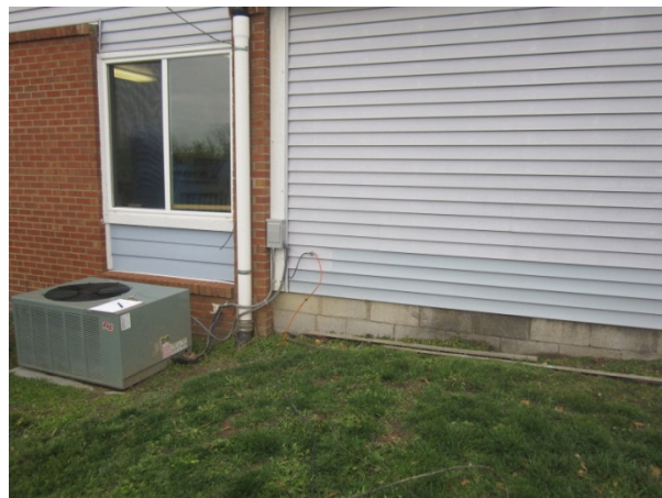
Photo 12: Condensing unit for Community Center
