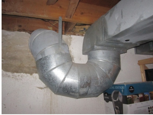
Photo 14: Ducting from the furnace
