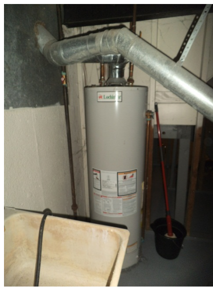
Photo 24: Typical hot water heater in residential unit
