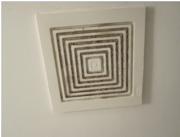
Photo 9: Typical bathroom exhaust fan
