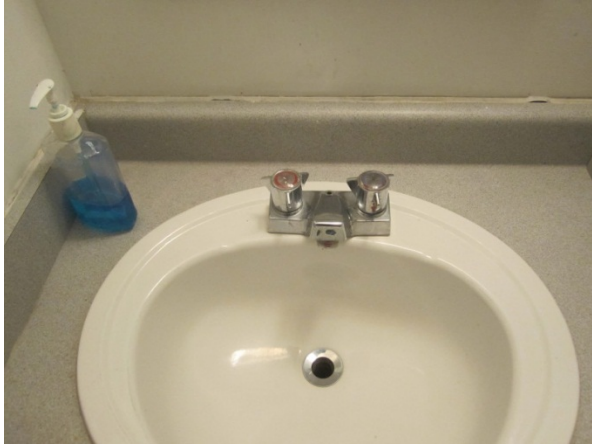
Photo 7: Typical bathroom faucet and sink
