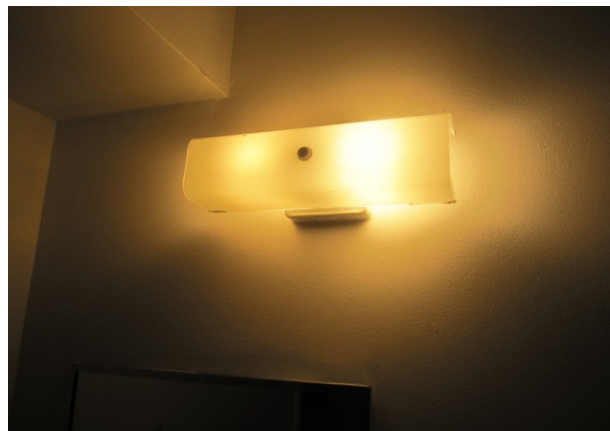
Photo 6: Typical bathroom lighting fixture
