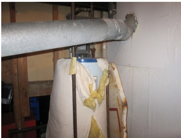
Photo 17: Slightly insulated hot water heater
