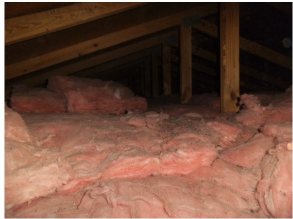
Photo 22: Batt insulation in attic space
