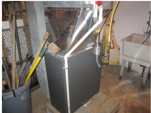
Photo 16: Typical furnace in basement
