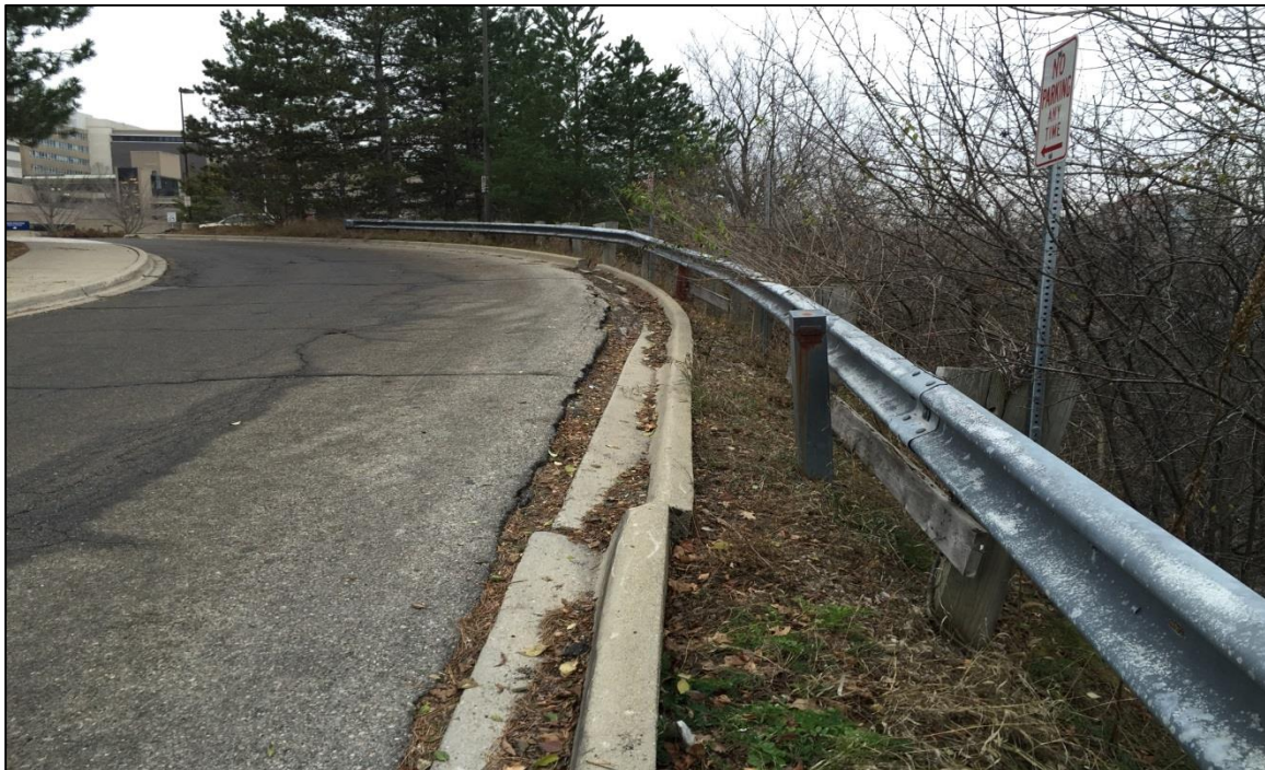
PHOTO NO. 1B – December 12, 2015: Looking west along the north curb line of Nichols Drive. Inclinometer I-2 is also visible in this photo between the guardrail and the curb line.
