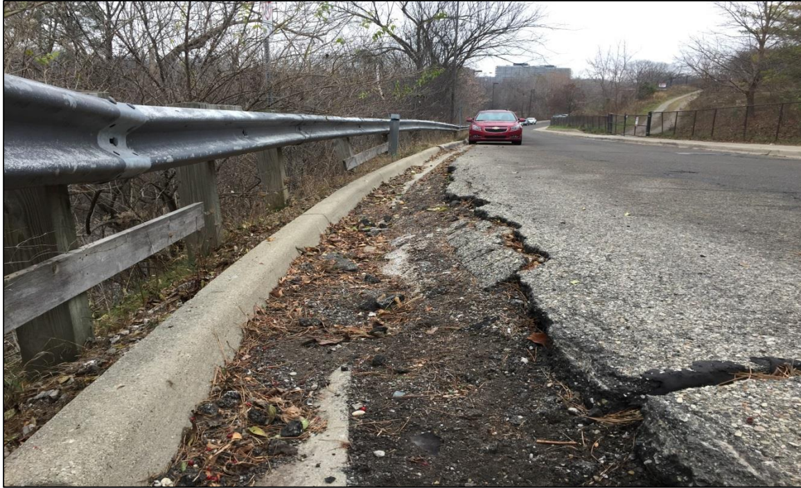
PHOTO NO. 7: Close-up of the drop in the pavement surface along the north curb line of Nichols Drive. Inclinometer I-1 is located immediately to the left of this location.
