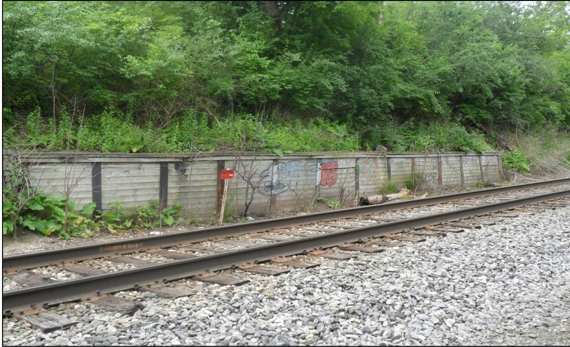
PHOTO NO. 4A – June 11, 2010: Looking at the soldier pile retaining wall at the toe of the slope on the south side of the railroad line.
