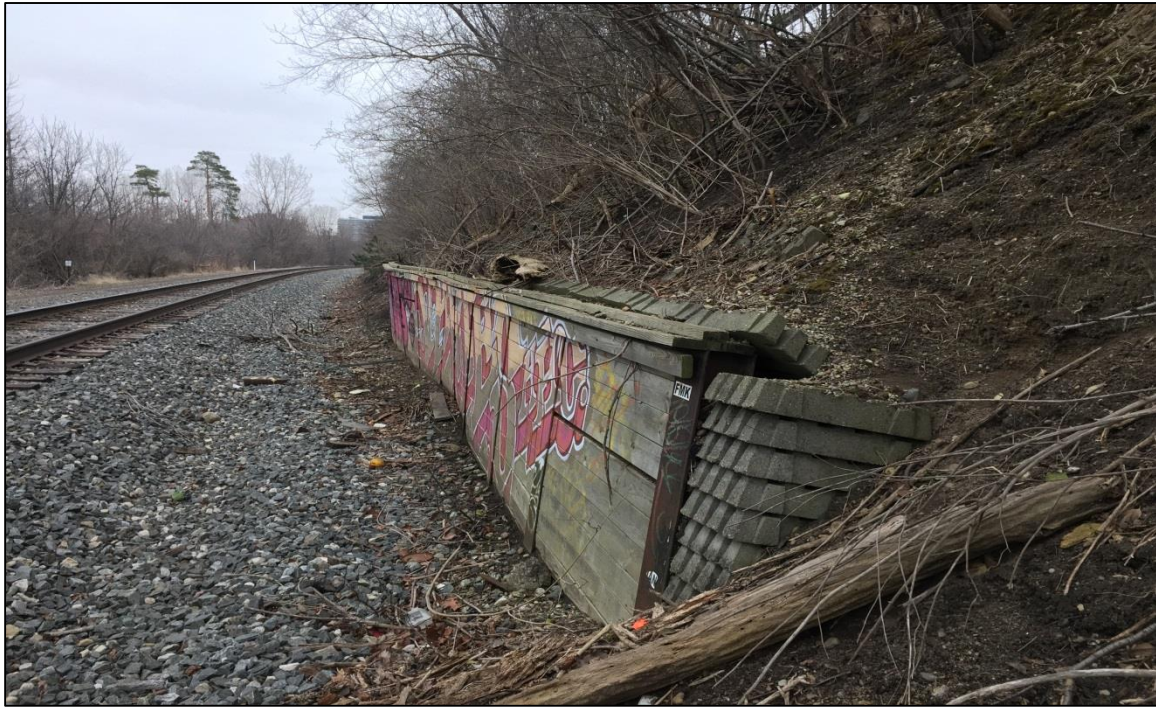
PHOTO NO. 11: Looking east at the soldier pile retaining wall at the toe of the slope.
