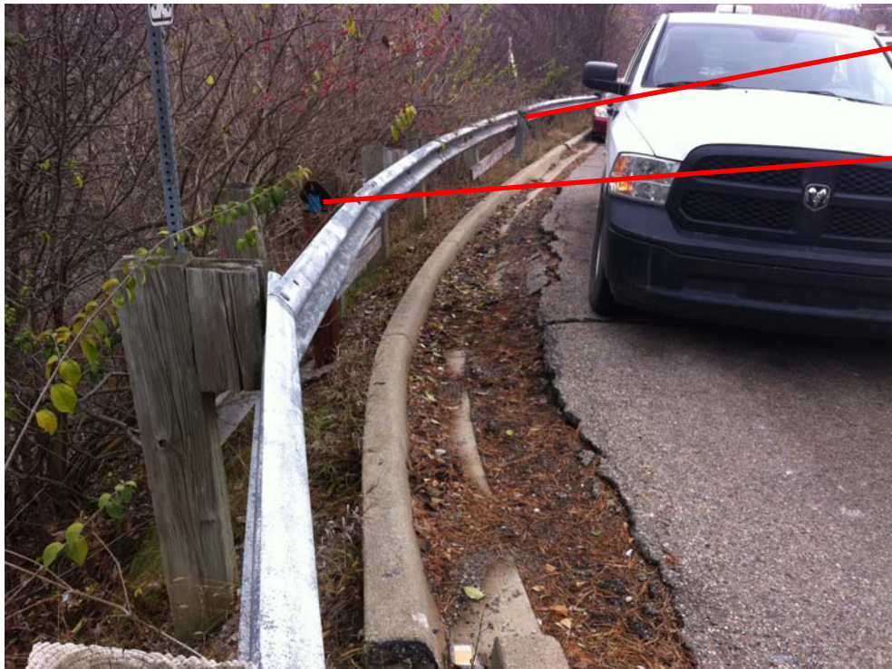
2015 Looking east, toward inclinometers I-1 and I-2
