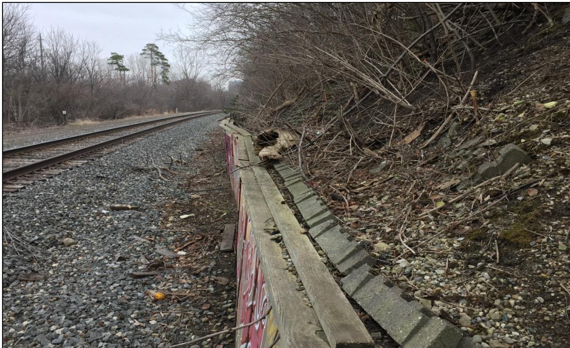
PHOTO NO. 12: Looking east along the top of the soldier pile retaining wall at the toe of the slope.
