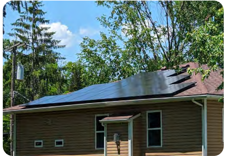
Solar panels installed through the Solarize Ann Arbor program this past year.
