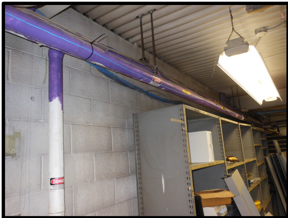
Asbestos wrap on piping in maintenance garage
