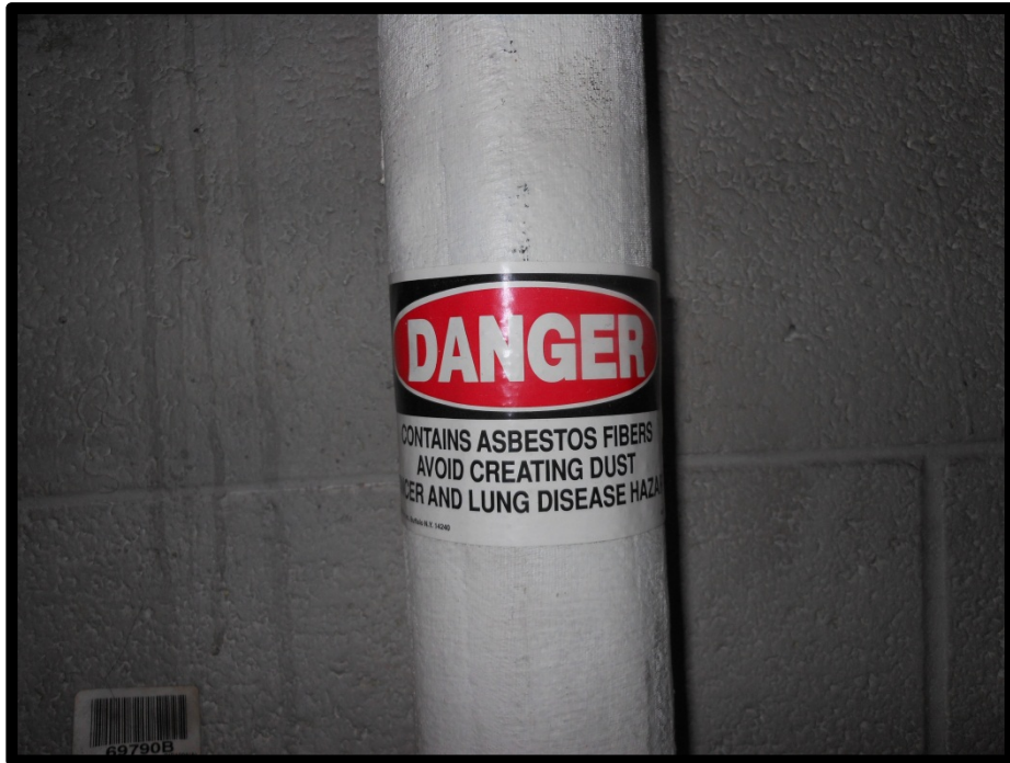
Asbestos wrap on piping in maintenance garage
