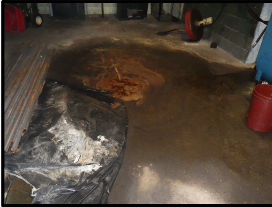
Staining on concrete in paint booth of maintenance garage
