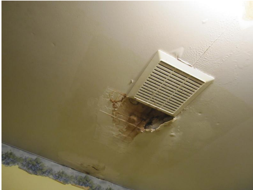
PHOTOGRAPH NO. 12: CEILING MOISTURE PROBLEM (UNIT 1020)
