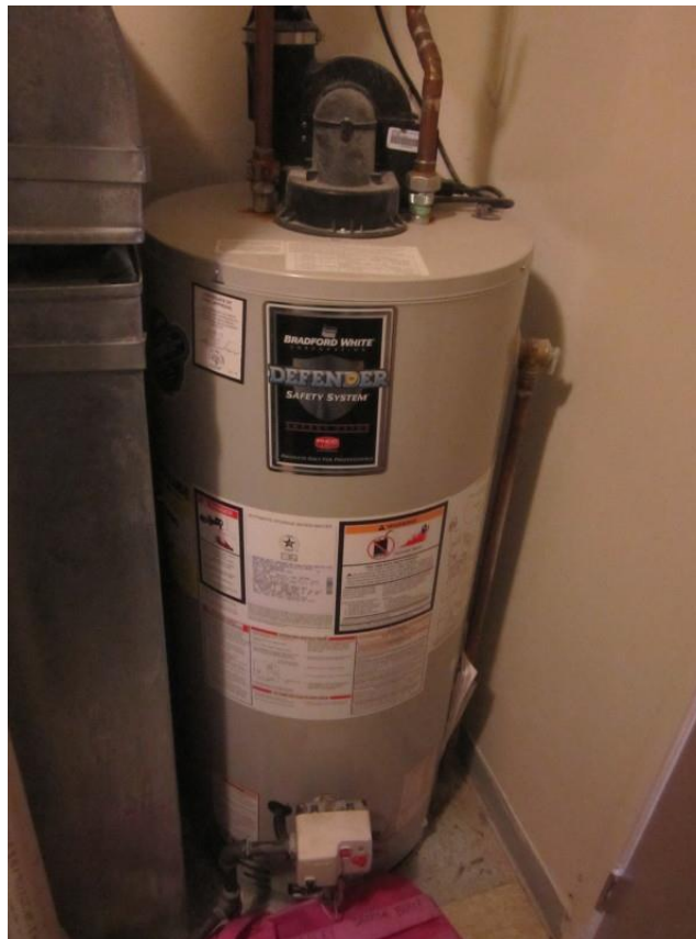
PHOTOGRAPH NO. 8 VIEW OF HOT WATER HEATER IN UNIT 1030
