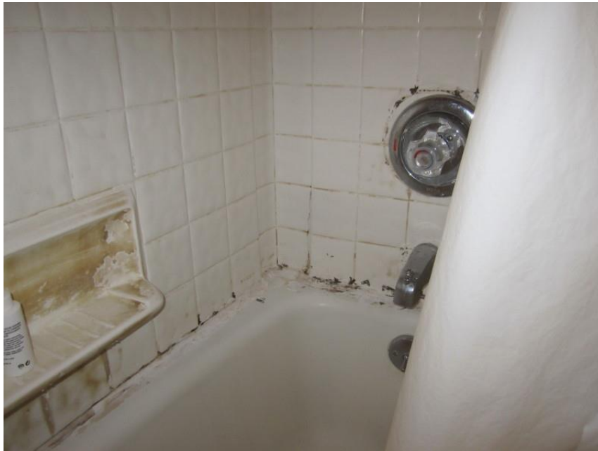
PHOTOGRAPH NO. 14: TENANT UNIT 1042 TUB AND ASSOCIATED VINYL ENCLOSURE
