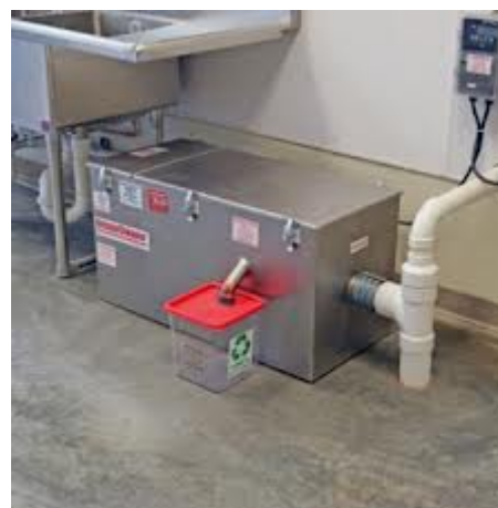
Figure 13: Typical Grease Accumulator near the kitchen sink
