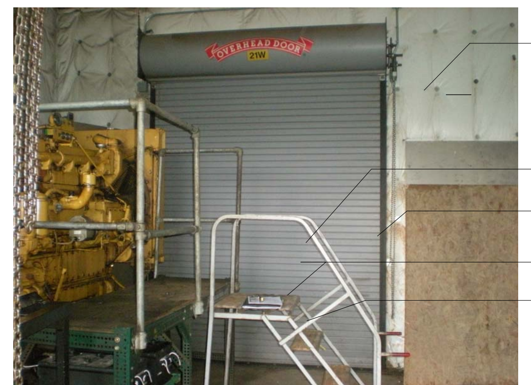
WELL HOUSE 21W - INTERIOR
