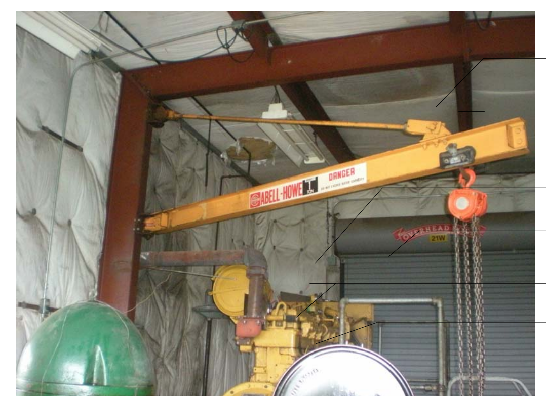
WELL HOUSE 21W - INTERIOR
