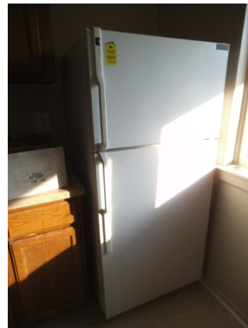
Photo 10: Typical unit refrigerator
