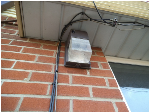
Photo 5: Typical exterior wall-mounted lights
