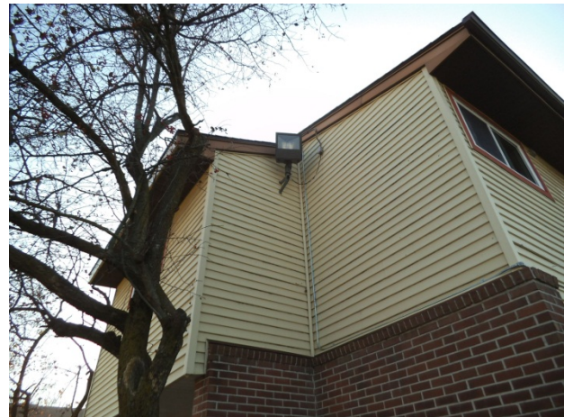
Photo 6: Typical exterior flood lights
