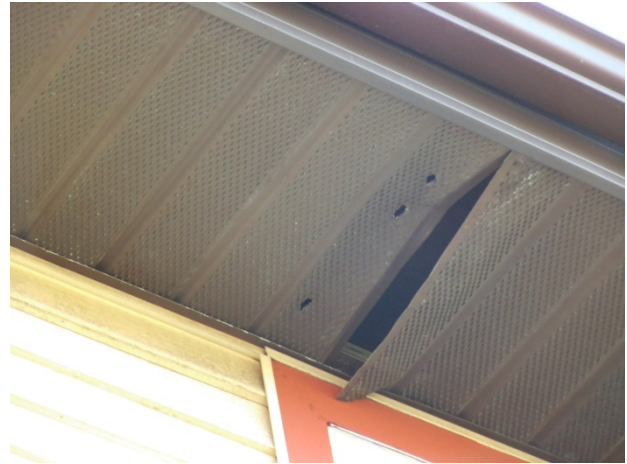
Photo 4: Broken soffit vents at complex
