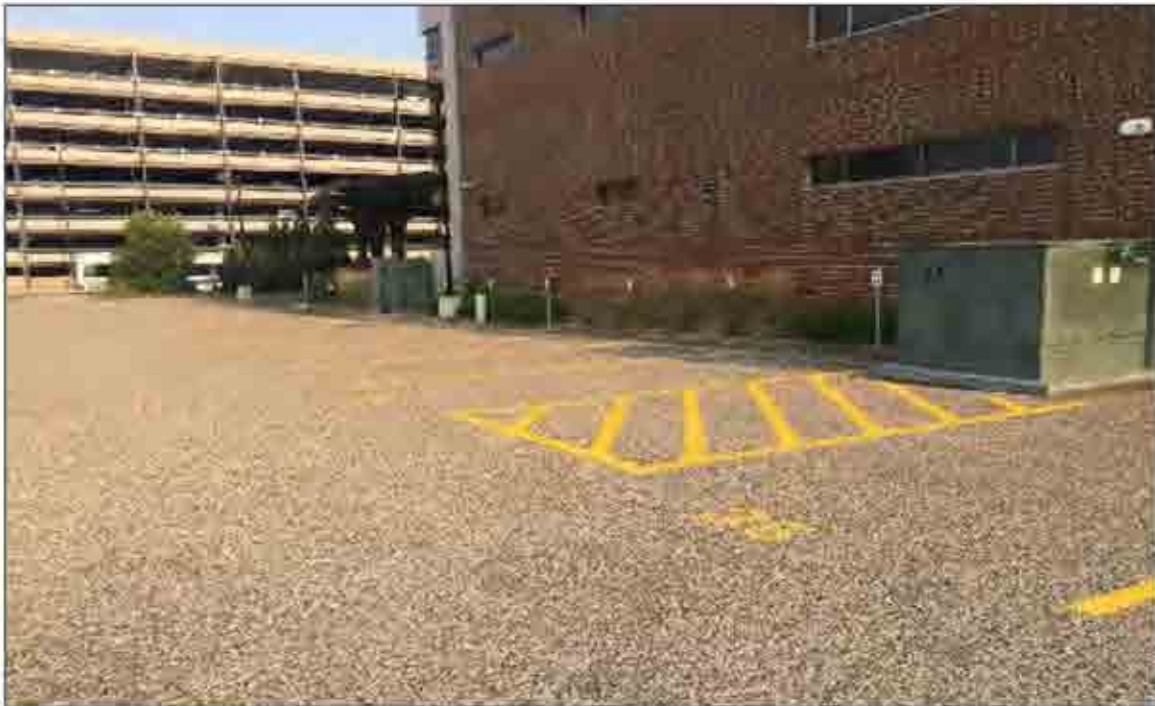
PHOTO NO. 6: Three concrete pad-mounted transformers along north side of the Property.
