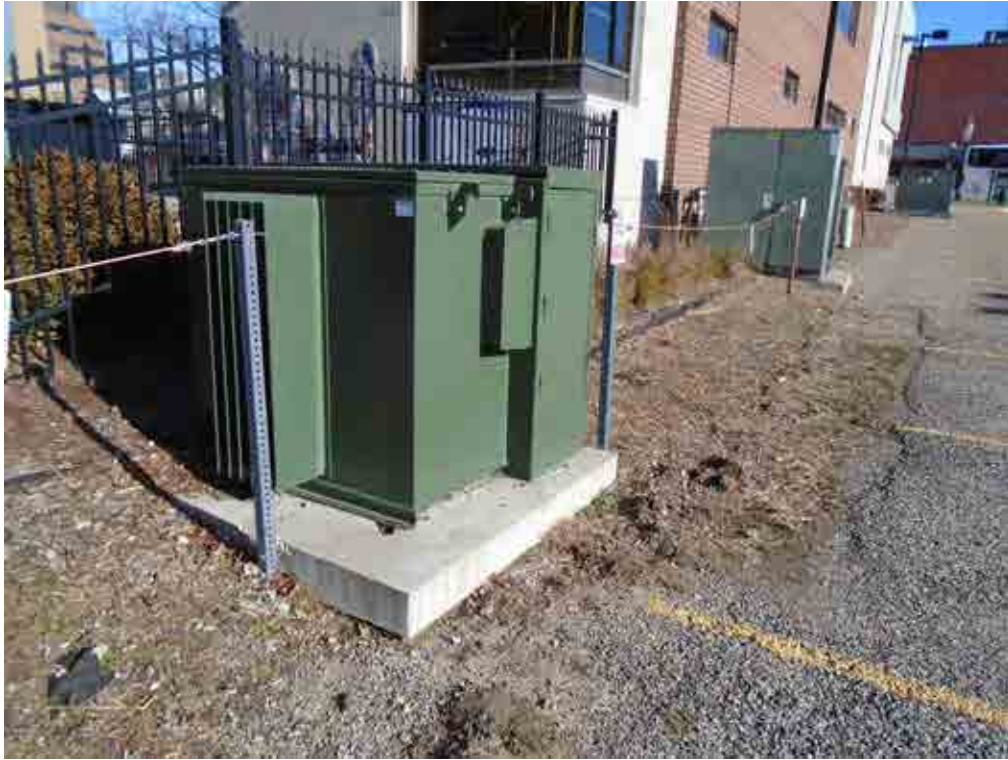
Photo 5: View of pad-mounted electrical transformers located along the northern Subject property boundary, facing east.
