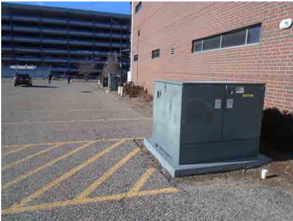
Photo 6: View of pad-mounted electrical transformers located along the northern Subject property boundary, facing west.
