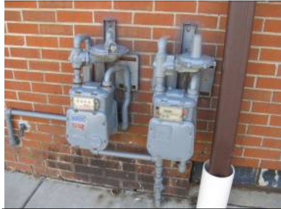
Photo #14: Gas meters and regulators
