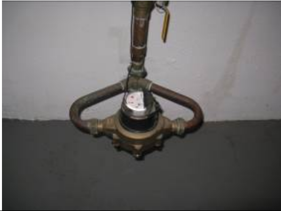
Photo #13: Water meter
