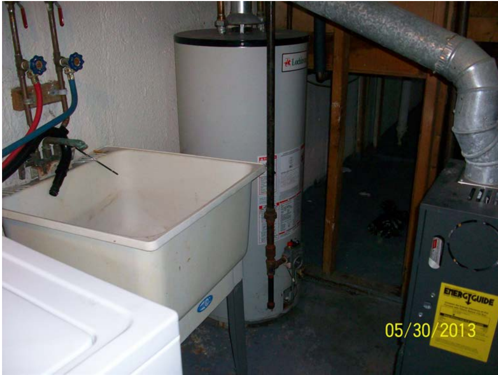
Photograph 13: Typical utility sink and water heater observed in the basement of the apartments.
