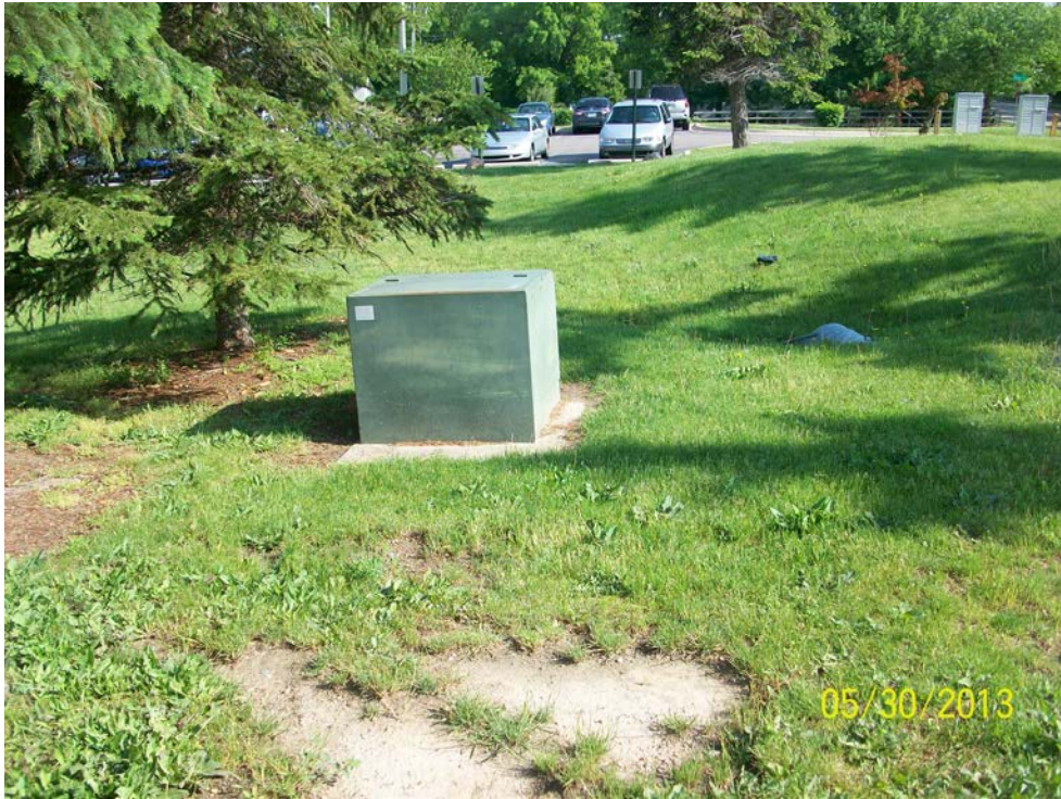
Photograph 7: Typical transformer observed on the Subject Property.
