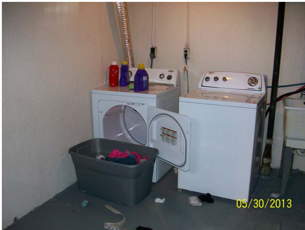
Photograph 12: Typical washing machine and dryer observed in the basement of the apartments.
