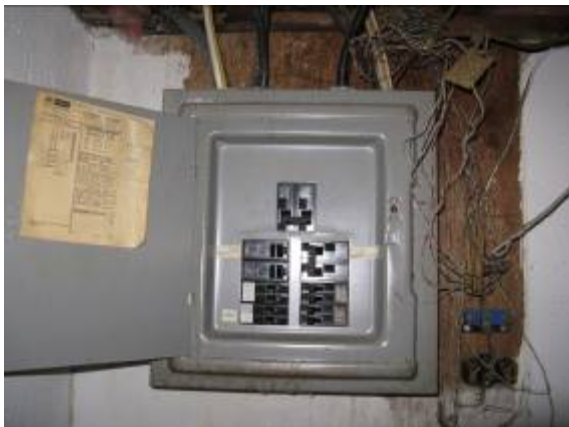
Photo #17: Circuit breaker panel
