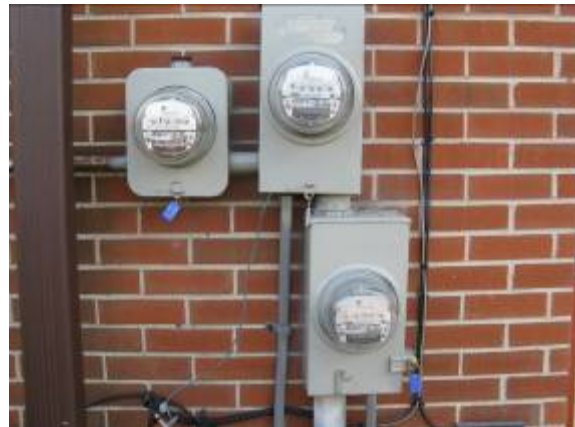
Photo #16: Electric metering
