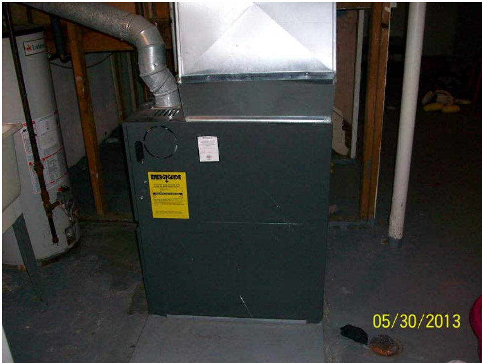
Photograph 14: Typical furnace observed in the basement of the apartments.
