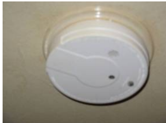
Photo #18: Smoke detector
