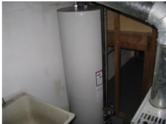
Photo #12: Water heater
