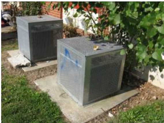
Photo #11: Community center condensing units
