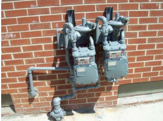
Photo #31: Gas meters and regulators
