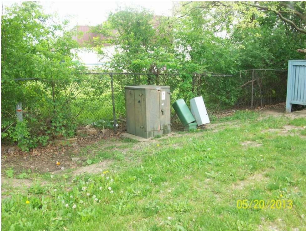
Photograph 8: Transformer observed near the northeast corner of the Subject Property.
