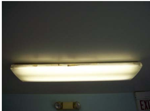
Photo #48: Fluorescent lighting in community center
