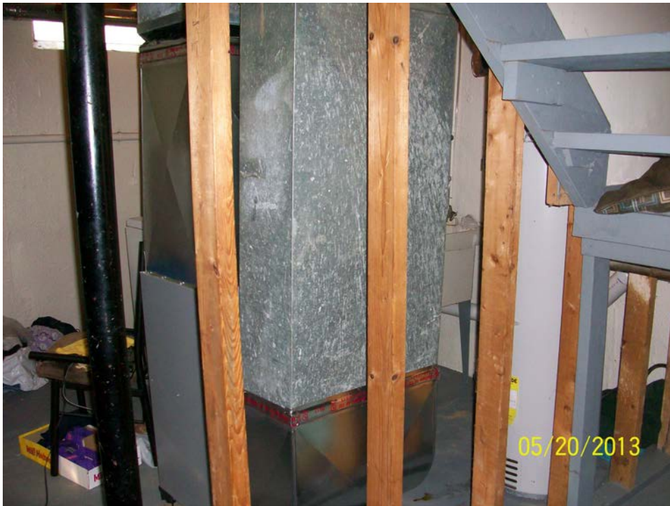
Photograph 12: Furnace and water heater in the basement of a typical apartment.
