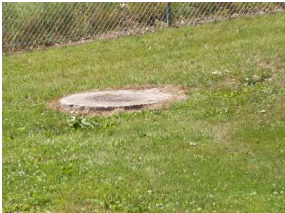
Photo #41: Storm water sump pump
