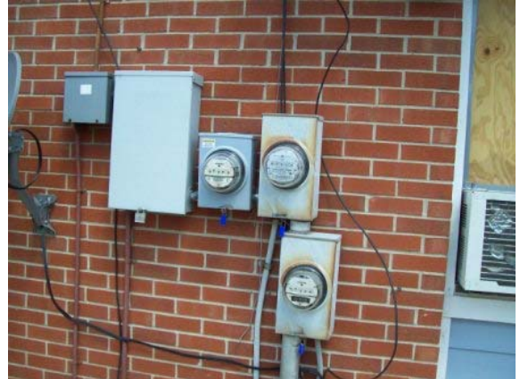
Photo #32: Electric meters
