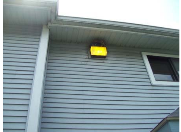
Photo #8: Soffit and gutters
