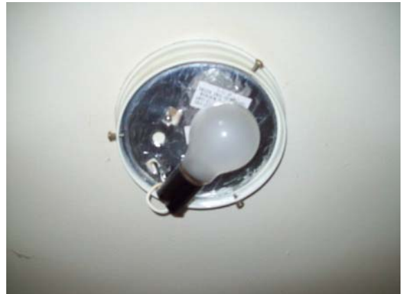
Photo #34: Incandescent light fixture
