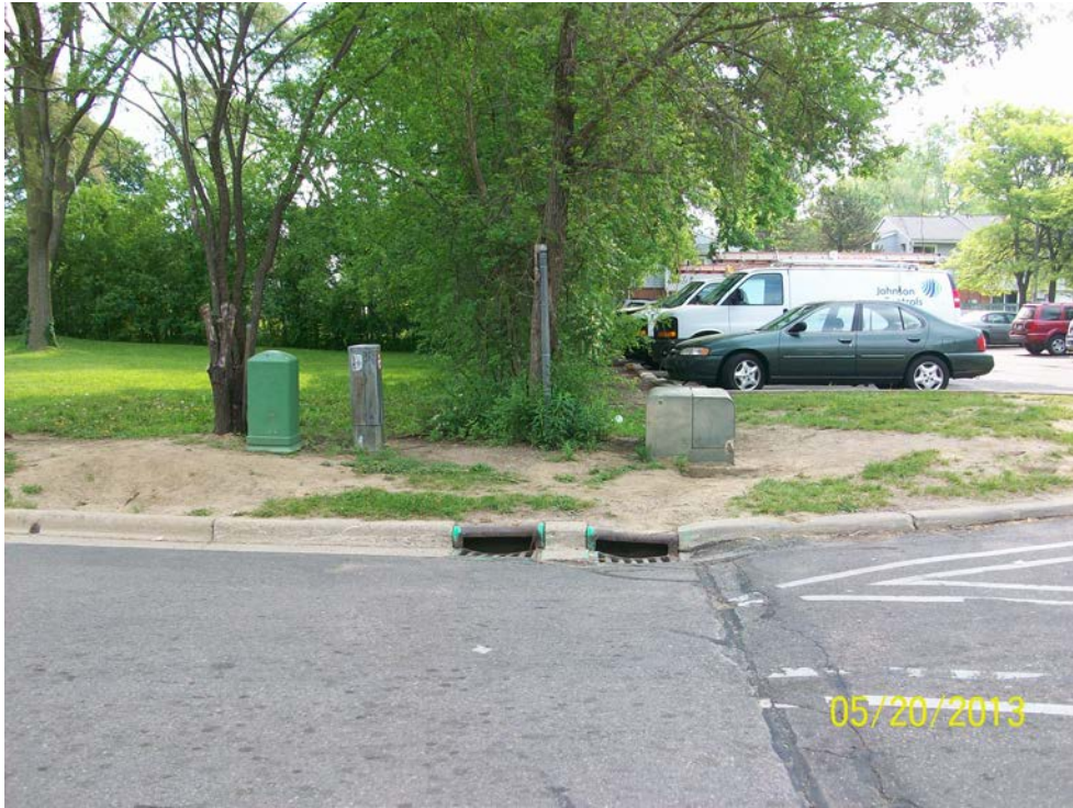
Photograph 9: Transformer observed on the north side of the Subject Property.
