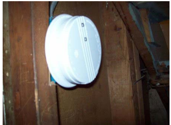
Photo #36: Smoke detector
