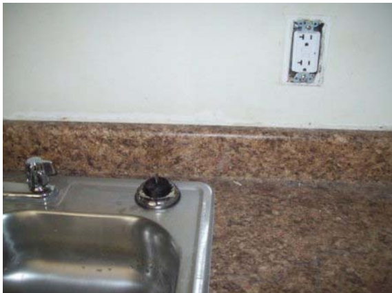
Photo #35: GFCI outlet near kitchen sink
