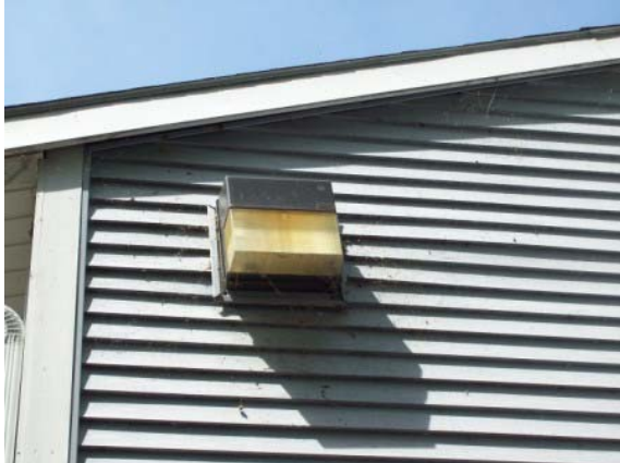
Photo #37: Building-mounted lighting
