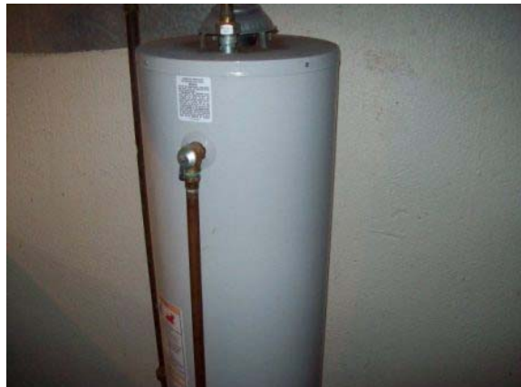
Photo #30: Domestic water heater
