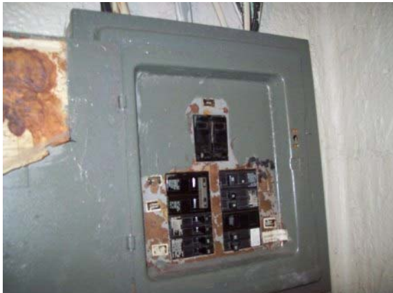
Photo #33: Breaker panel
