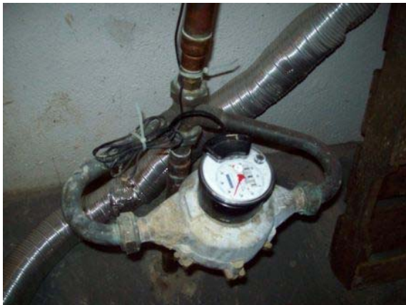
Photo #29: Building water meter
