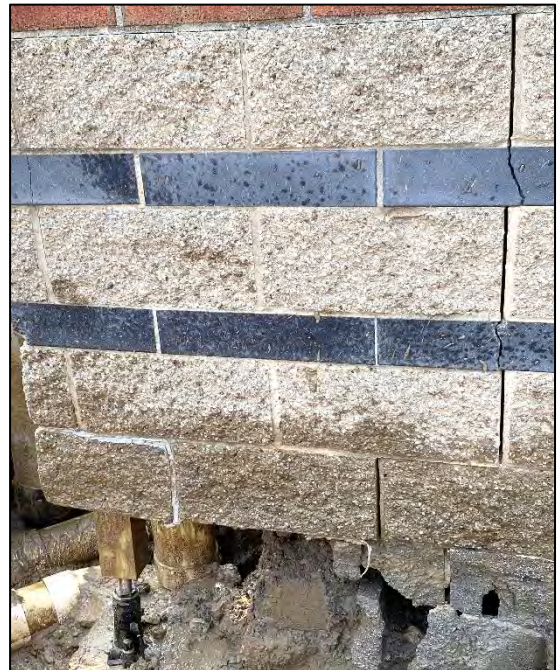
Photo 8: West Wall Cracks
