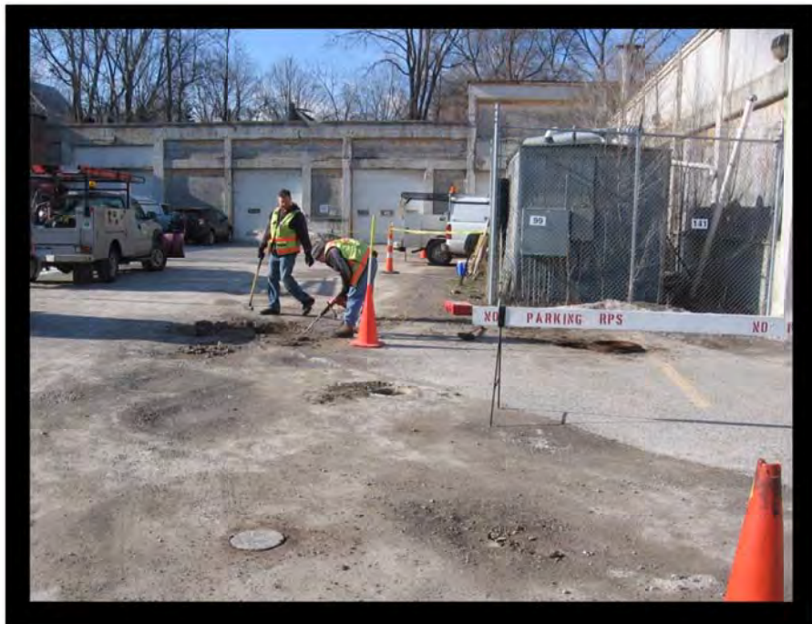
Looking west at West Garage, monitoring wells, piezometers, and manholes associated with the remediation system (right)
