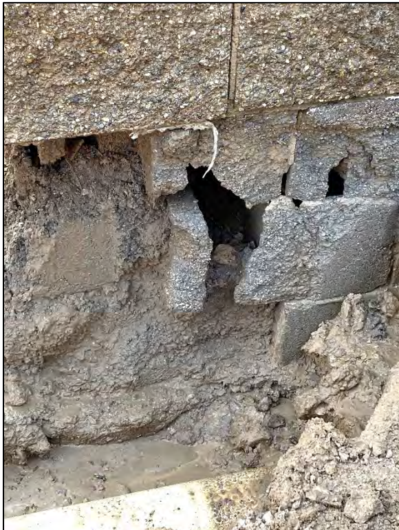
Photo 11: West Foundation Wall Disintegrating CMU
