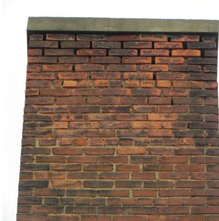
Photoset 1: Loose bricks and lack of mortar joints at top of chimney.
