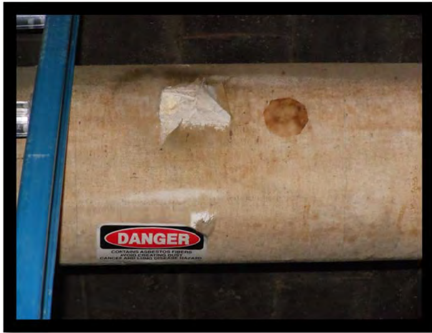
Potential asbestos covered pipes located inside the North Garage
