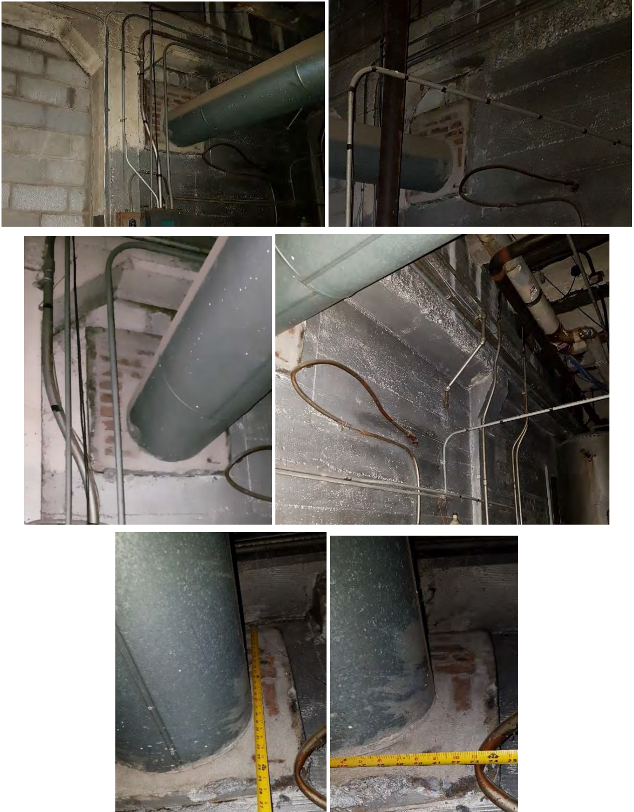
Photoset 5: Extension of the concrete beam end to the inside of the adjacent building.
