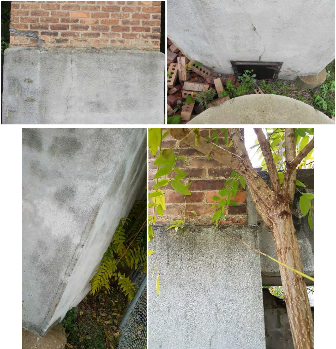
Photoset 2: Major vertical cracks along the south and east sides of the base.
