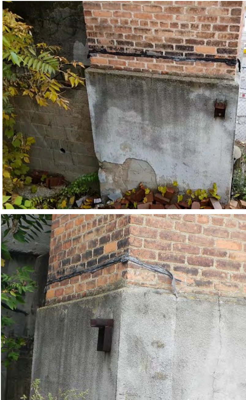
Photoset 3: Major horizontal cracks in brick above the concrete base along south and west sides.
