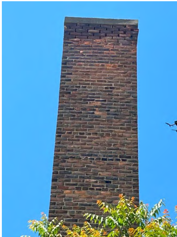
Photo 4: Top of Chimney with upper courses needed to be tuck pointed.
