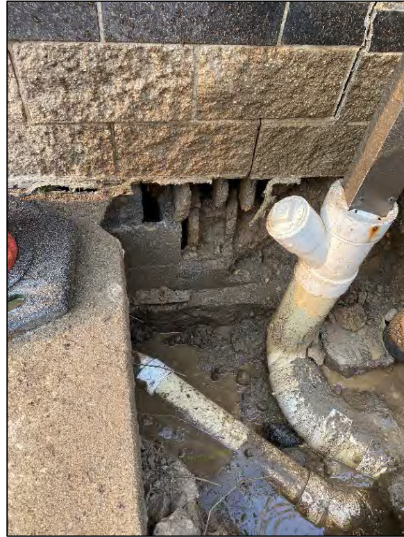
Photo 2: North Foundation Wall CMU Cores with Debris
