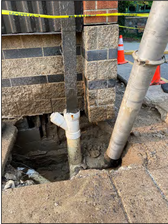
Photo 1: North Foundation Wall Missing CMU Elements
