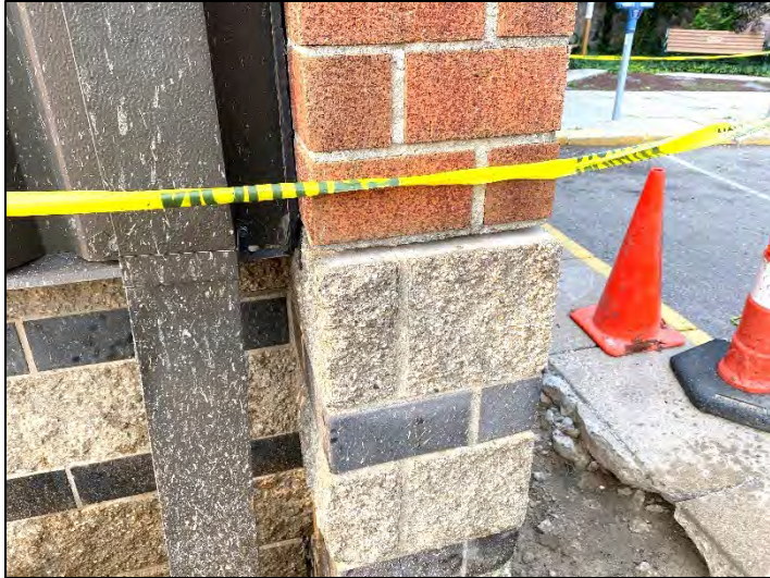
Photo 5: Northwest Wing Wall Crack (Widening During Excavations)
