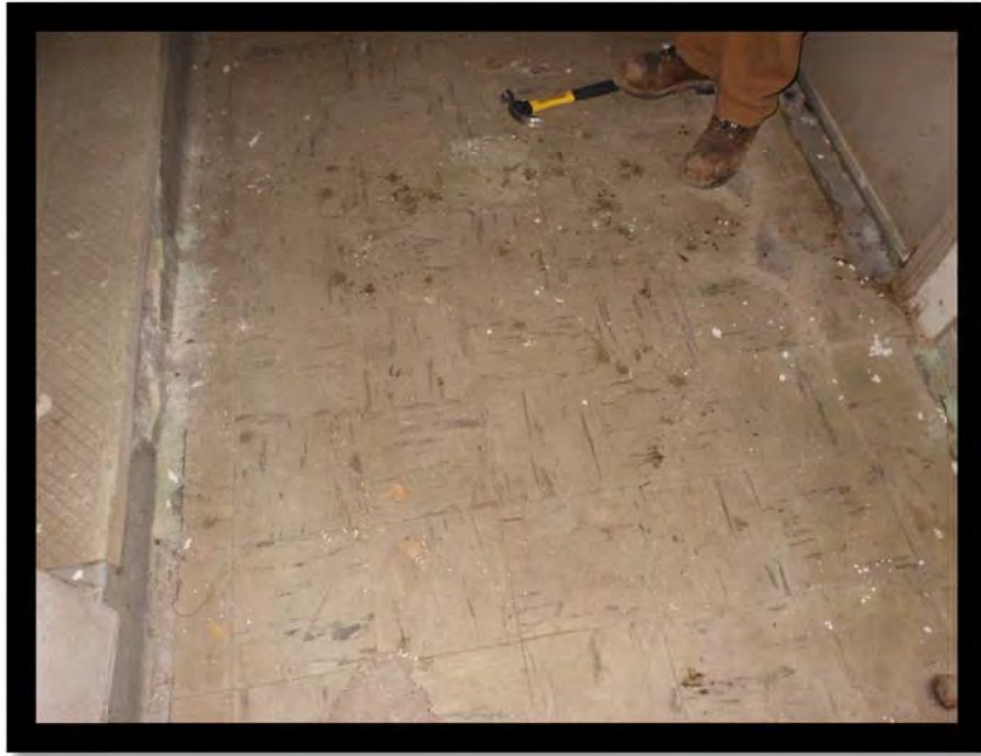
Potential asbestos containing tiles located in the offices above the North Garage
