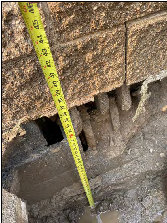
Photo 3: North Wing Wall 3 Courses of CMU Missing
