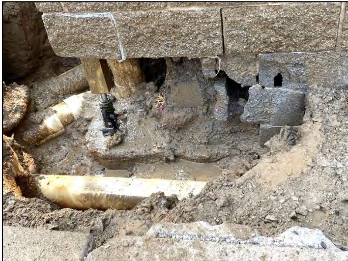
Photo 7: West Wing Foundation Wall with Missing CMU Units
