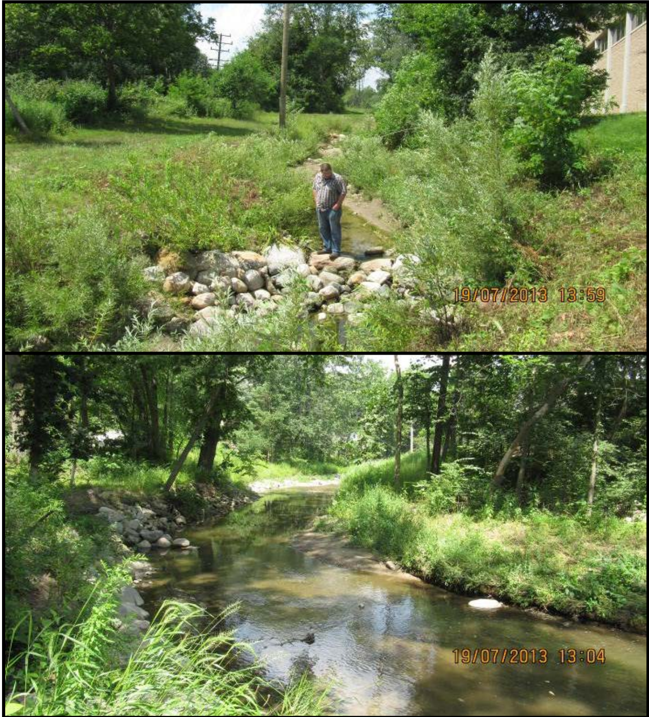
Figure 24. 2012 Mallets Creek channel restoration at County Farm Park (top) and Huron Parkway (bottom) using a combination of bank stabilization techniques and in-stream grade control structures
