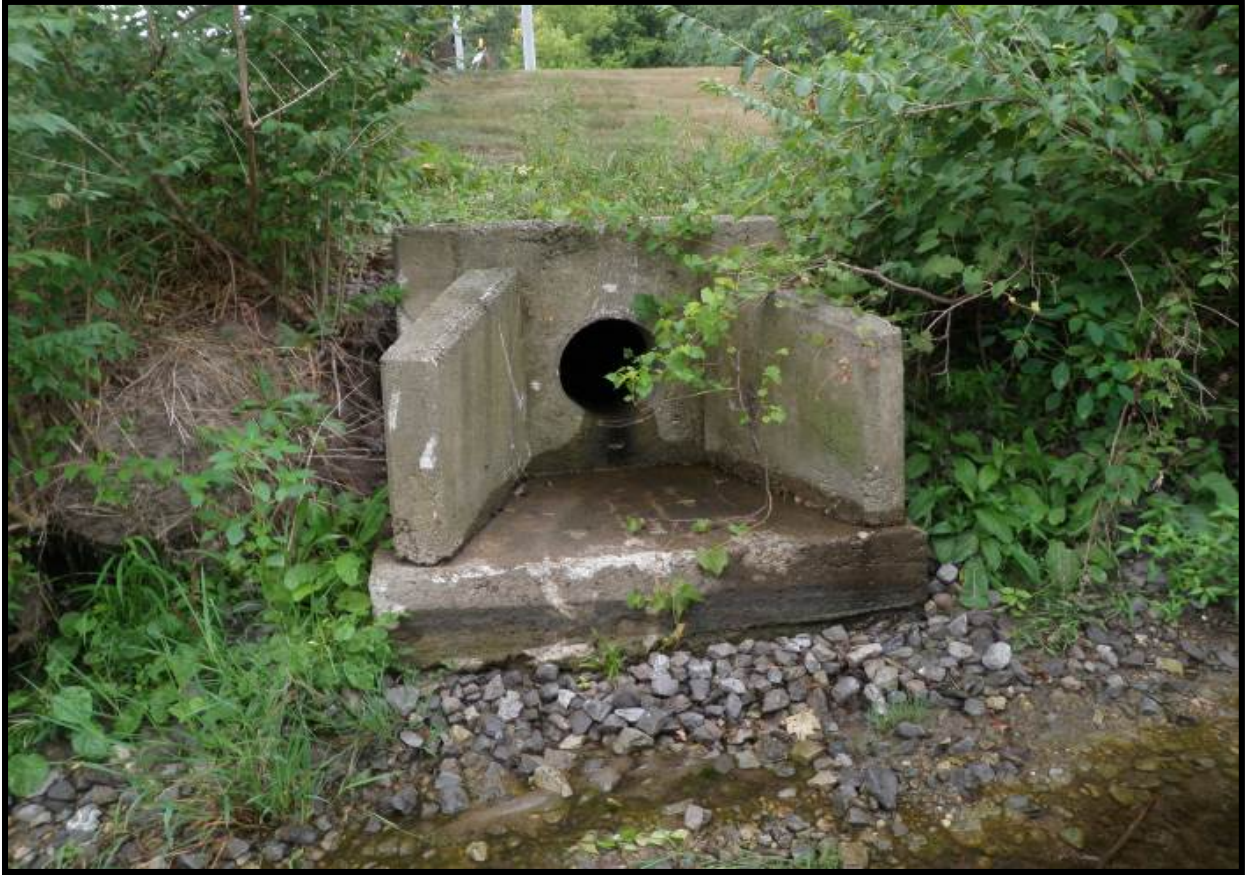
Figure 8. Storm sewer outfall in Reach 4 showing degree of bed lowering
