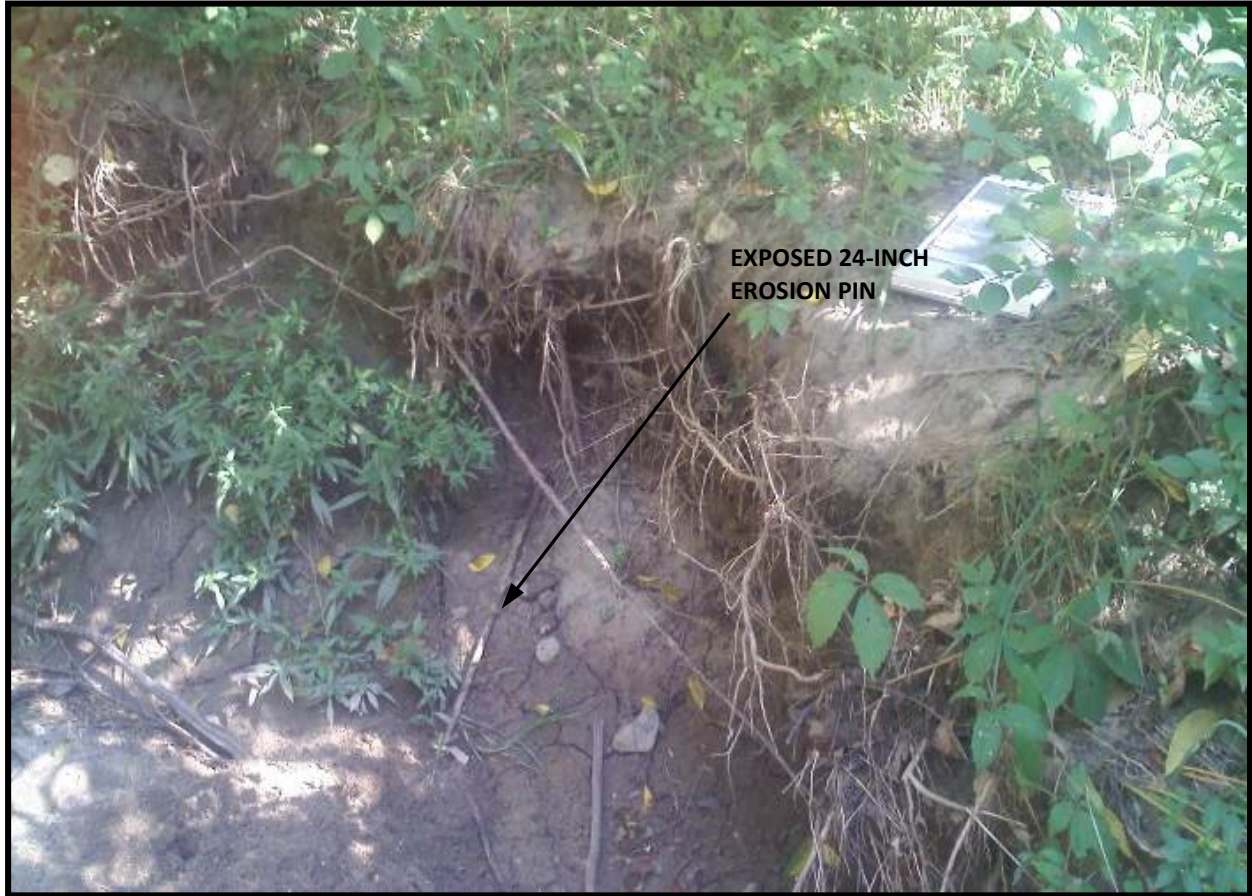
Figure 6. Completely exposed 24-inch erosion pin, Reach F
