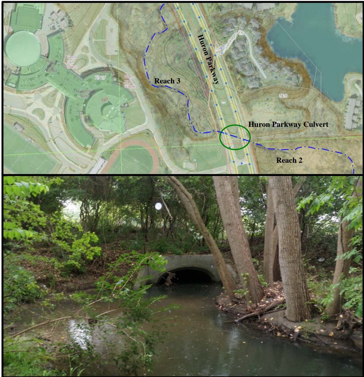
Figure 10. Location of the Huron Parkway Culvert (top) and photo (bottom) of the upstream end of the culvert showing sediment accumulation immediately upstream of the culvert and extending into the culvert.
