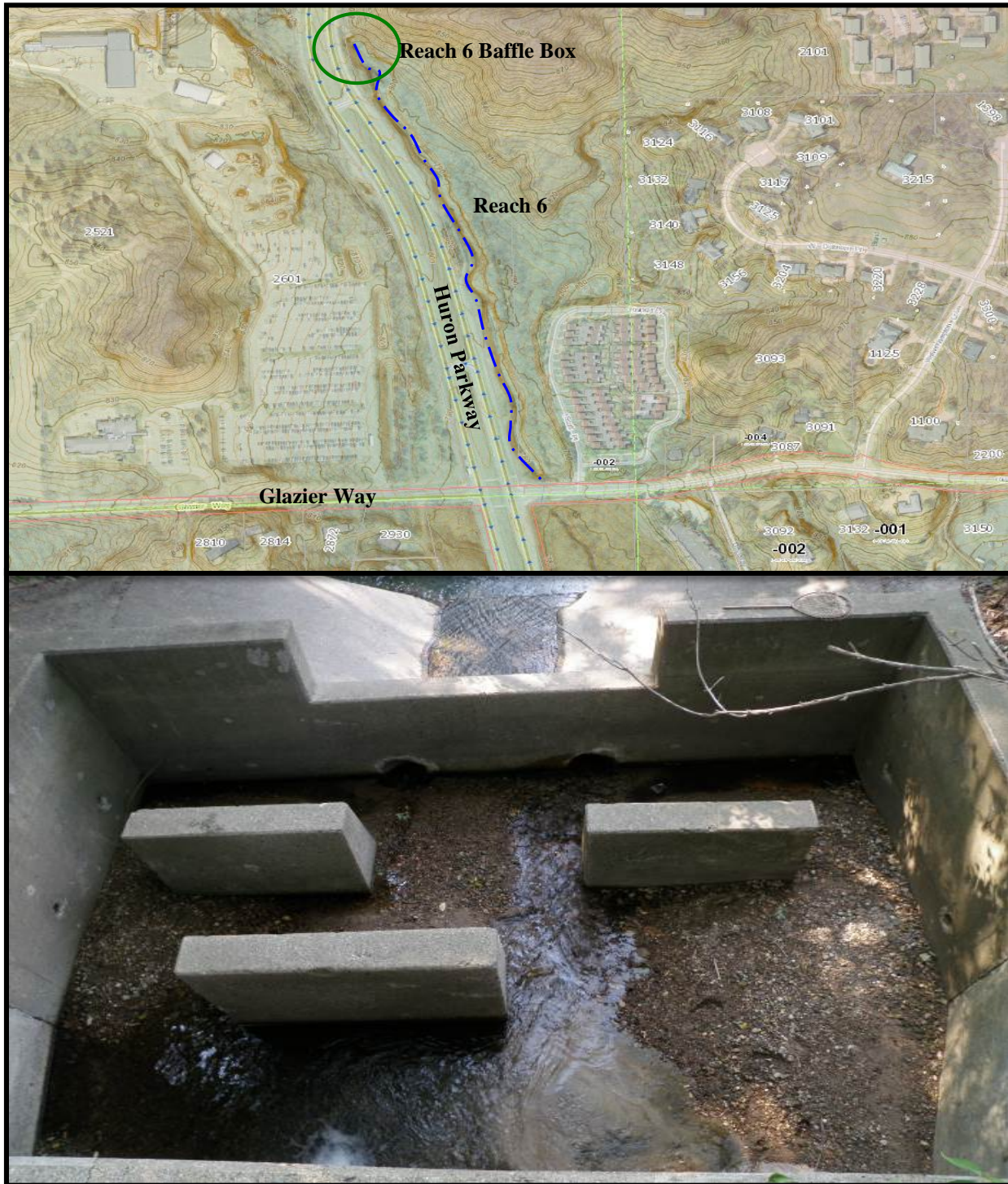
Figure 11. Location of the Reach 6 baffle box (top) and photo (bottom) of the baffle box as viewed from above
