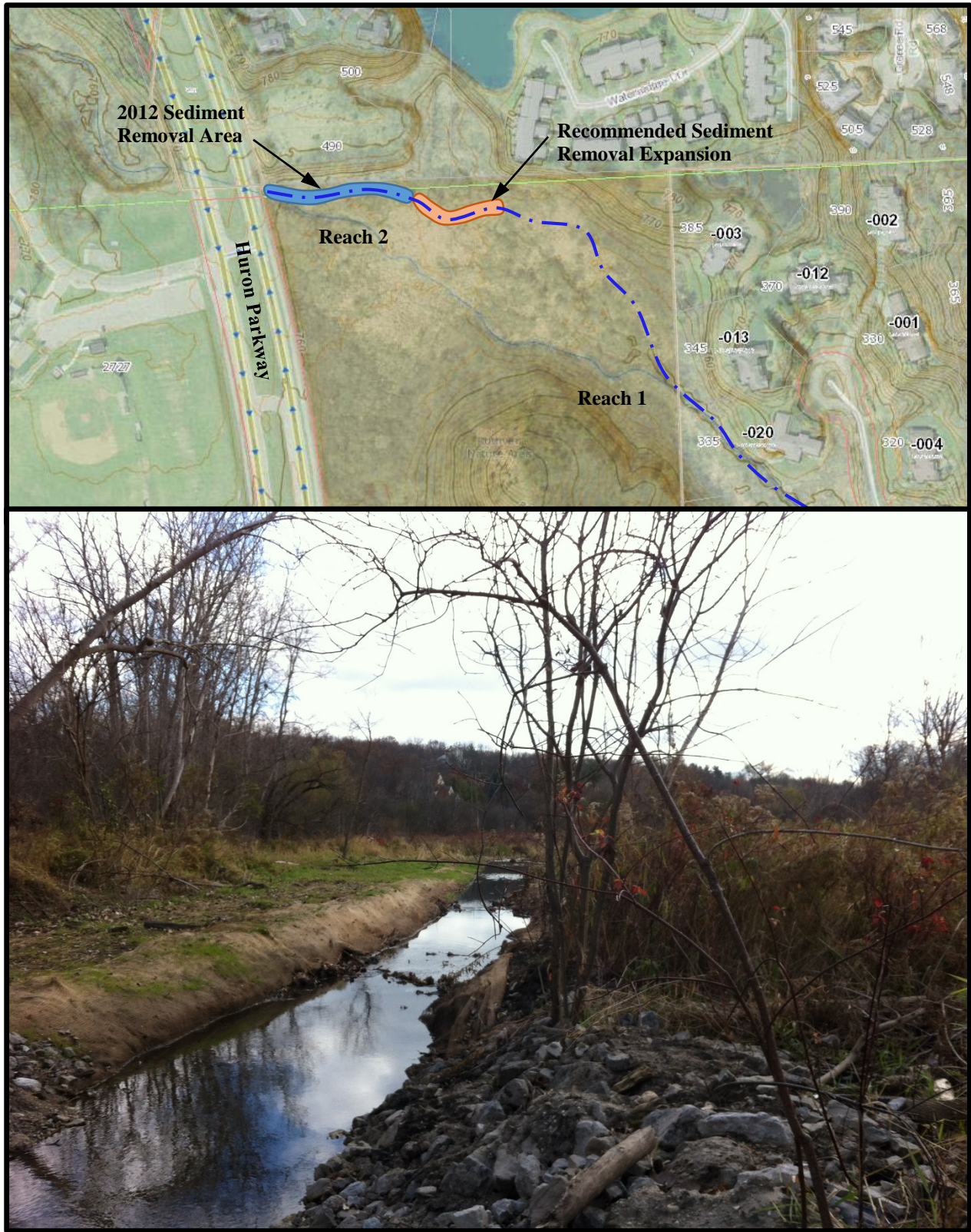
Figure 12. Location of Reach 2 expanded sediment removal (top) and photo (bottom) of sediment removal completed in 2012.
