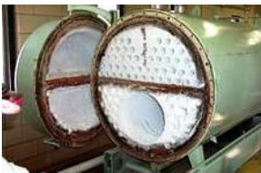
Figure 2.3 - Siloxane Deposits in Boiler
