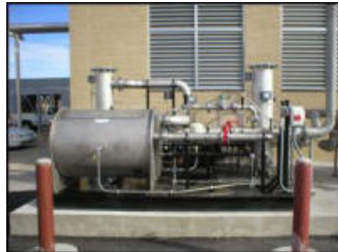
Figure 2.2 - Gas Cleaning Skid
