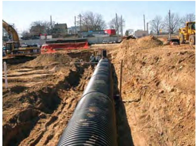
Subsurface infiltration at Mid Towne Village at the City of Grand Rapids, MI
