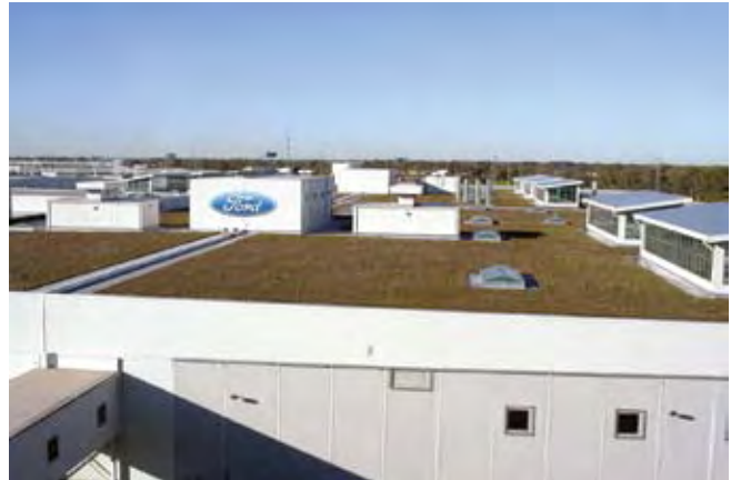
World's largest green roof covering 454,000 square feet atop Ford's truck assembly plant in Dearborn, MI.
