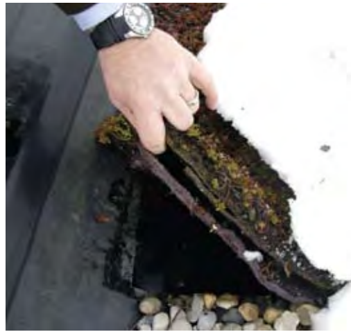
Active growth on Fraser public school maintenance green roof during winter in Fraser, MI
