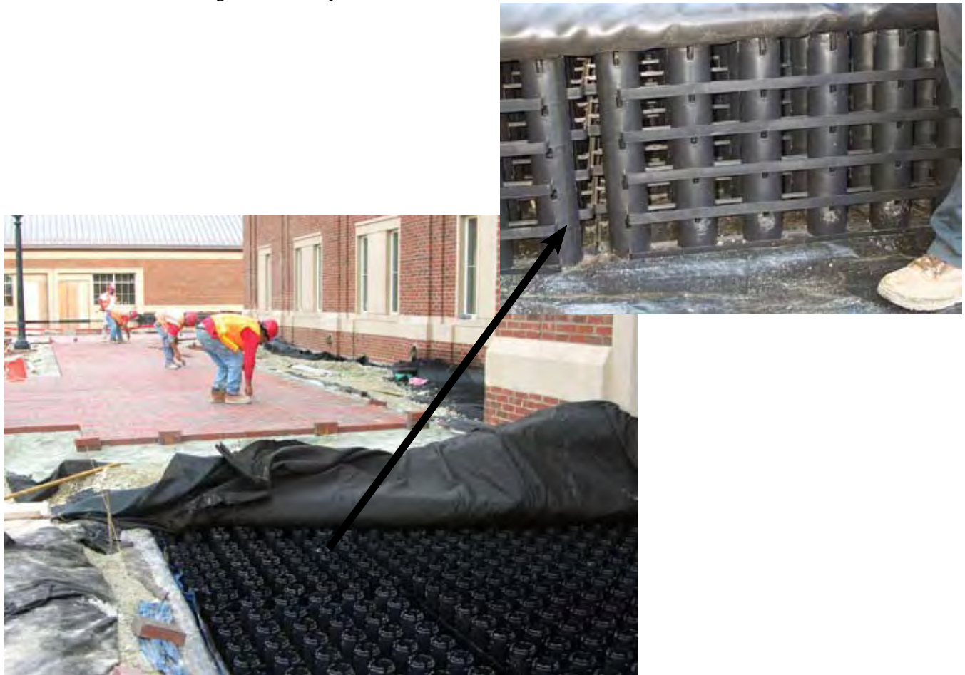
Rainstore™ cistern beneath brick pavers on a vegetated rooftop plaza at University of North Carolina – Chapel Hill
