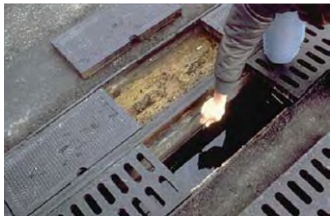
Linear perimeter filter in trench drain
