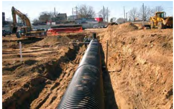
Underground system at Mid Towne Village, Grand Rapids, MI Source: Driesenga & Associates, Inc.
