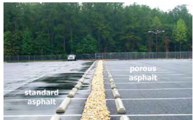
Figure 7.33 Riverstone edge serves as a backup inlet into the infiltration bed under the porous asphalt
