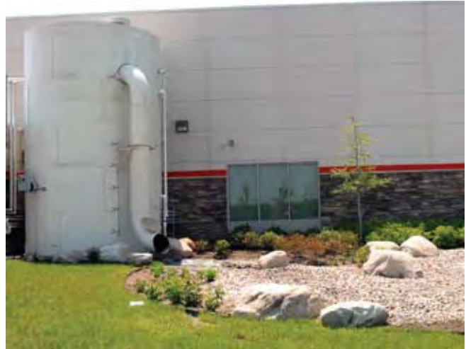
Retail center with cistern for greywater needs
