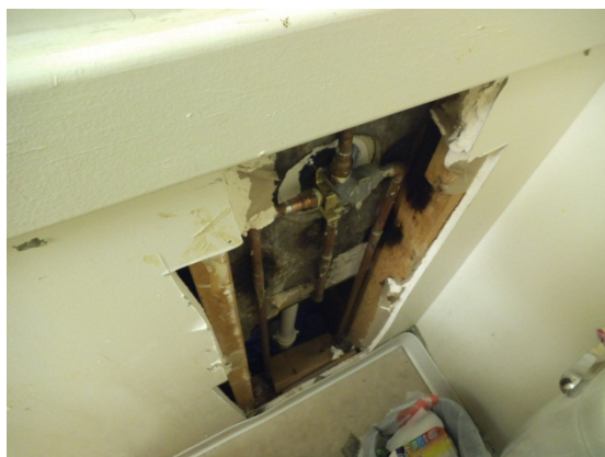
Photo 11: Cut-out wall section in bathroom (exposed to crawl space)
