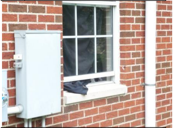
Photo #22: Missing window screen, potential pest entry point
