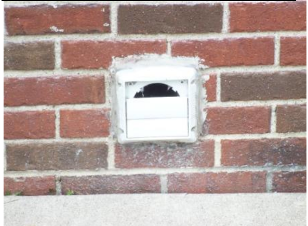
Photo #18: Missing dryer vent flap, potential entry point
