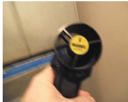
Substantial flow to outside through ducts
