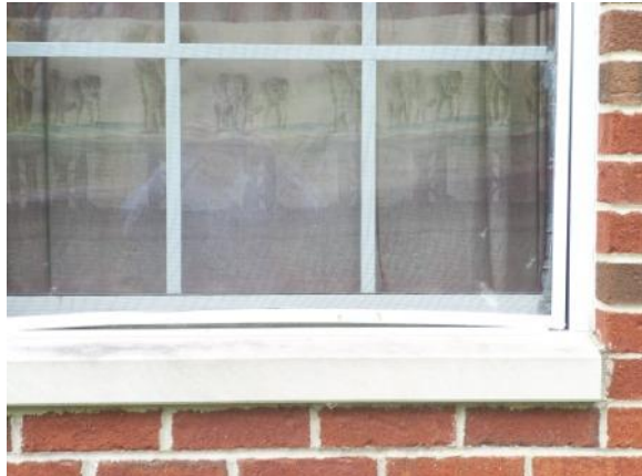
Photo #19: Bent window screens, potential entry point
