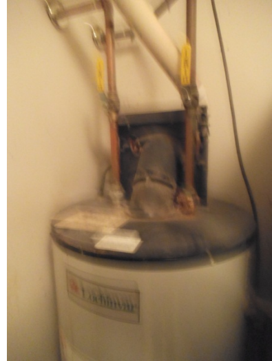
Photo 8: Typical DHW storage tank in unit
