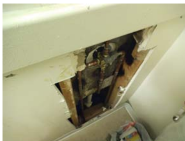
Plumbing chase at bathroom
