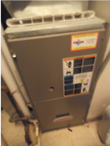
Photo 7: Typical high-efficiency furnace in unit
