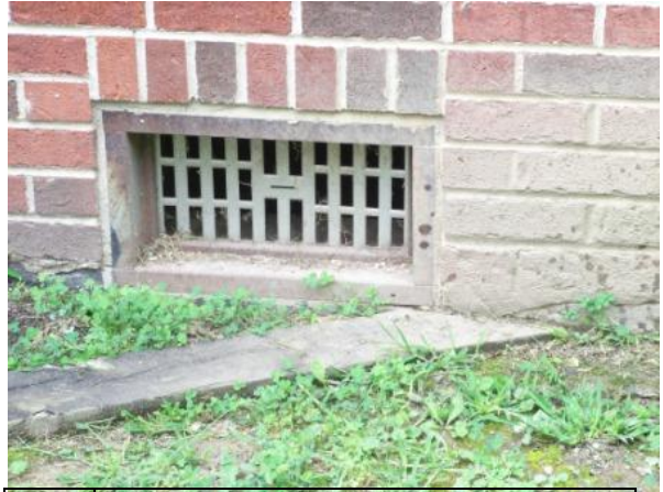
Photo #190: Crawlspace vents missing mesh, potential pest entry point
