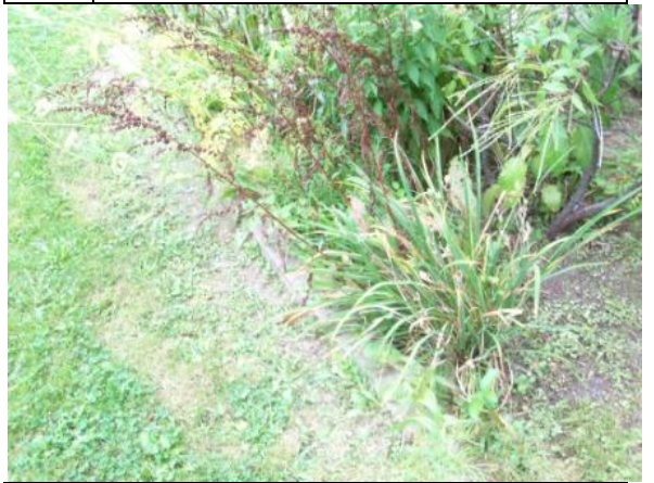
Photo #24: Railroad ties – wood/soil contact, attractive to termites.
