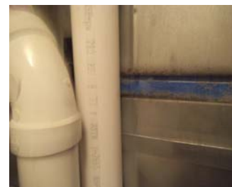
Filter removal blocked by PVC venting
