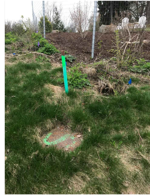
71-70034 • MH ON A SMALL HILL BETWEEN NICHOLAS DR & BACK YARD OF A HOUSE. • RIM: 909.00 • INVERT ELE: 900.00 • NOT ACCESSIBLE WITH A VEHICLE • PHOTO LOOKING SOUTH
