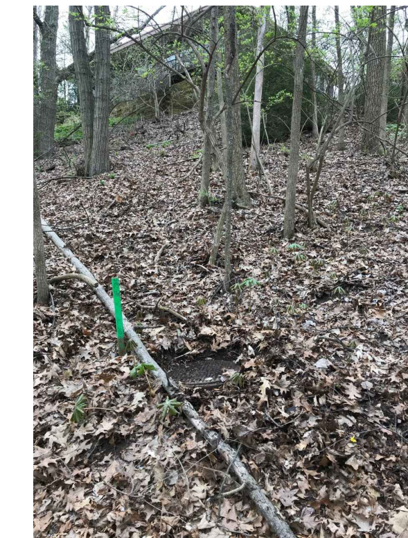
71-69943 • MH ON A STEEP SLOPE IN A FENCED BACK YARD. • RIM: 833.63 • INVERT ELE: 825.63 • NOTE 1 • PHOTO LOOKING SOUTHEAST
