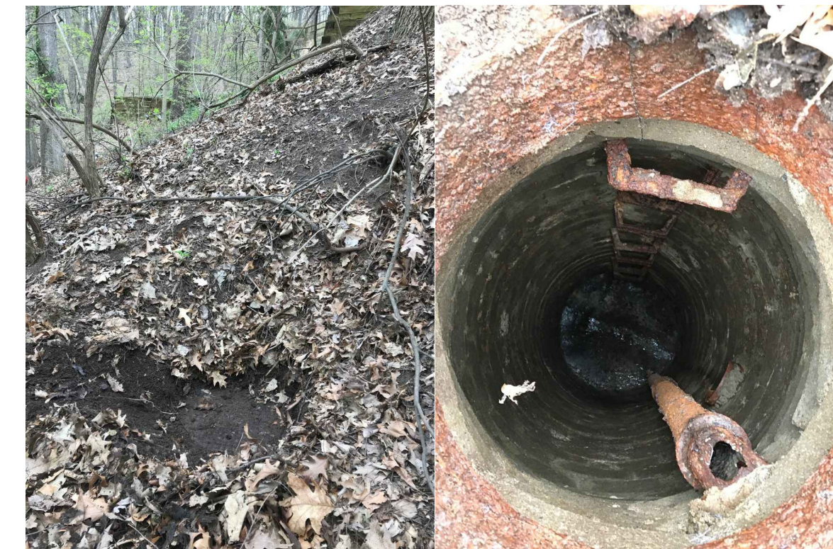
71-69944 • MH ON A STEEP SLOPE IN A FENCED BACK YARD WITH 2 DROP CONNECTIONS. • ADJUST TO GRADE • RIM: 857.09 • INVERT ELE: 842.09 • NOT ACCESSIBLE BY A VEHICLE • PHOTOS LOOKING NORTHEAST & INTO MH
