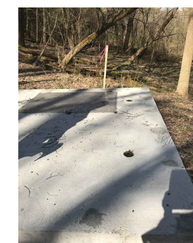
71-69895 RIM: 776.56 INVERT ELE: 767.81 PHOTO LOOKING EAST
