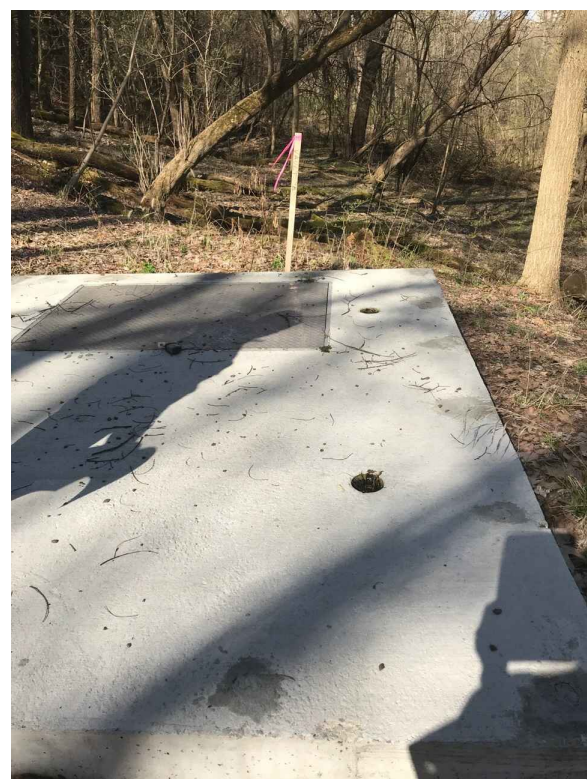
71-69895 • RIM: 776.56 • INVERT ELE: 769.39 • PHOTO LOOKING EAST
