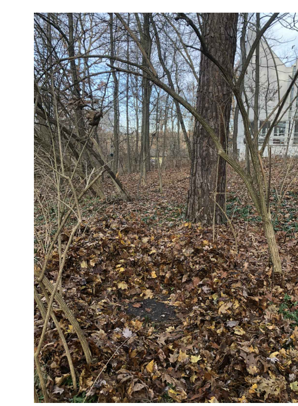
71-70071 • RIM: 773.31 • INVERT ELE: 764.95 • PHOTO LOOKING NORTHEAST
