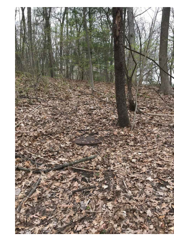
71-70073 • RIM: 775.57 • INVERT ELE: 765.57 • CASTING NEEDS REPLACEMENT • PHOTO LOOKING SOUTH
