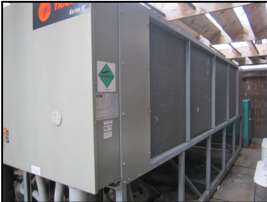
PHOTOGRAPH NO. 8: SUBJECT BUILDING: TYPICAL VIEW OF CENTRAL CHILLER FOR COOLING
