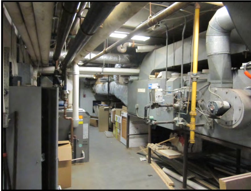
PHOTOGRAPH NO. 7: SUBJECT BUILDING: TYPICAL VIEW OF GAS-FIRED MUA UNIT
