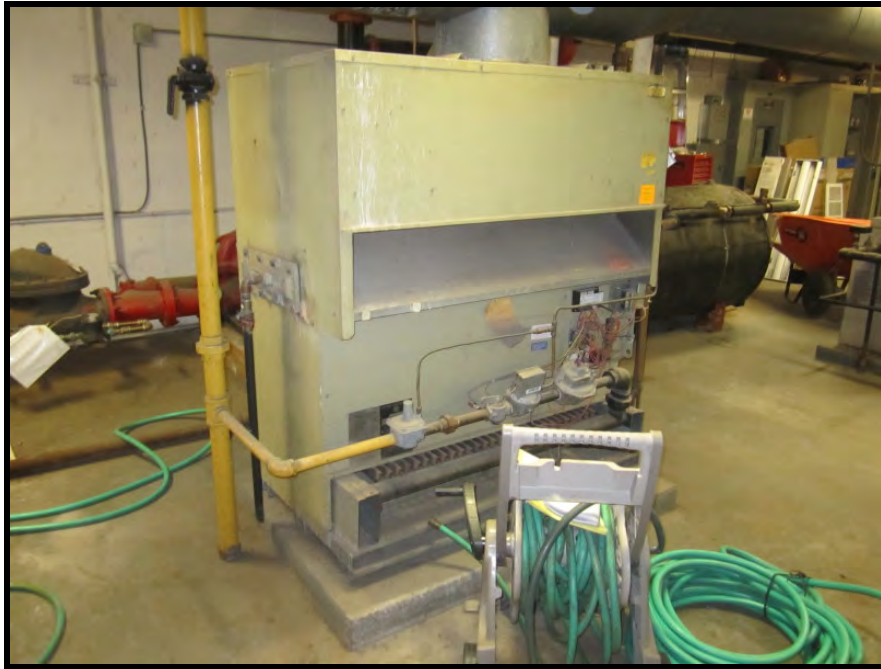
PHOTOGRAPH NO. 5: SUBJECT BUILDING: VIEW OF HOT WATER BOILER
