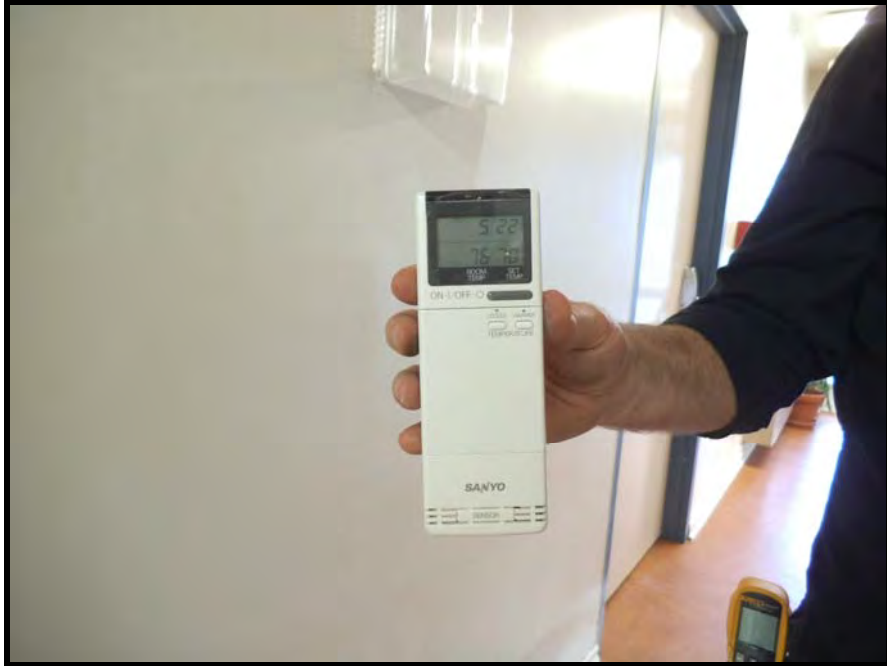
PHOTOGRAPH NO. 19: SUBJECT BUILDING: VIEW OF THERMOSTAT FOR FAN COIL TERMINALS
