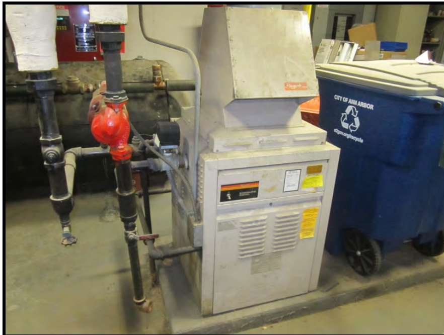
PHOTOGRAPH NO. 4: SUBJECT BUILDING: VIEW OF BACKUP HOT WATER BOILER FOR SPACE HEATING
