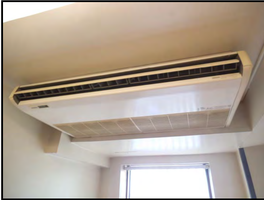
PHOTOGRAPH NO. 11: SUBJECT BUILDING: TYPICAL VIEW OF INDOOR FAN COIL UNITS
