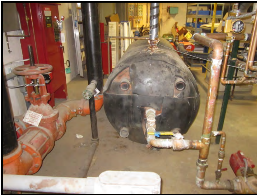
PHOTOGRAPH NO. 6: SUBJECT BUILDING: VIEW OF HOT WATER STORAGE TANK
