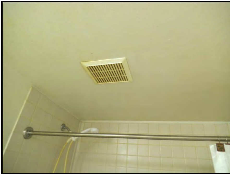
PHOTOGRAPH NO. 16: SUBJECT BUILDING: TYPICAL VIEW OF TENANT UNIT BATHROOM EXHAUST FAN
