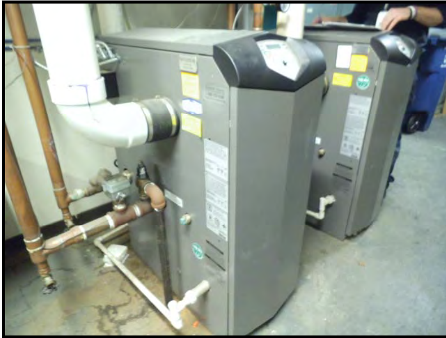
PHOTOGRAPH NO. 3: SUBJECT BUILDING: VIEW OF HIGH EFFICIENCY HEATING BOILERS
