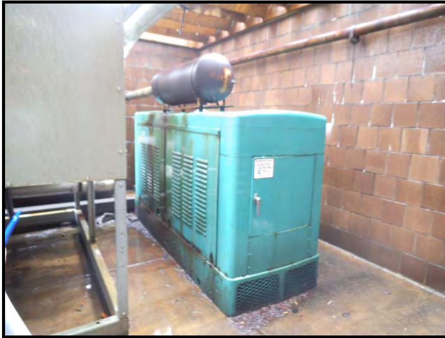
PHOTOGRAPH NO. 9: SUBJECT BUILDING: TYPICAL VIEW OF OLD DIESEL GENERATOR
