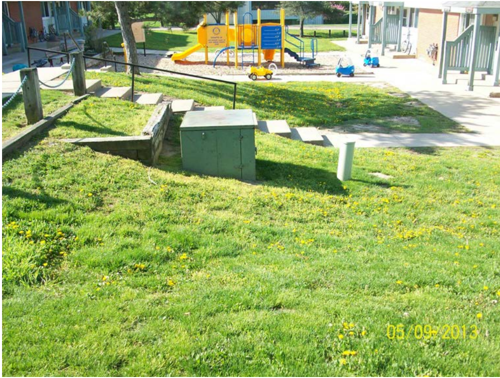
Photograph 13: Switch gear observed on the Subject Property.
