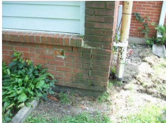
Photo #16: Brick veneer damage
