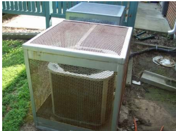
Photo #42: Condensing units for Community Center
