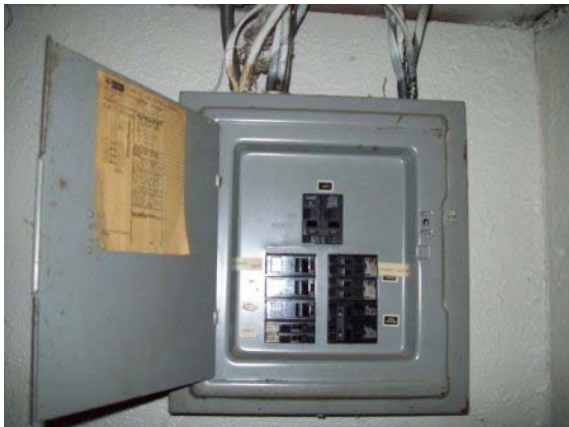
Photo #35: Breaker panel
