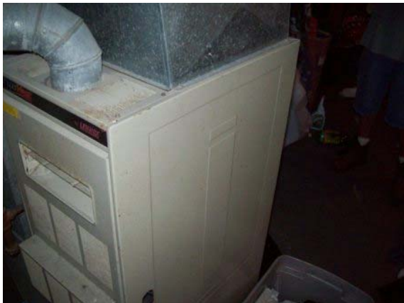
Photo #41: Furnace in Community Center
