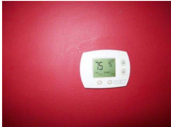
Photo #40: Thermostat in Community Center
