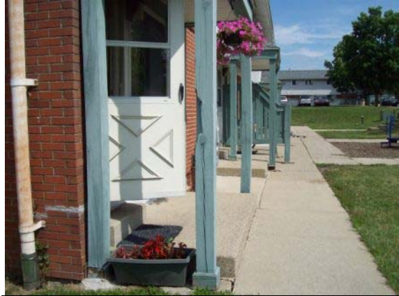
Photo #14: Damaged wood posts at entry structure
