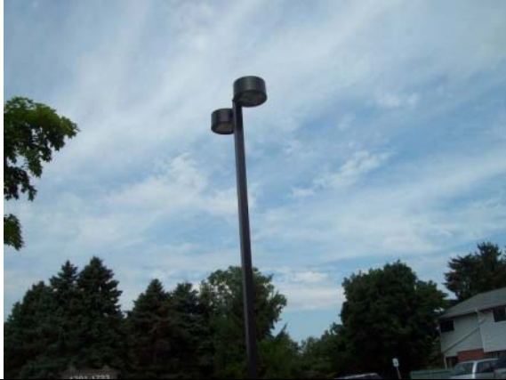
Photo #43: Pole-mounted lighting
