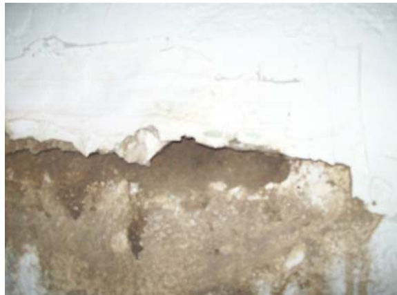
Photo #18: Basement wall damage in Unit 1723
