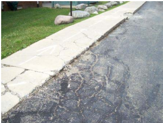
Photo #11: Asphalt and sidewalk damage
