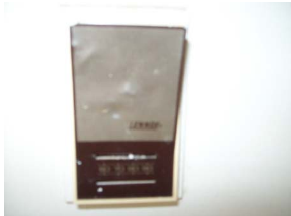
Photo #30: Older thermostat
