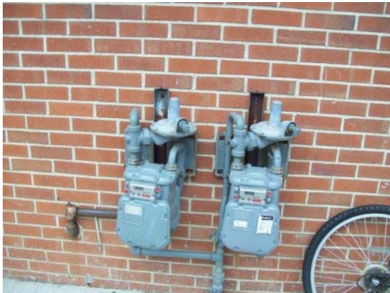
Photo #33: Gas meters and regulators
