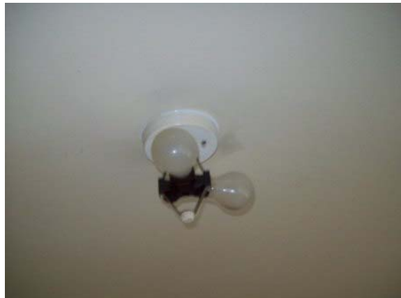
Photo #36: Incandescent lighting
