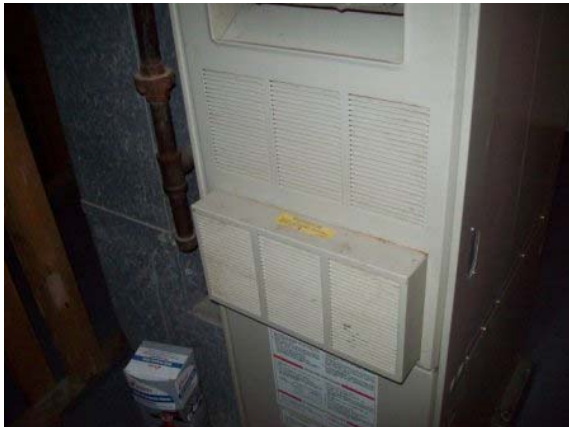
Photo #27: Typical furnace
