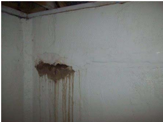
Photo #17: Basement wall damage in Unit 1723
