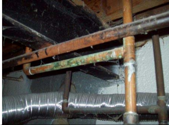
Photo #32: Domestic water piping and gas piping
