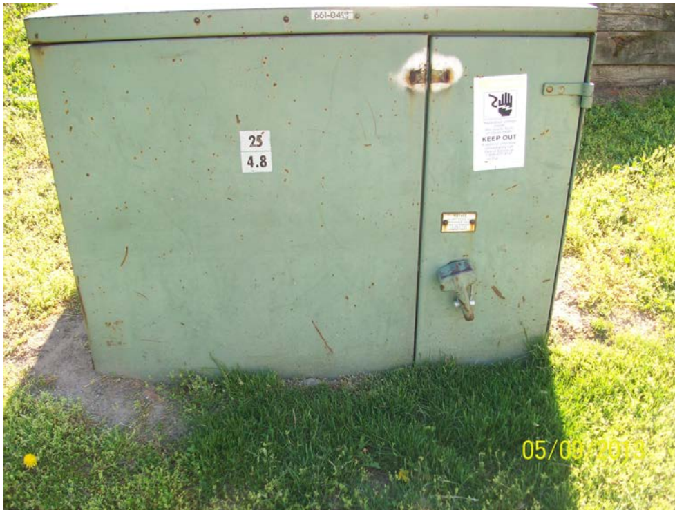
Photograph 14: Switch gear observed on the Subject Property.
