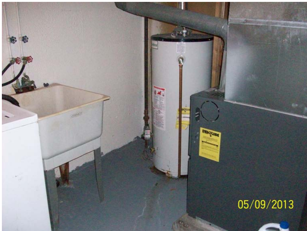
Photograph 10: Typical water heater and furnace in the basement of the apartment units.
