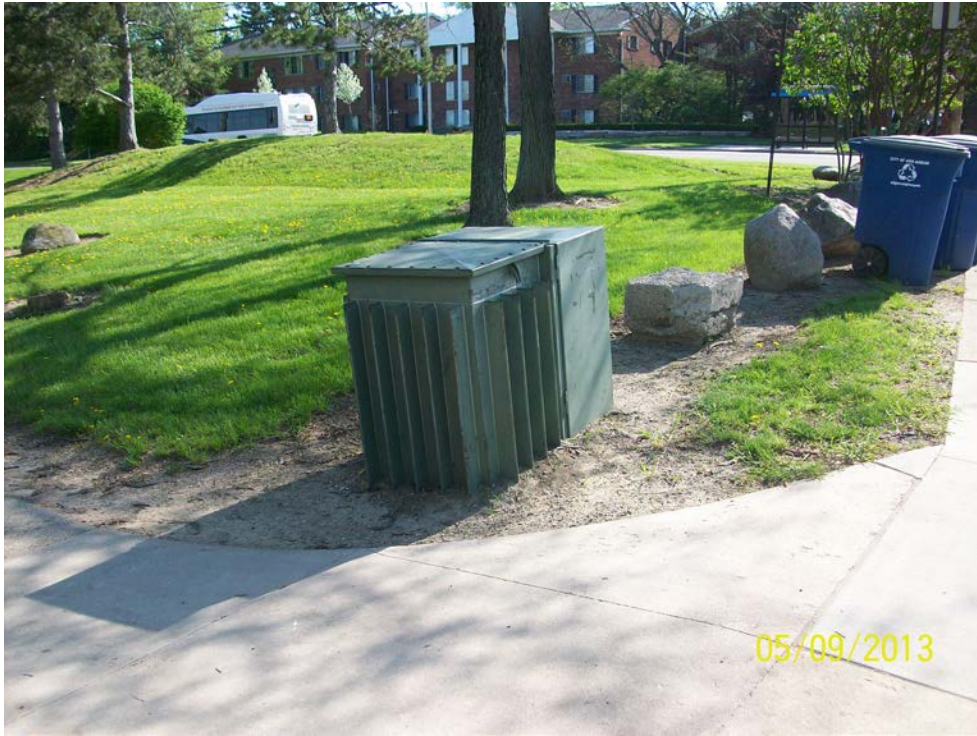
Photograph 15: Typical transformer observed on the Subject Property.
