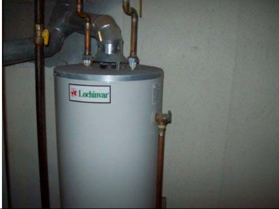
Photo #31: Domestic water heater
