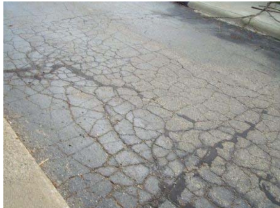
Photo #10: Asphalt detail – alligator cracking
