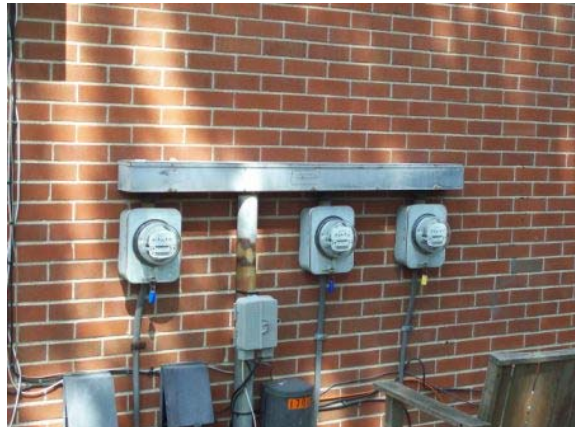
Photo #34: Electric meters
