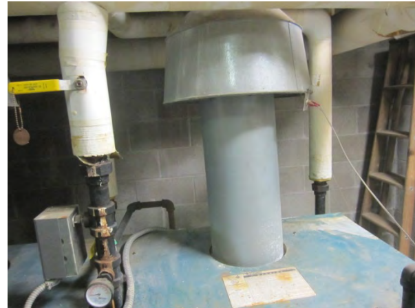
Photo 16: Insulated Hot Water Piping
