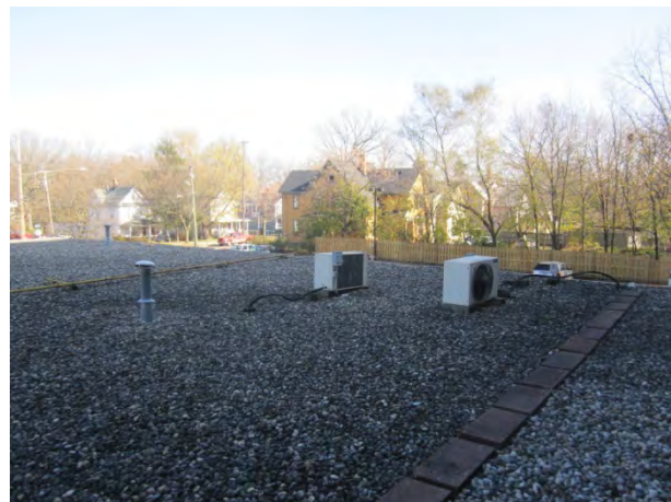
Photo 24: Split system condensing unit for lobby
