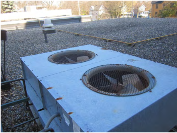
Photo 27: Split system condensing unit for community room
