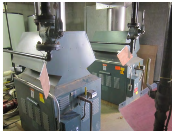
Photo 18: Domestic Water Boilers
