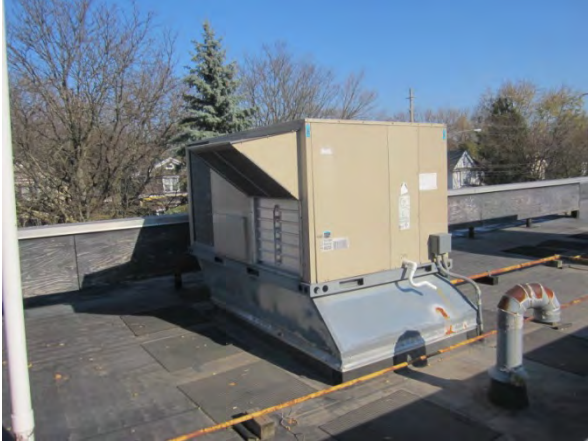
Photo 25: Packaged rooftop unit for west end of office area
