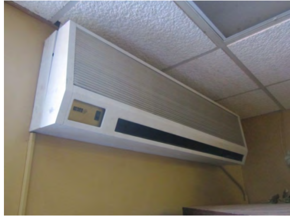
Photo 20: Interior fan coil unit
