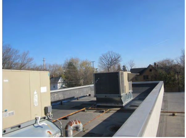
Photo 26: Packaged rooftop unit for east end of office area
