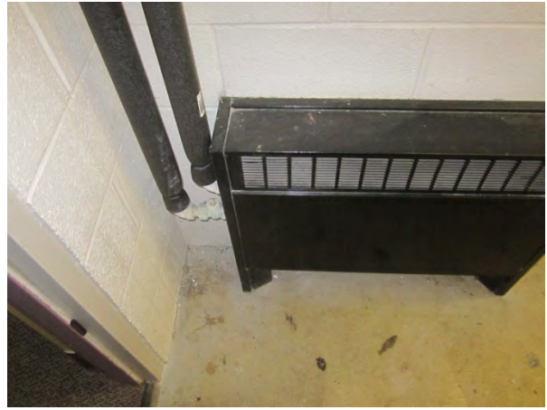
Photo 28: Hot water unit heater in stairwell
