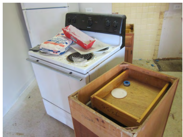
Photo 12: Resident Gas Range Oven
