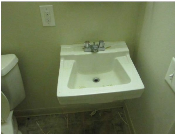
Photo 11: Typical Bathroom Sink
