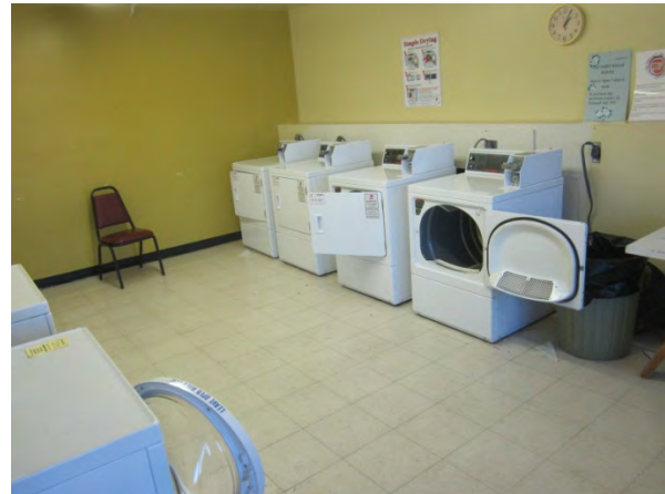
Photo 22: Common Area Dryers
