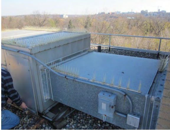
Photo 19: Make-up air unit (1 of 2)
