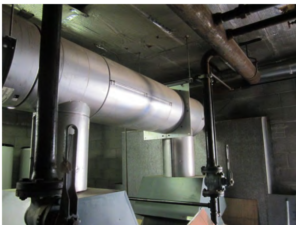
Photo 17: Natural draft exhaust venting
