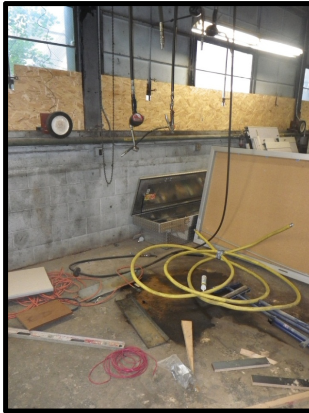
Staining on concrete in maintenance garage
