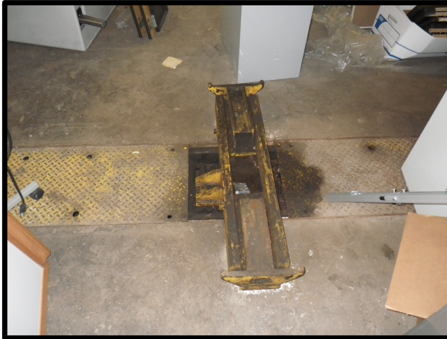
Hoist system in maintenance garage
