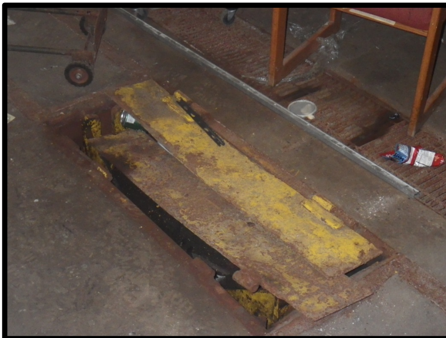
Hoist system and associated trenches in maintenance garage
