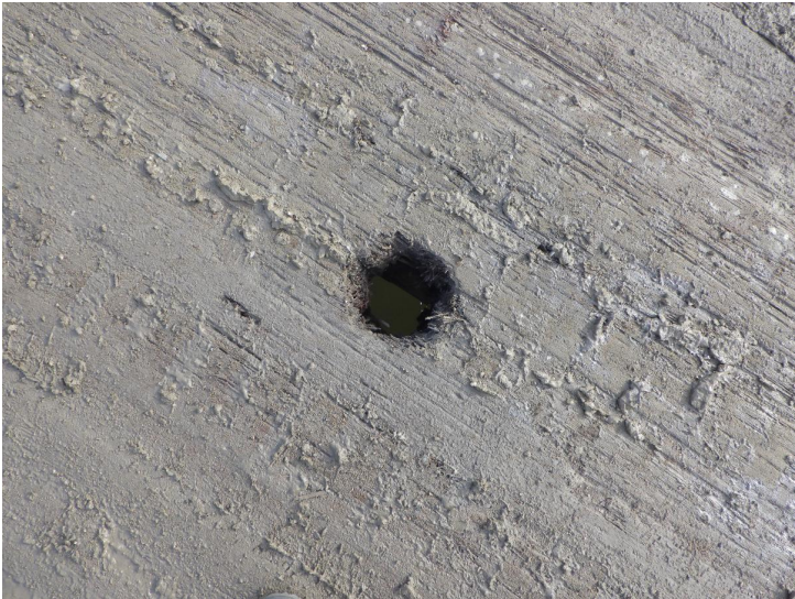
Document Name: R0011783.JPG Category: Deck Span Number: 2 Comments: Boring hole near midspan of bridge
