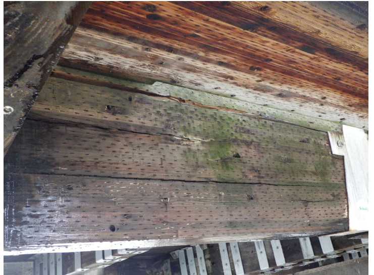
Document Name: R0011805.JPG Category: Superstructure Span Number: 2 Comments: Multiple splits in west beam near south splice
