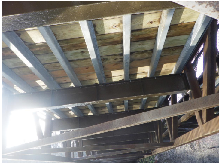
Document Name: R0012534.JPG Category: Superstructure Span Number: 1 Comments: Typical galvanized stringers and bottom of deck
