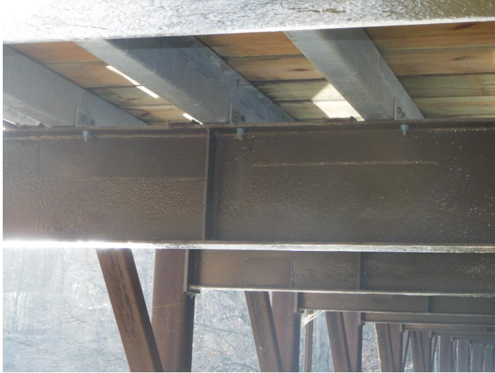
Document Name: R0012536.JPG Category: Superstructure Span Number: 1 Comments: Typical floorbeam web repair and paint condition
