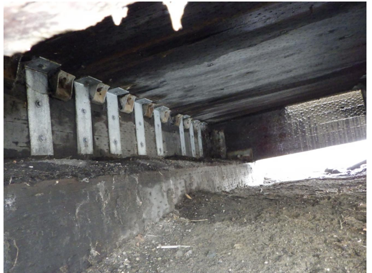
Document Name: R0011799.JPG Category: Substructure Span Number: 1 Comments: Typical timber abutments located behind previous stone abutments
