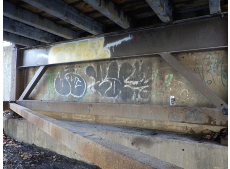
Document Name: R0011742.JPG Category: Substructure Span Number: 1 Comments: Typical abutment, south shown
