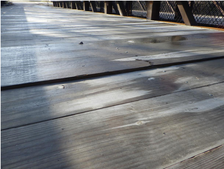
Document Name: R0011727.JPG Category: Deck Span Number: 1 Comments: Deck member with broken connection near midspan
