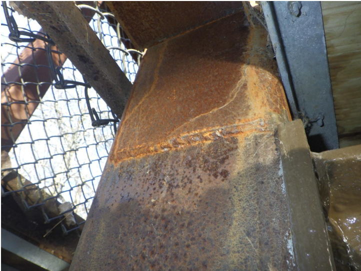
Document Name: R0012532.JPG Category: Superstructure Span Number: 1 Comments: Typical vertical truss member repair, located above floorbeam connections
