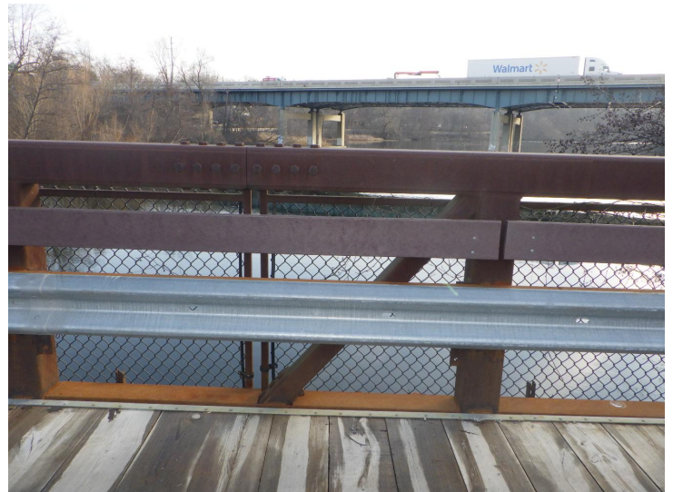
Document Name: R0012525.JPG Category: Railing Span Number: 1 Comments: Guardrail and fencing on bridge
