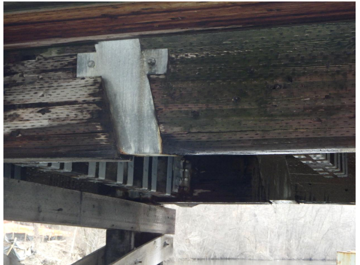
Document Name: R0011802.JPG Category: Superstructure Span Number: Comments: Hanger plate splice not supporting both sides of beam, typical all four locations
