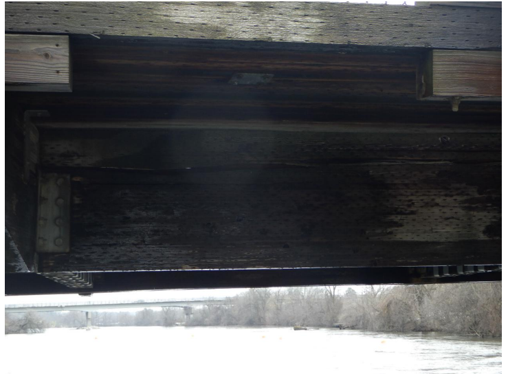
Document Name: R0011792.JPG Category: Superstructure Span Number: 2 Comments: Large split in west beam
