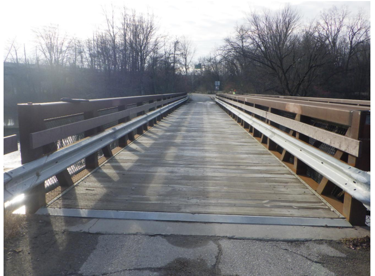
Document Name: R0012526.JPG Category: Deck Span Number: 1 Comments: Bridge deck looking south
