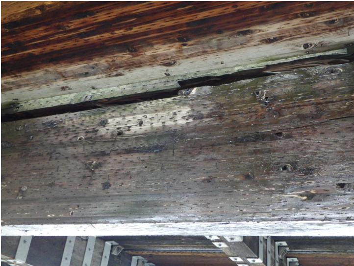
Document Name: R0011803.JPG Category: Superstructure Span Number: 2 Comments: Large split in west beam
