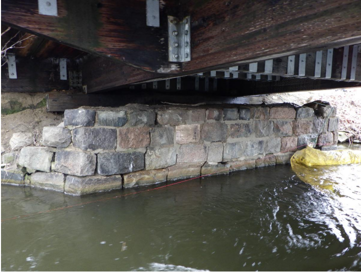
Document Name: R0011808.JPG Category: Substructure Span Number: 1 Comments: South abutment missing grout between stones. Timber abutments behind previous bridge abutment
