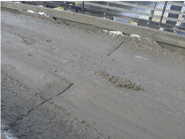
Document Name: R0011776.JPG Category: Deck Span Number: Comments: Worn wheel lines in decking, worse at edges of decking members
