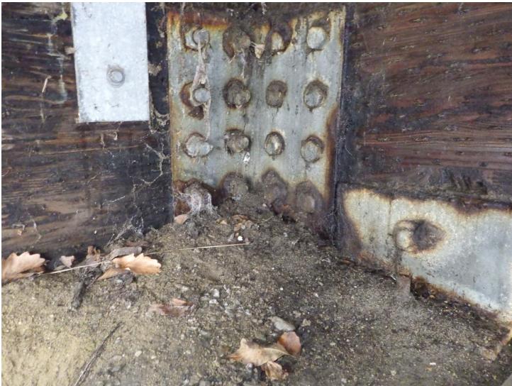
Document Name: R0011795.JPG Category: Bearings Span Number: Comments: Typical abutment bearings with debris/sediment
