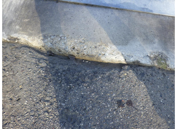
Document Name: R0011732.JPG Category: Approach Span Number: 1 Comments: HMA spall at south reference line
