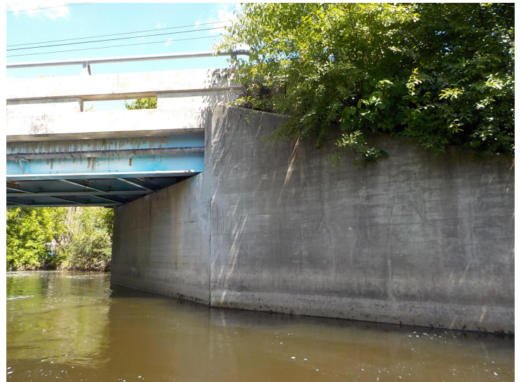
Document Name: DSCN3006.JPG Category: Substructure Span Number: Comments: Concrete returnwall at the SE quadrant
