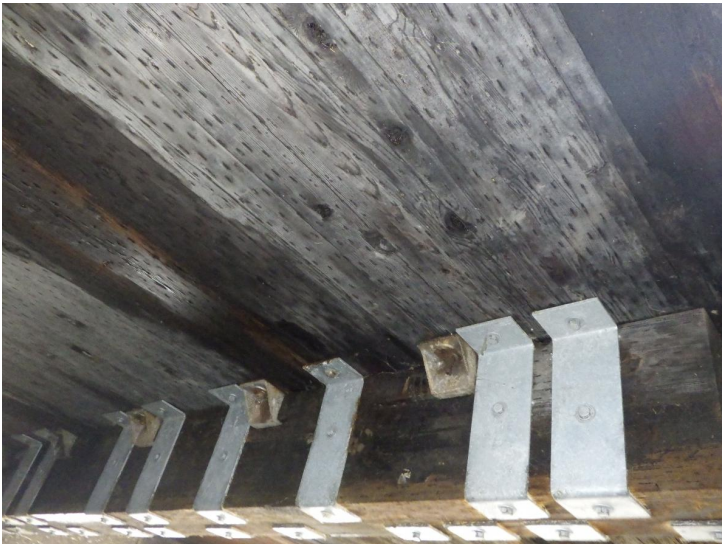
Document Name: R0011800.JPG Category: Superstructure Span Number: Comments: Typical bottom of decking and floorbeam
