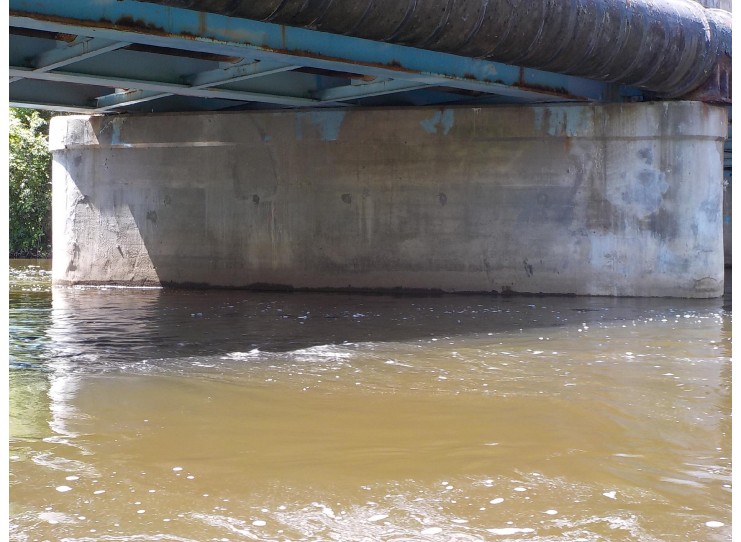
Document Name: DSCN3004.JPG Category: Substructure Span Number: Comments: East elevation of Pier 1w
