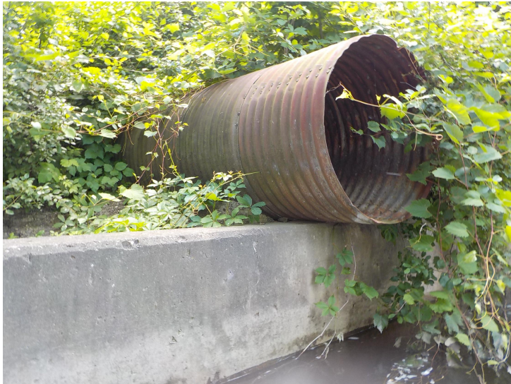
Document Name: DSCN3013.JPG Category: Culvert Span Number: Comments: Outlet culvert NE quadrant
