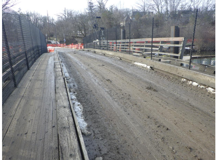
Document Name: R0011773.JPG Category: Deck Span Number: Comments: Bridge deck looking south
